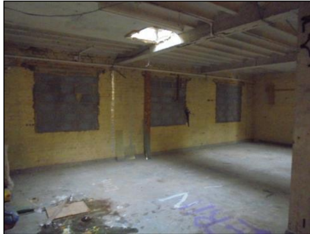
Photo 6: Interior view of the second floor south-west corner of the warehouse building, from the north-east
