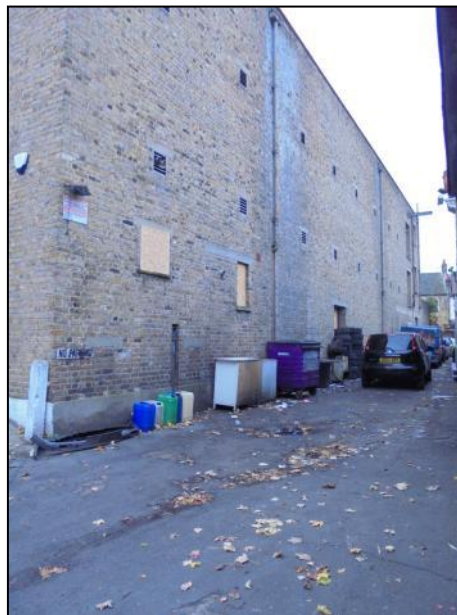
Photo 5: View of the northern side of the warehouse building, from the east
