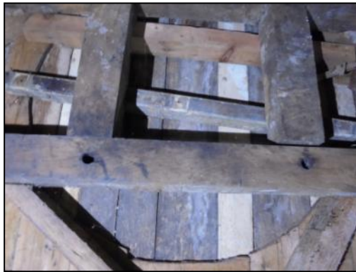
Photo 6: Circular hole at the top of the frame
