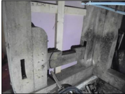
Photo 5: Horizontal mechanism of timber framed structure, behind modern partition wall within Building 2
