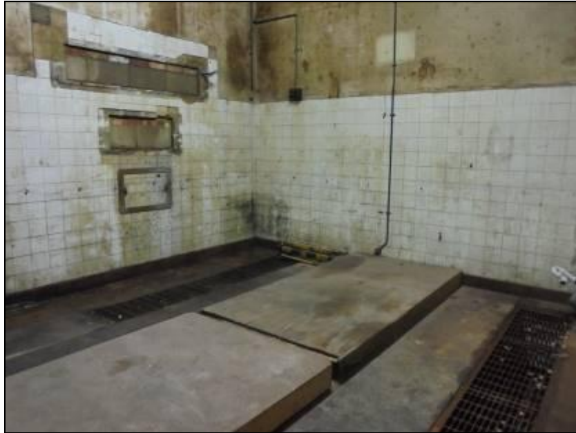
Photo 3: The work space in the rear (north) of the brick structure at the site, showing the covered inspection pit in the centre, and the linear drains either side
