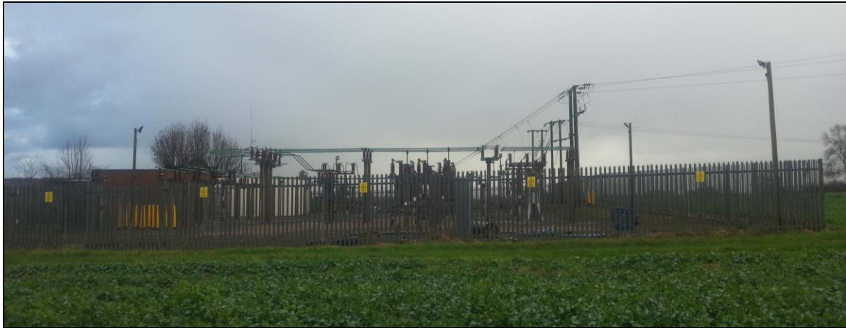
Plate 1 Electricity Substation taken at the north of the site facing east
