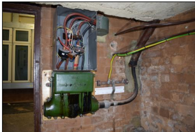
Photo 7: Former electricity connection box, at basement level
