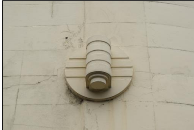
Photo 4: One of two exterior uplight on the western elevation
