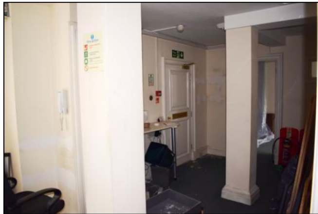
Photo 6: Cast concrete columns and beams in the reception area. Wall inspected is immediately to the right of the columns
