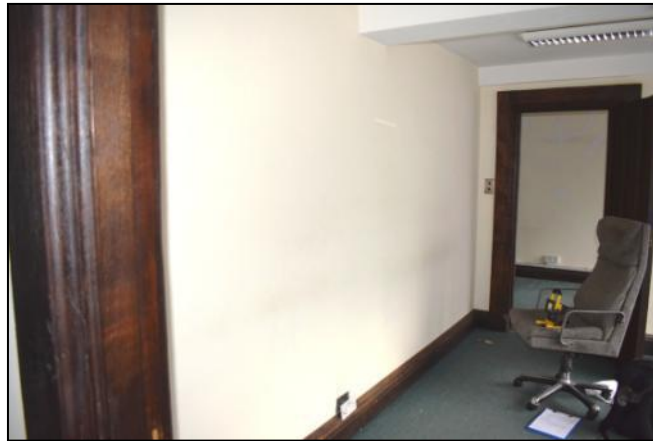
Photo 5: The inspected interior wall with cast concrete beams visible in the ceiling
