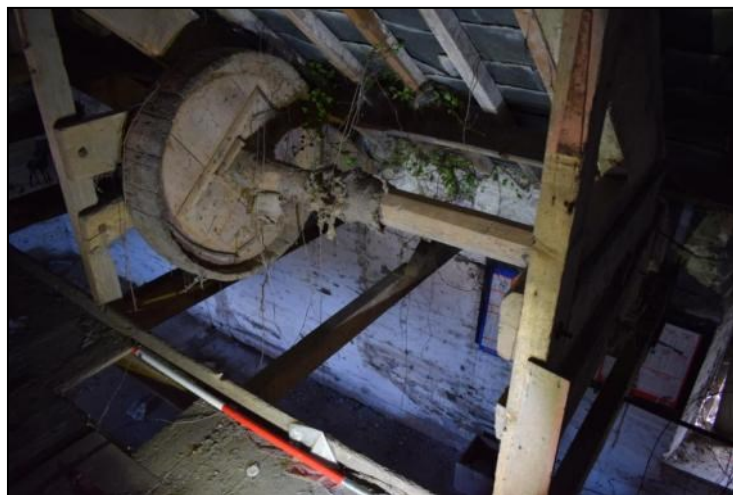
Photo 12: Sack hoist drive wheel & chain drum in the second floor loft. Scale 1m
