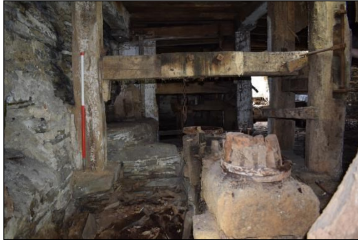
Photo 8: View of the interior of the hurst from the north pit wheel pit. Scale 1m
