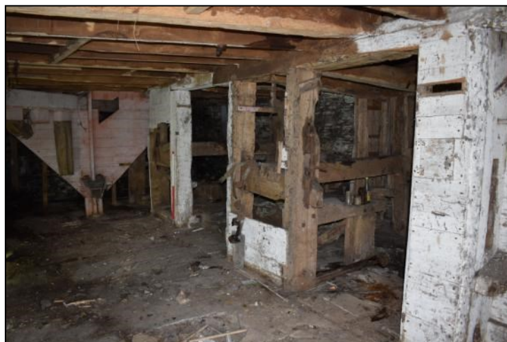
Photo 7: Eastern end of the ground floor with hurst and hopper. Scale 1m
