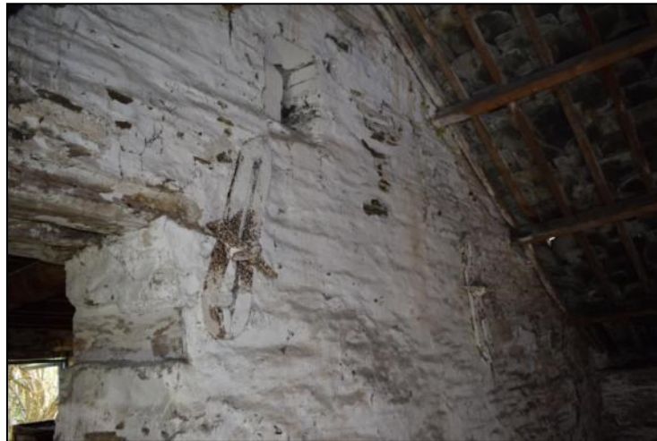
Photo 11: Details of the former west facing exterior wall of the mill at first floor level
