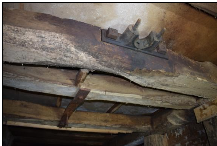
Photo 9: Stone beams & vertical bearing on bridge beam above northern wheel pit wheel on the ground floor
