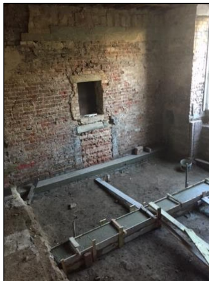
Photo 12: Blocked chimney (centre) & flue (top left) and raised ceiling height (top) during redevelopment works (Building Logistics Ltd)
