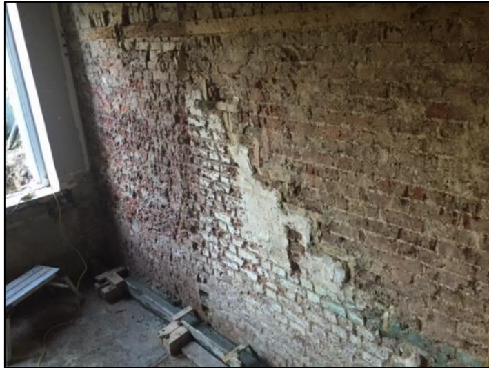
Photo 13: Scar of former staircase and wall plate during the redevelopment works (Building Logistics Ltd)
