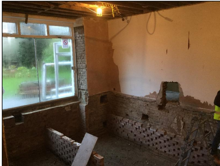
Photo 10: Raised floor level in the lower ground floor during redevelopment works (Building Logistics Ltd)
