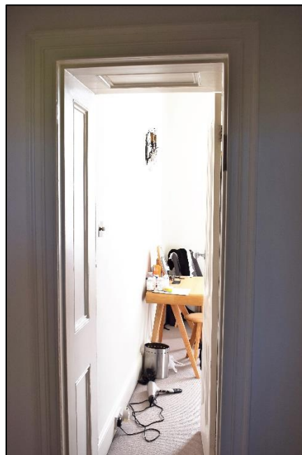
Photo 16: Reduced width doorframe in first floor flat
