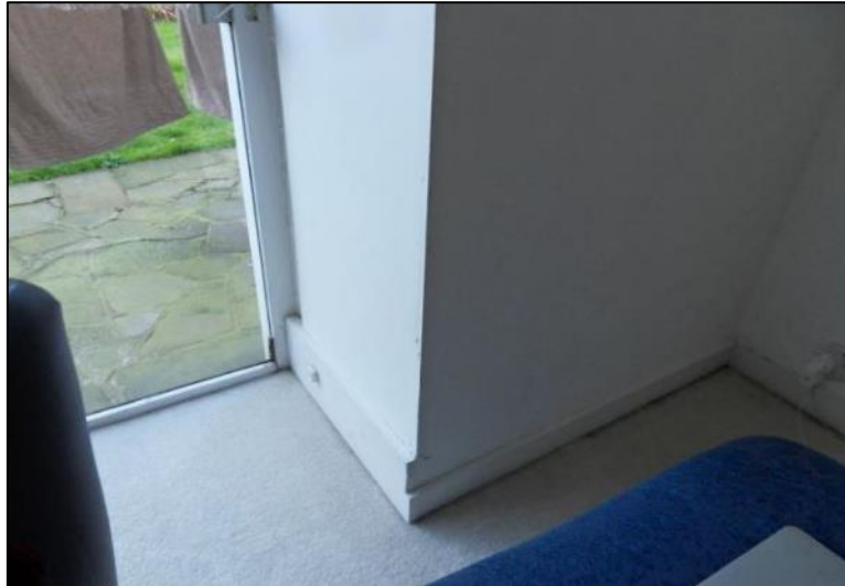
Photo 8: Skirting board in the living room of 84b (Gemini Building & Design Consultancy)
