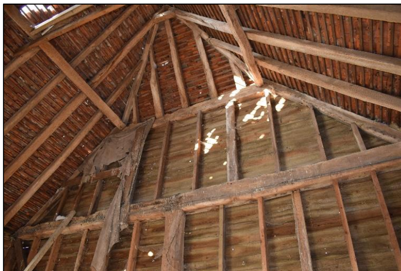
Photo 11: Details of the roof structure at the western end of the barn
