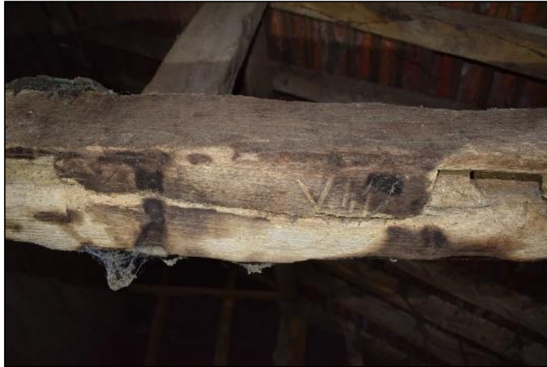
Photo 18: Carpenters mark and burn marks on a timber in the catslide extension
