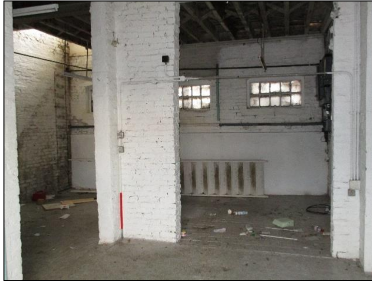
Photo 10: Surviving brick floor (rear) & concrete floors (foreground). Position of former staircase (rear left)
