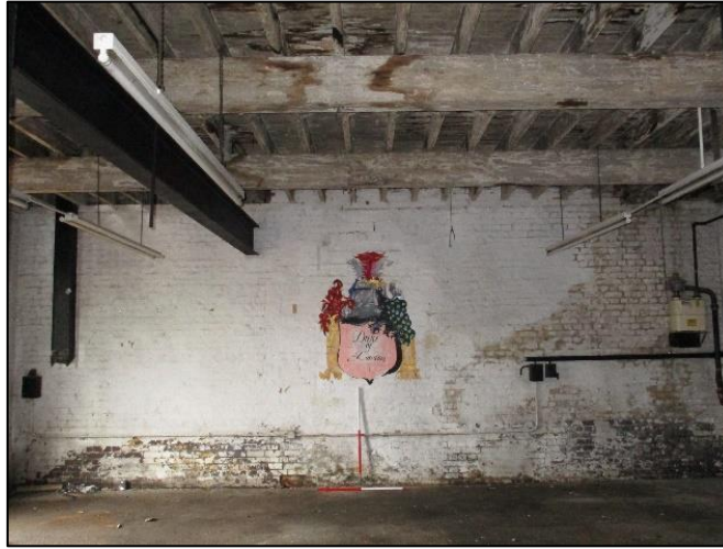
Photo 8: Blocked doorway in the south-east end of the building (in location mural) & example of the stripped-out interior
