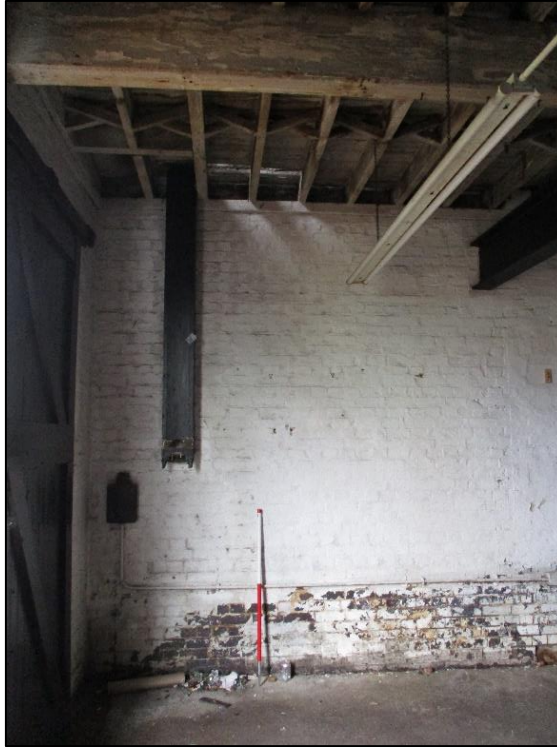
Photo 12: Shoot from first-floor level and additional bracing of the first-floor floor boards
