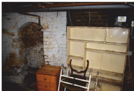
Photo 14: Base of the chimney and blocked doorway (behind the built-in shelves, right) in the rear basement
