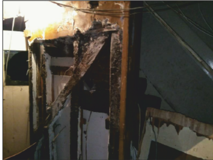
Photo 2. Staircase at ground floor. Shot shows side panel removed revealing timber behind. Note stair handrail on right of shot
