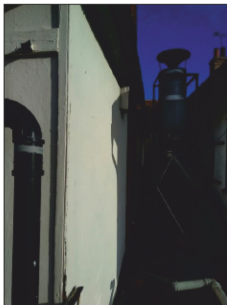
Photo 3. Looking at rear of building showing existing duct exit in south elevation
