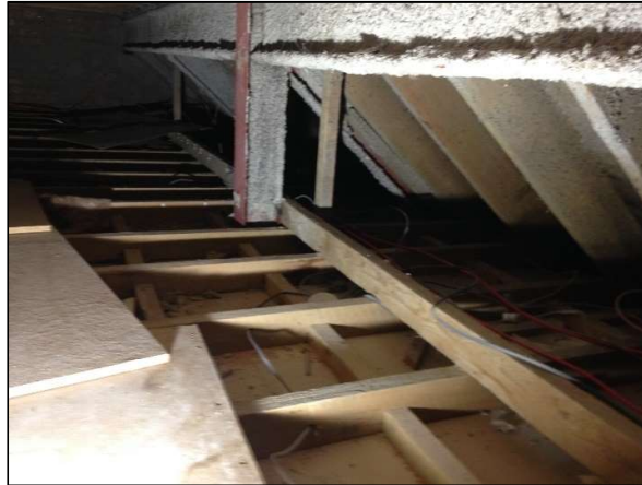
Photo 2: Roof interior, showing steel frame construction (courtesy of Jo Dyszlewicz; Design-London Ltd)
