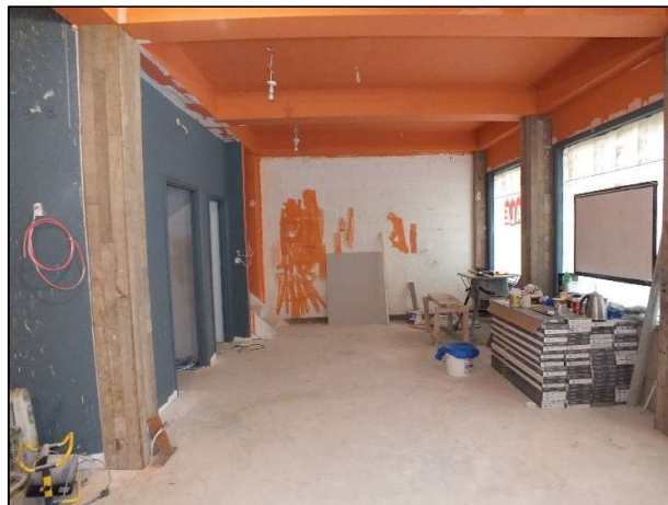
Photo 1: Interior of Unit 6 showing concrete floor and breeze block walls, looking east
