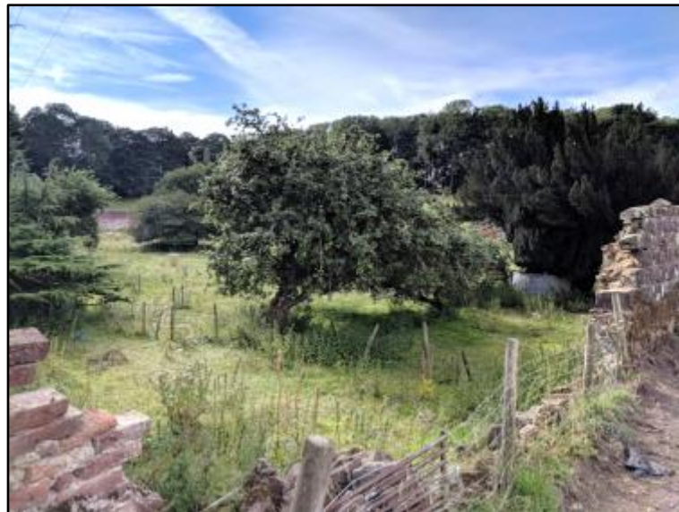
Photo 4. Damaged wall at south-east corner, looking north-west into site
