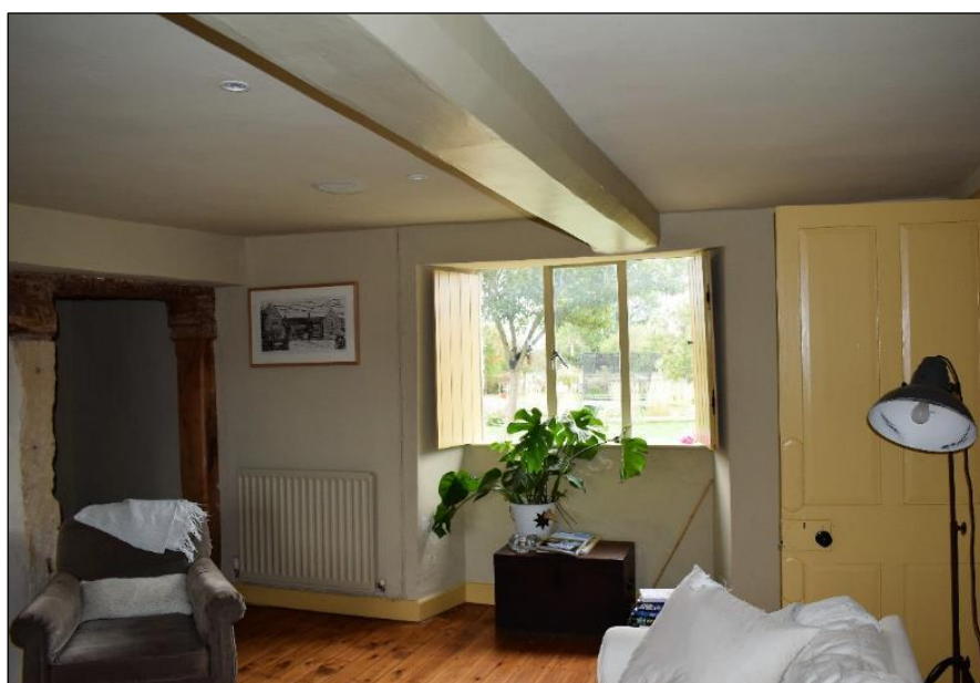
Photo 6: Oddly placed beam in the sitting room
