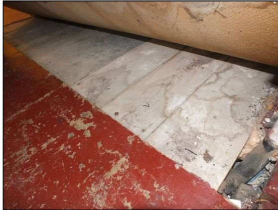
Photo 6. Floorboards at the top of the steps in the lobby
