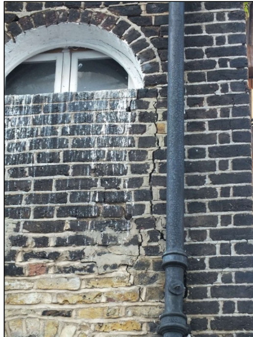
Photo 4. Close up of cracks in brickwork on rear elevation
