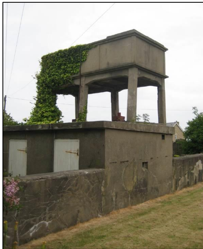
Photo 17: The boundary wall and water tower of Roberts Battery from the garden of Beresford Lodge
