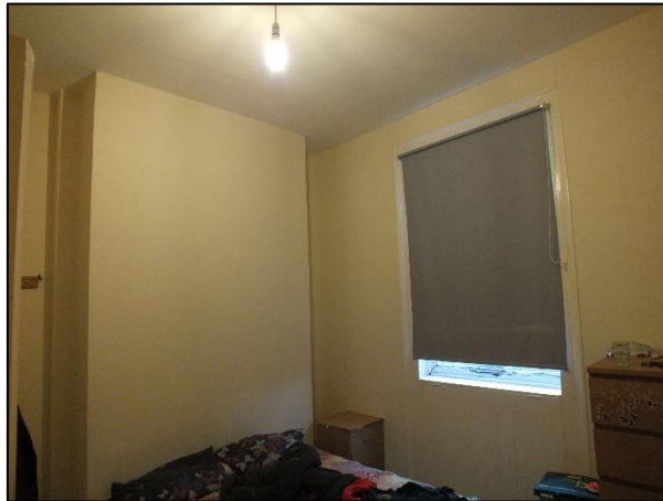
Photo 5. Rear bedroom with blocked fireplace and timber panel below window
