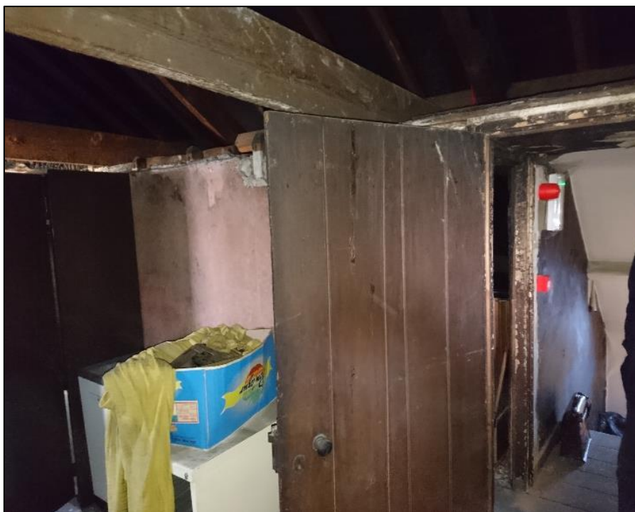
Photo 1. Showing demolished ceiling at front attic room. Note the door which may be original
