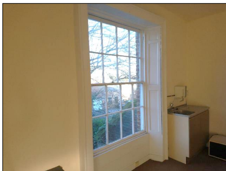
Photo 3. Showing rear window at first floor. Original panelled architrave but replacement sashes
