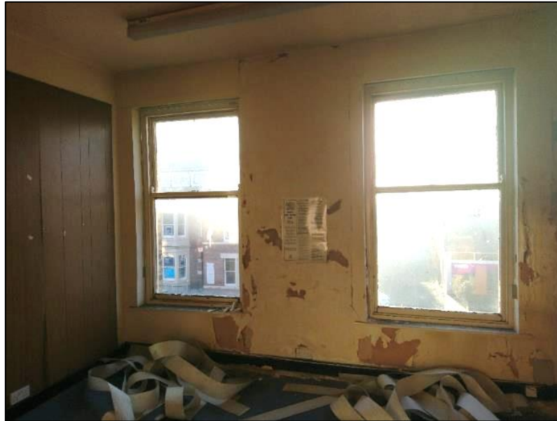
Photo 4. Showing mid and west windows at first floor. Note the strip light on the ceiling
