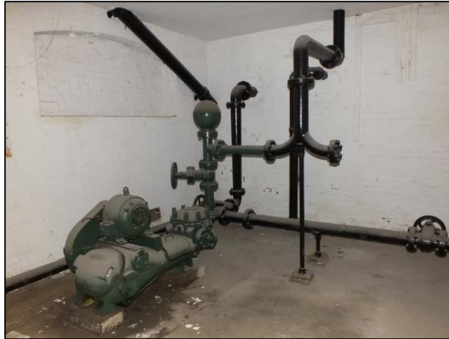
Photo 12. Pump in basement below Generator Hall
