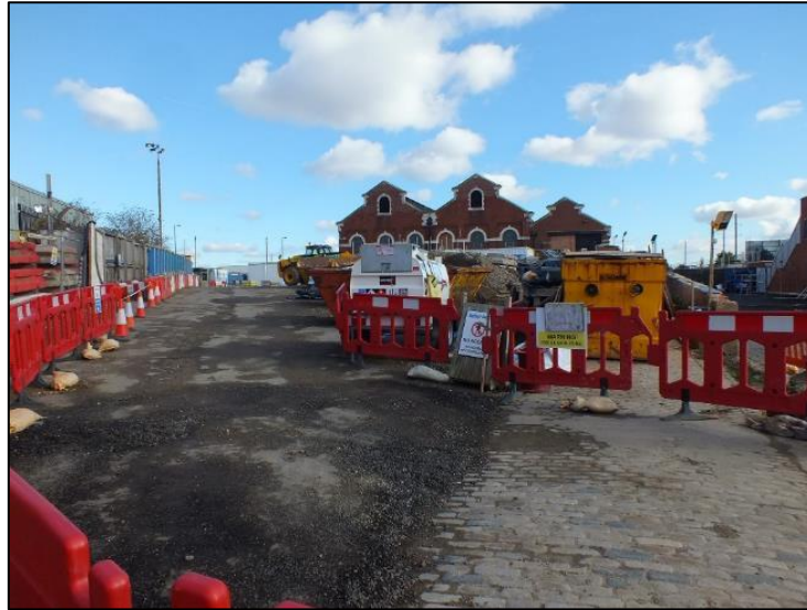
Photo 2. Western part of site, including cobbled ramp leading into the depot (direction: NE)
