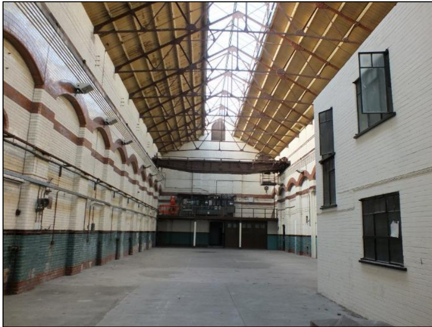
Photo 10. Interior of Generator Hall (direction W)
