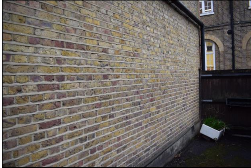
Photo 12: View of north facing external wall of former school building viewed from western courtyard area, looking southwest
