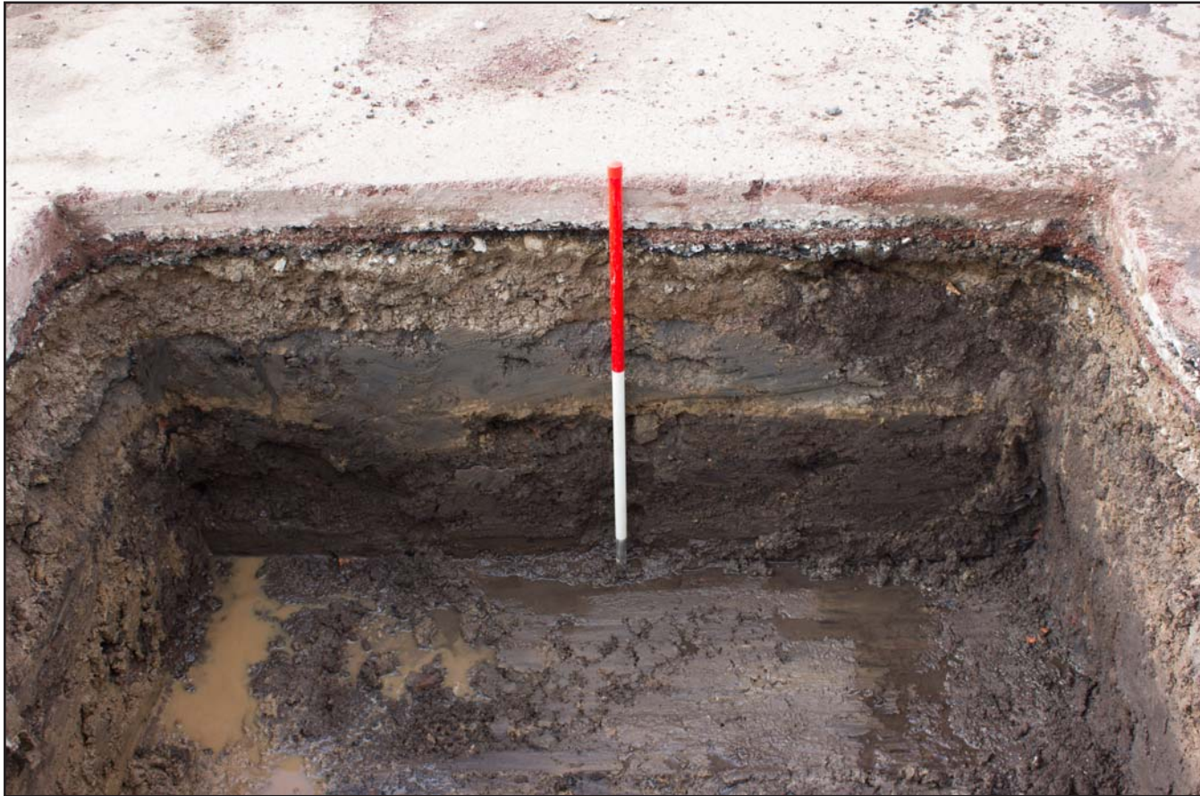
Plate 39: Parasol Base 10 for Parade Ring Canopies at Chester Racecourse, Chester - from the southeast - 1.00m scale
