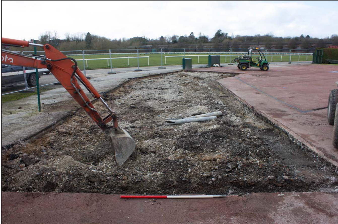
Plate 04: Post Tarmac removal Kitchen Pod foundations, Chester Racecourse, Chester - from the east - 1.00m scale
