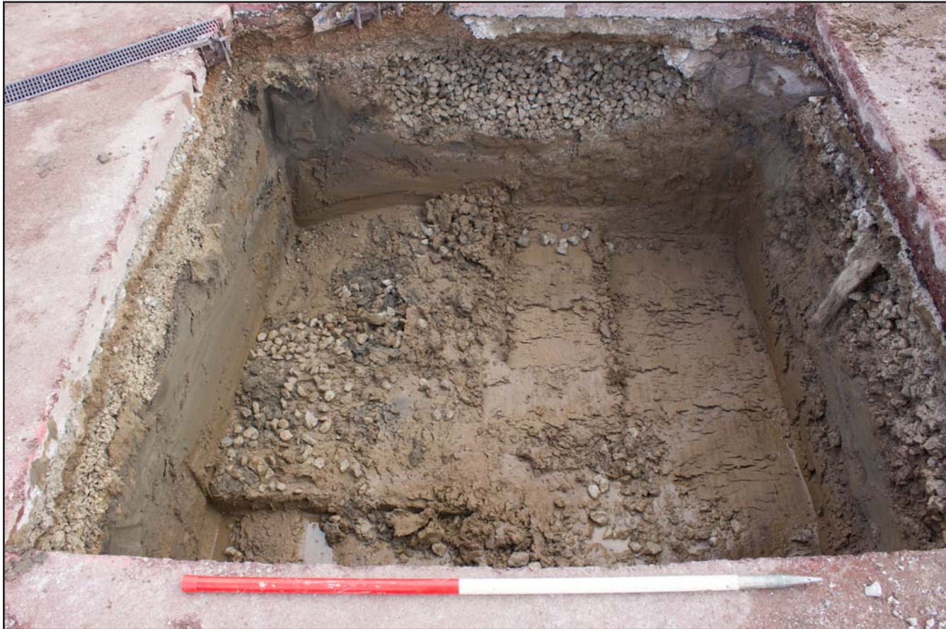
Plate 34: Parasol Base 8 for Parade Ring Canopies at Chester Racecourse, Chester - from the southwest - 1.00m scale
