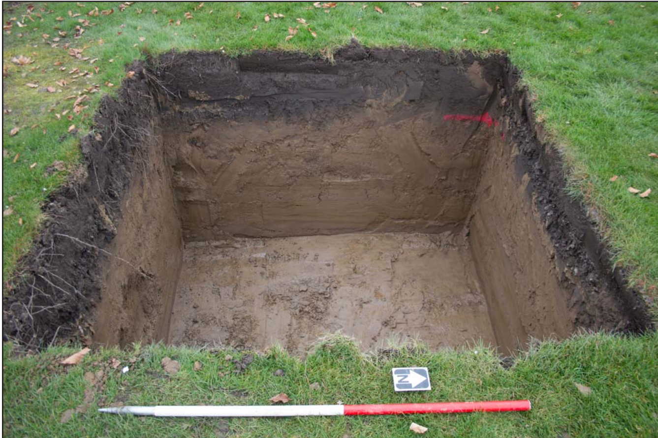
Plate 20: Parasol Base 1 for Parade Ring Canopies at Chester Racecourse, Chester - from the east - 1.00m scale
