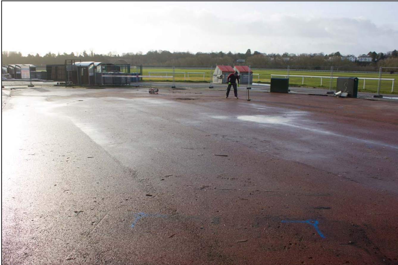
Plate 02: Pre excavation shot of foundations for Kitchen Pod, Chester Racecourse, Chester - from the north - no scale
