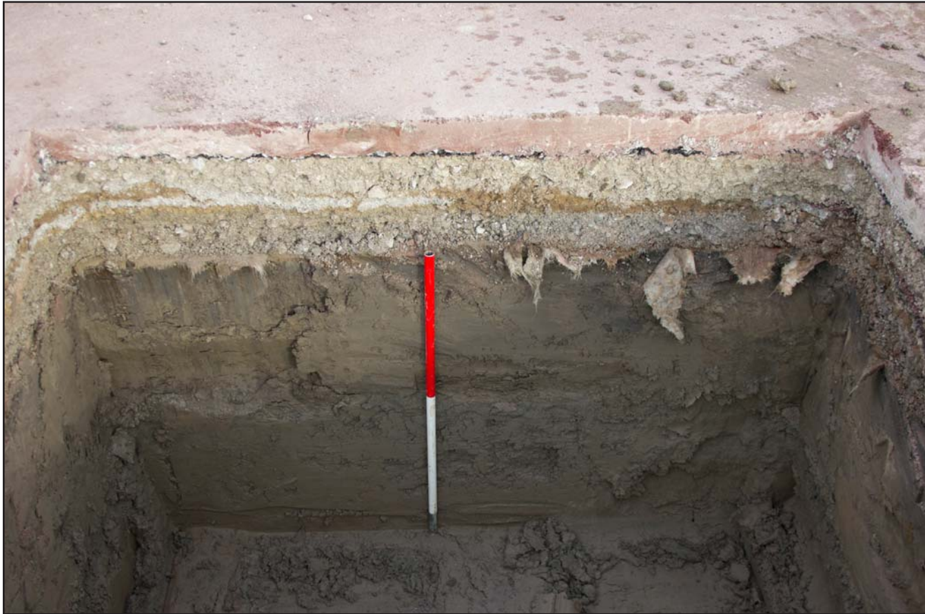
Plate 33: Parasol Base 7 for Parade Ring Canopies at Chester Racecourse, Chester - from the west - 1.00m scale
