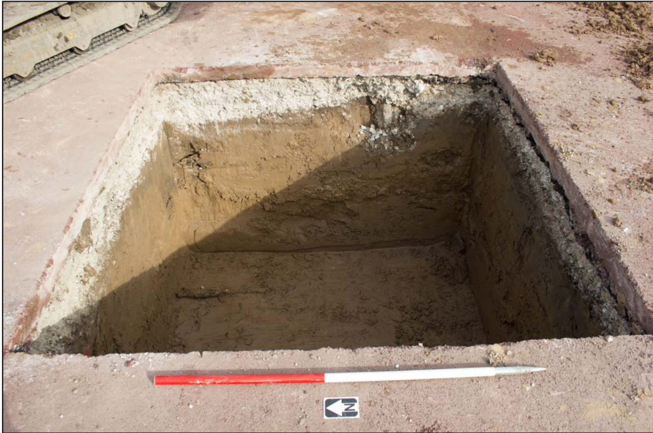
Plate 30: Parasol Base 6 for Parade Ring Canopies at Chester Racecourse, Chester - from the west - 1.00m scale
