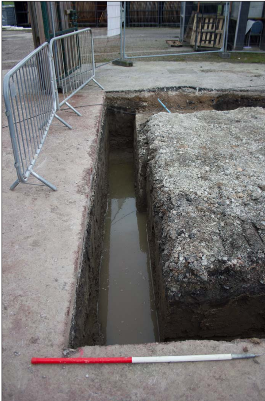
Plate 14: Trench C within foundations for Kitchen Pod, Chester Racecourse, Chester - from the south - 1.00m scale
