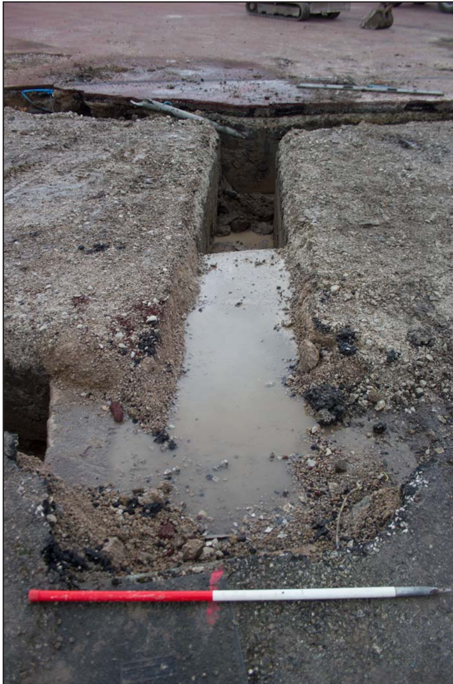
Plate 17: Trench F within foundations for Kitchen Pod, Chester Racecourse, Chester - from the south - 1.00m scale
