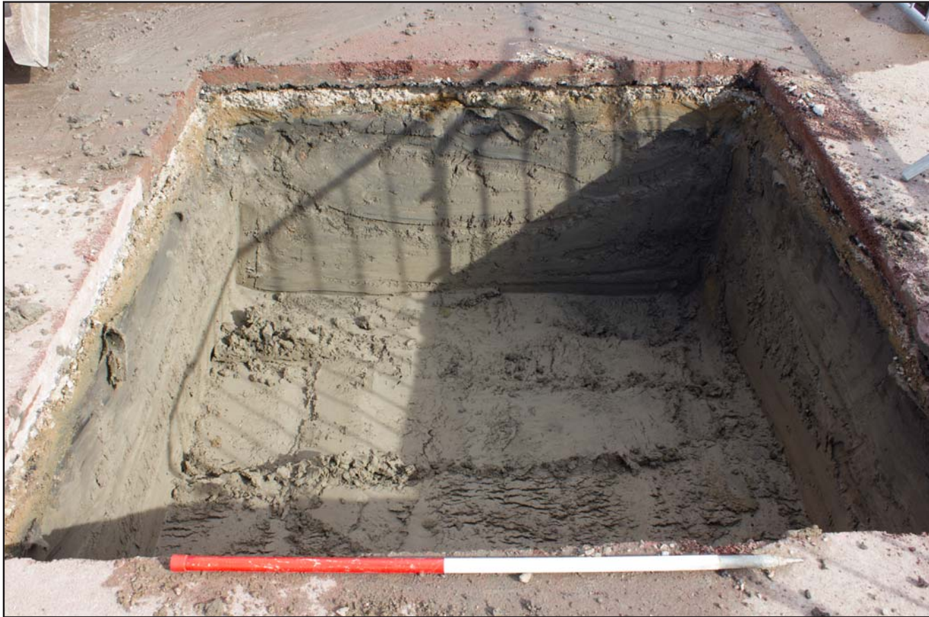
Plate 44: Parasol Base 13 for Parade Ring Canopies at Chester Racecourse, Chester - from the southwest - 1.00m scale
