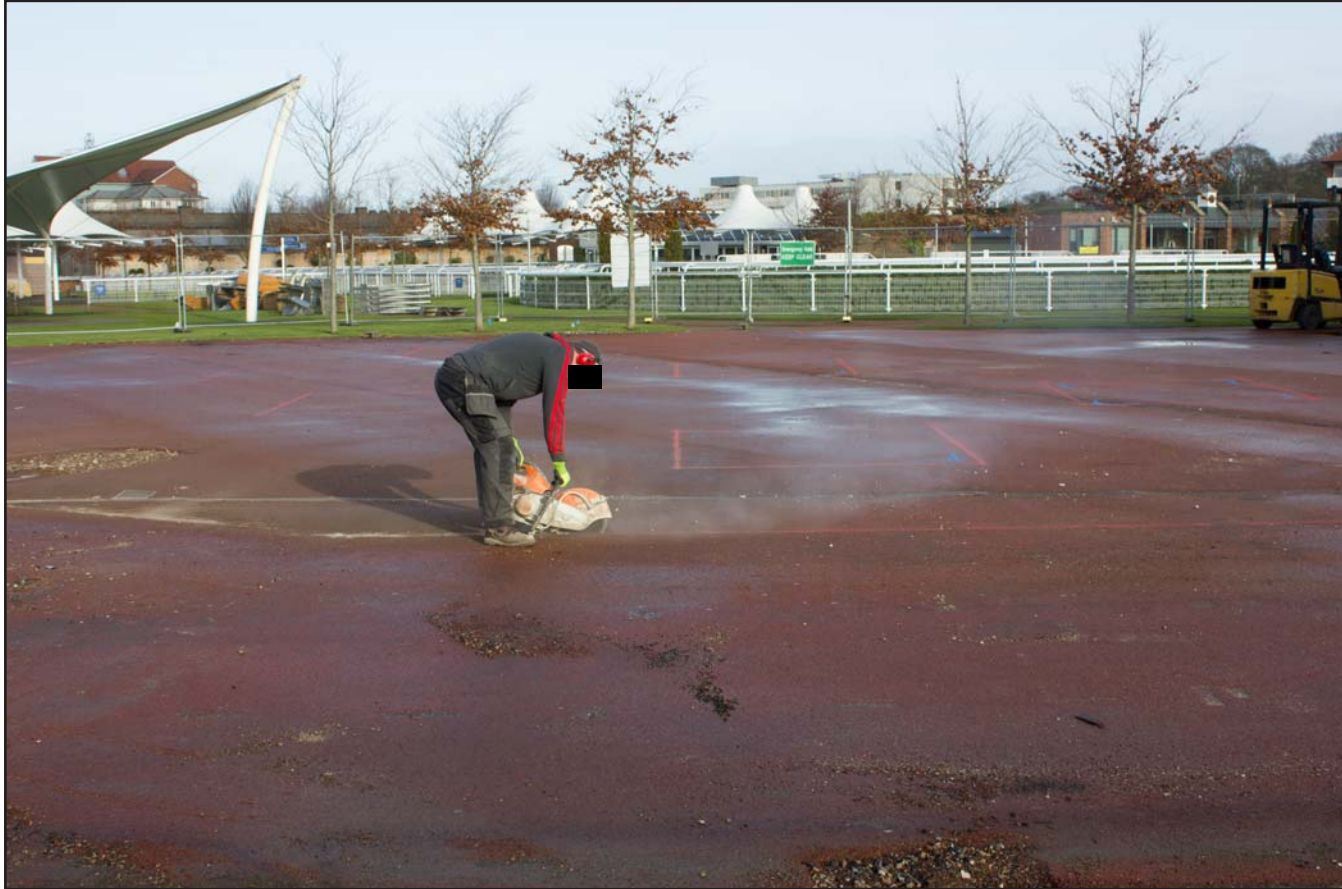
Plate 03: Working Shot cutting Tarmac, Chester Racecourse, Chester - from the south - no scale
