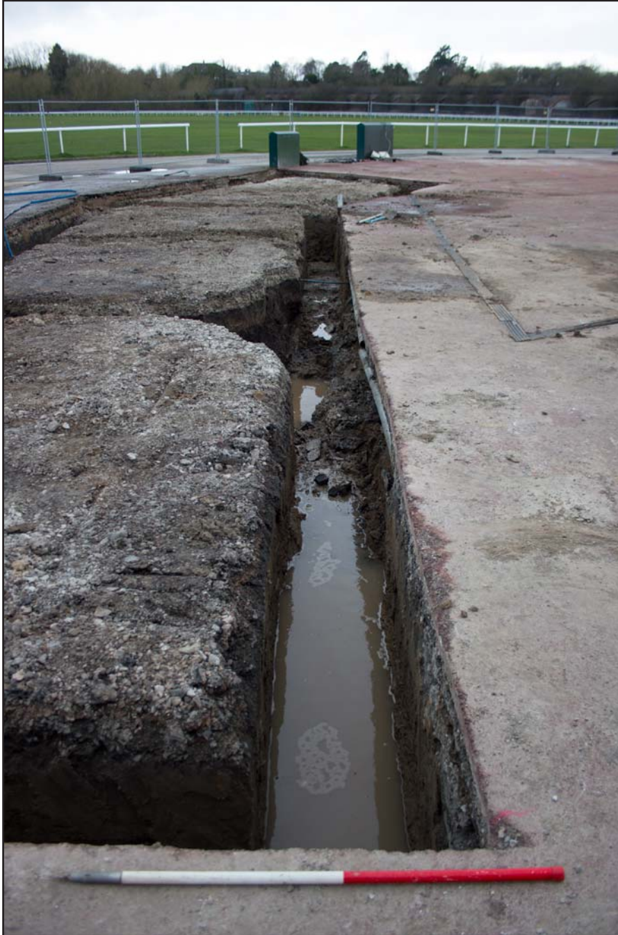
Plate 12: Trench A within foundations for Kitchen Pod, Chester Racecourse, Chester - from the south - 1.00m scale
