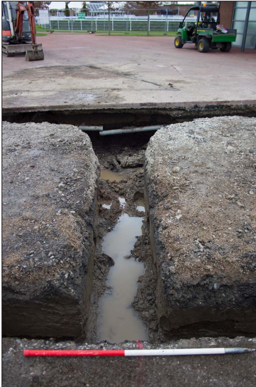
Plate 15: Trench D within foundations for Kitchen Pod, Chester Racecourse, Chester - from the south - 1.00m scale
