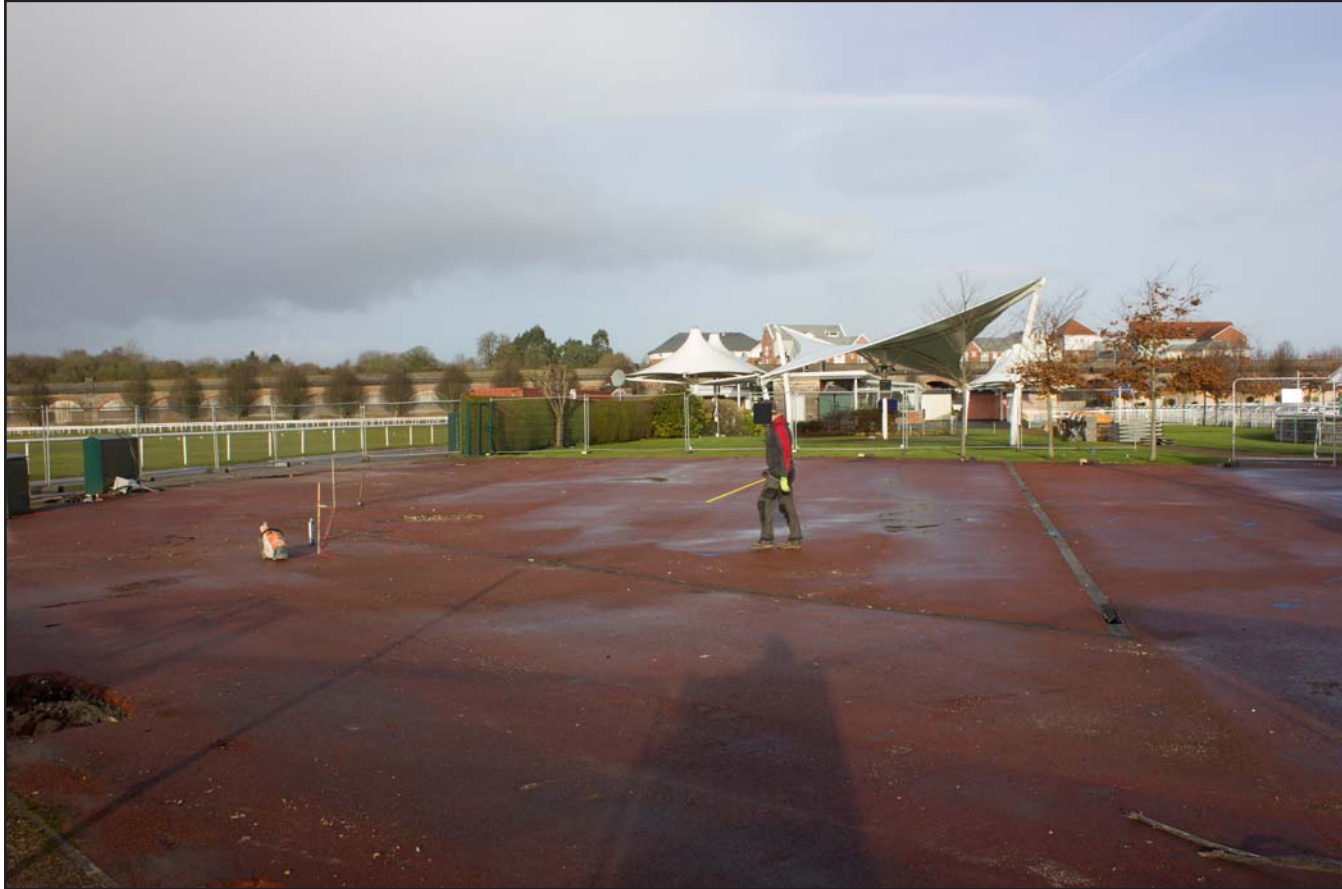
Plate 01: Pre excavation shot of foundations for Kitchen Pod, Chester Racecourse, Chester - from the south - no scale
