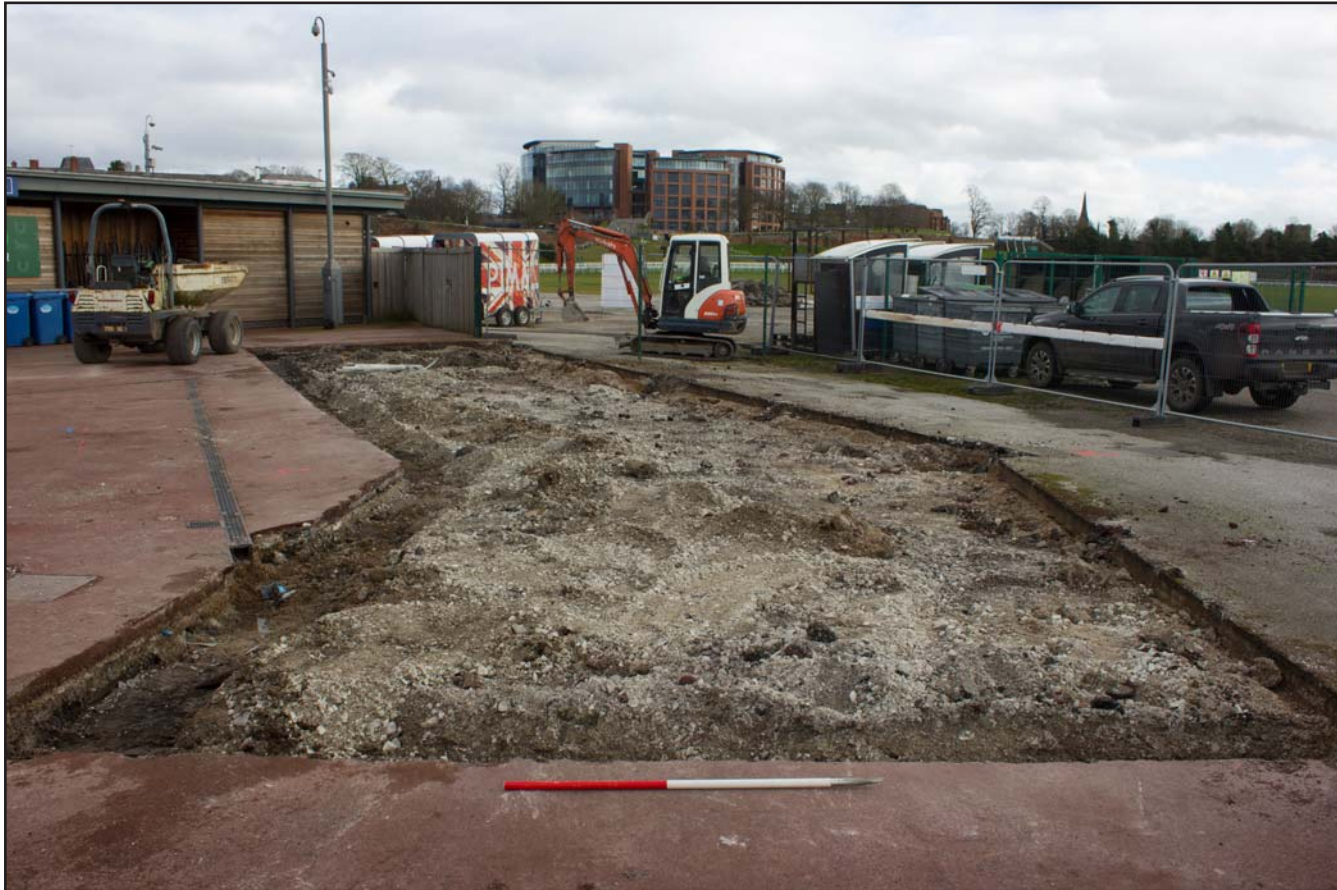
Plate 05: Post Tarmac removal Kitchen Pod foundations, Chester Racecourse, Chester - from the northwest - 1.00m scale
