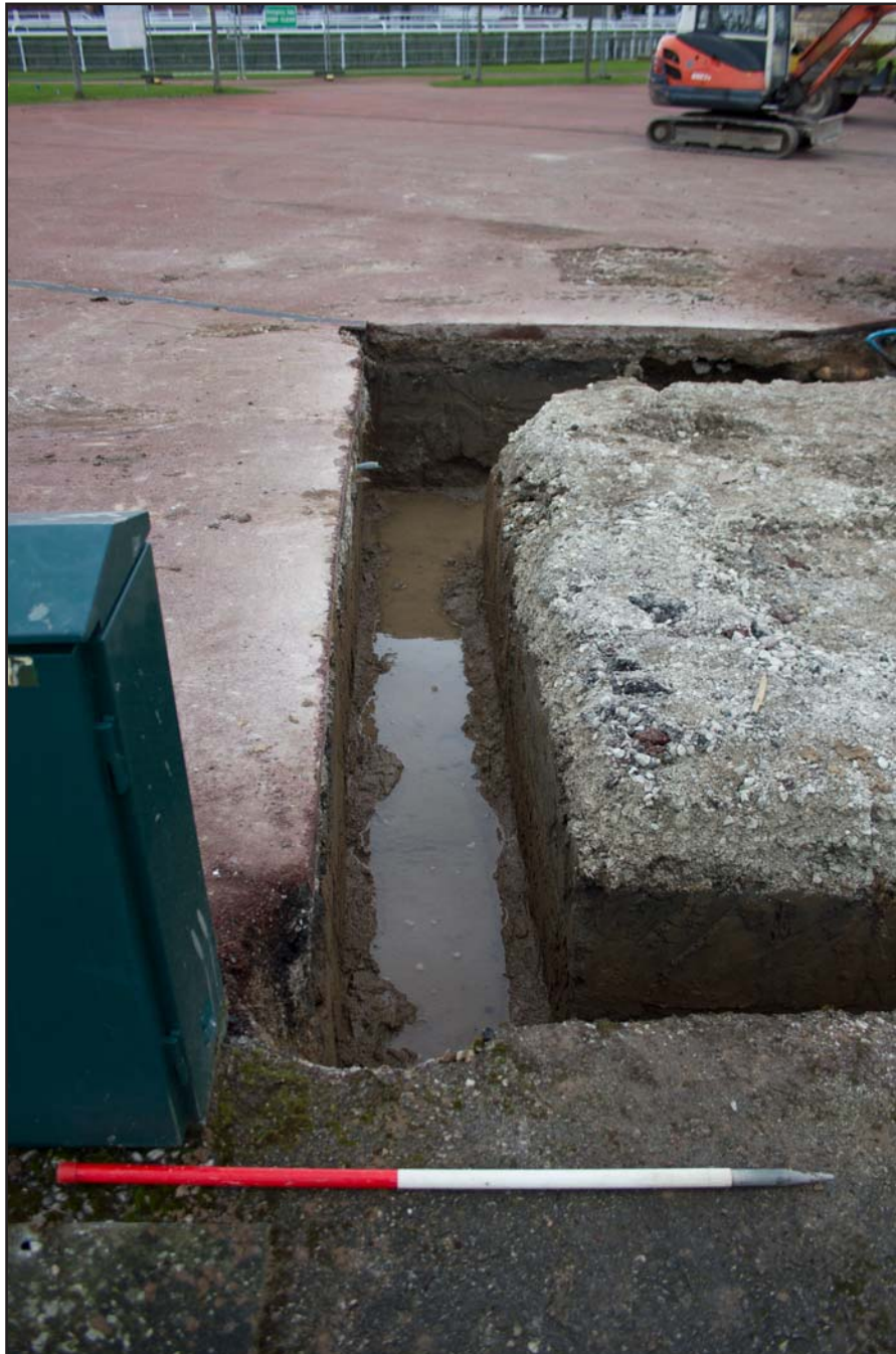
Plate 18: Trench G within foundations for Kitchen Pod, Chester Racecourse, Chester - from the south - 1.00m scale
