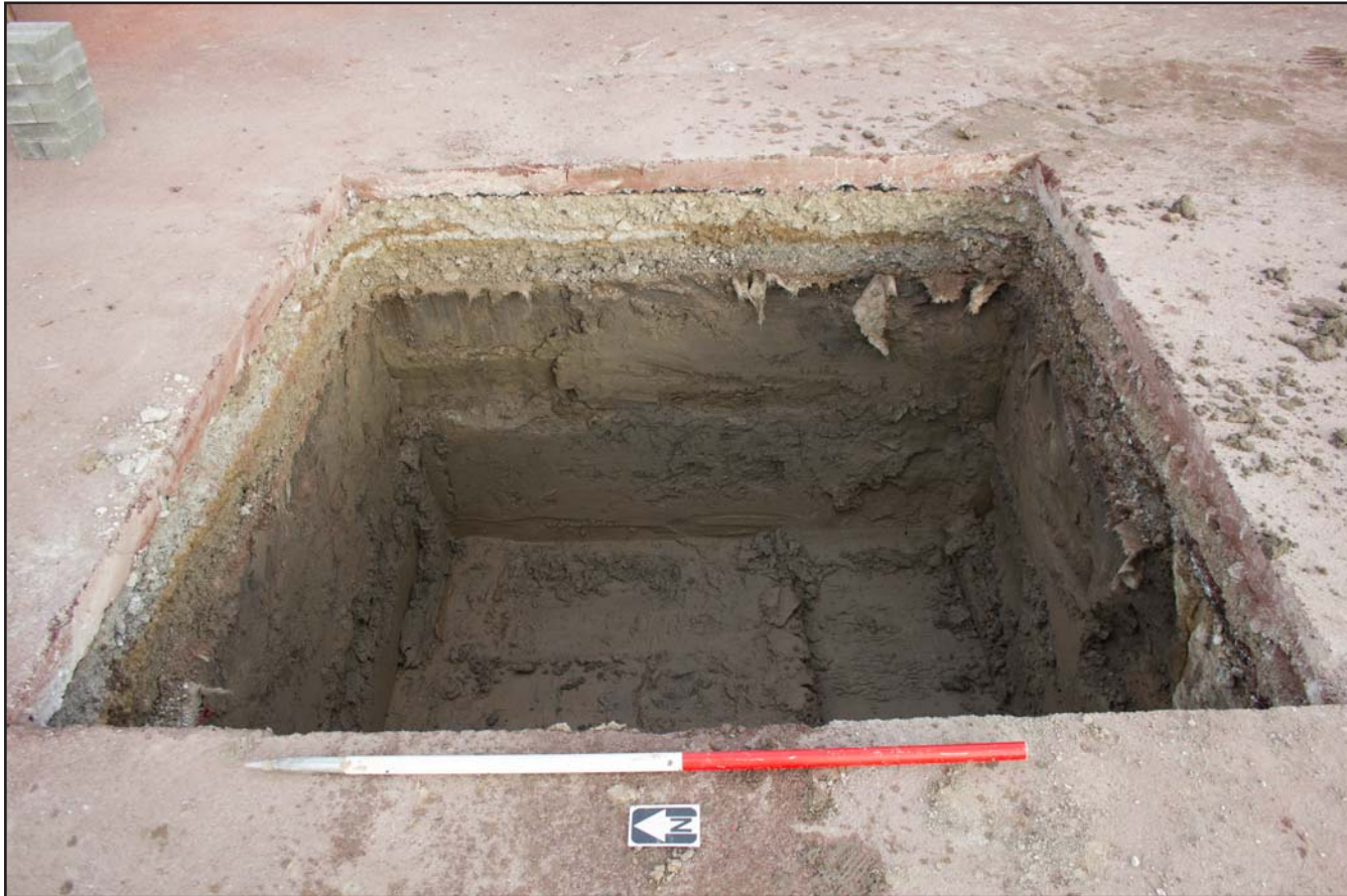
Plate 32: Parabol Base 7 for Parade Ring Canopies at Chester Racecourse, Chester - from the west - 1.00m scale
