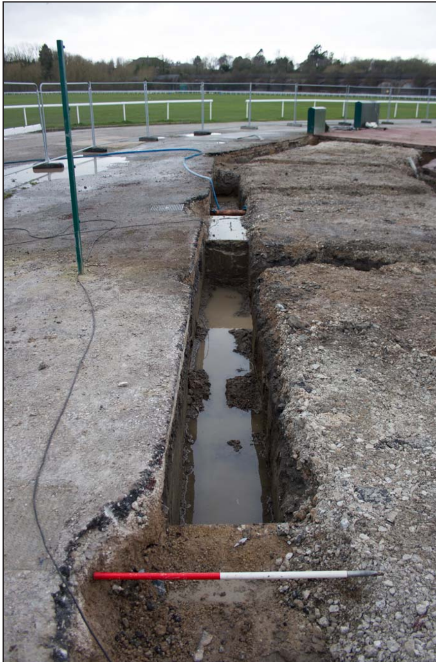
Plate 13: Trench B within foundations for Kitchen Pod, Chester Racecourse, Chester - from the south - 1.00m scale
