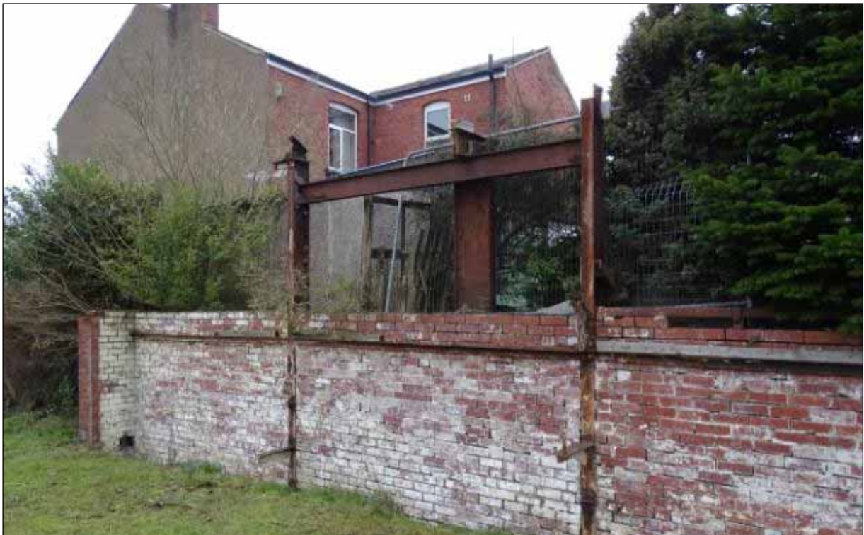
Plate 14: detail of brick wall (laid in an eccentric bond apparently mixing Flemish Bond and Scottish Bond) and embedded rolled steel joist structure), presumably boundary to or wall of industrial building which once occupied this part of the Site (Trafalgar Works)
