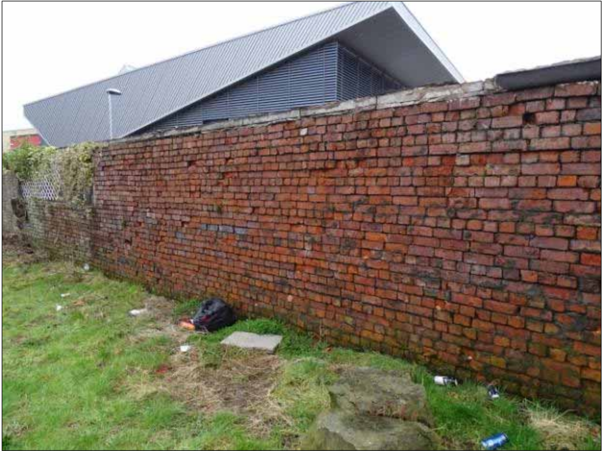
Plate 8: Brick wall forming western boundary to Site, laid to English Garden Wall bond
