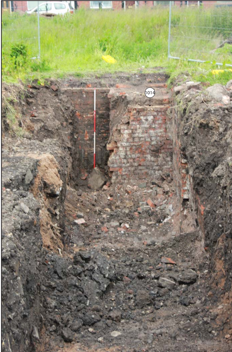
Plate 13: Trench 3 showing cellar foundations of Trafalgar Street Cotton Mill (1014), from the south-southeast. Scale 2.0m.
