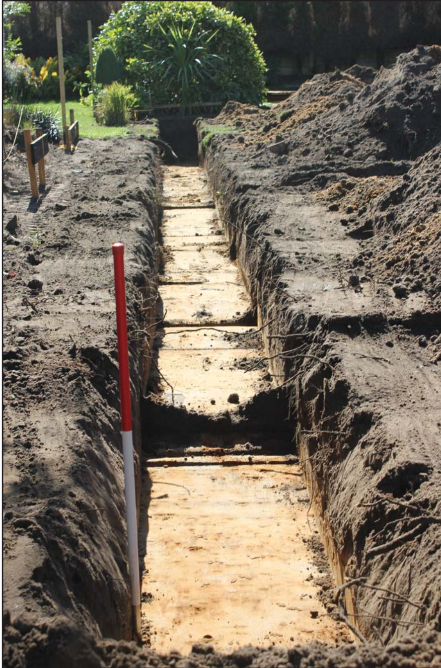
Plate 07: Trench Shot - to north of footings; easternmost trench - from North - Scale 1m
