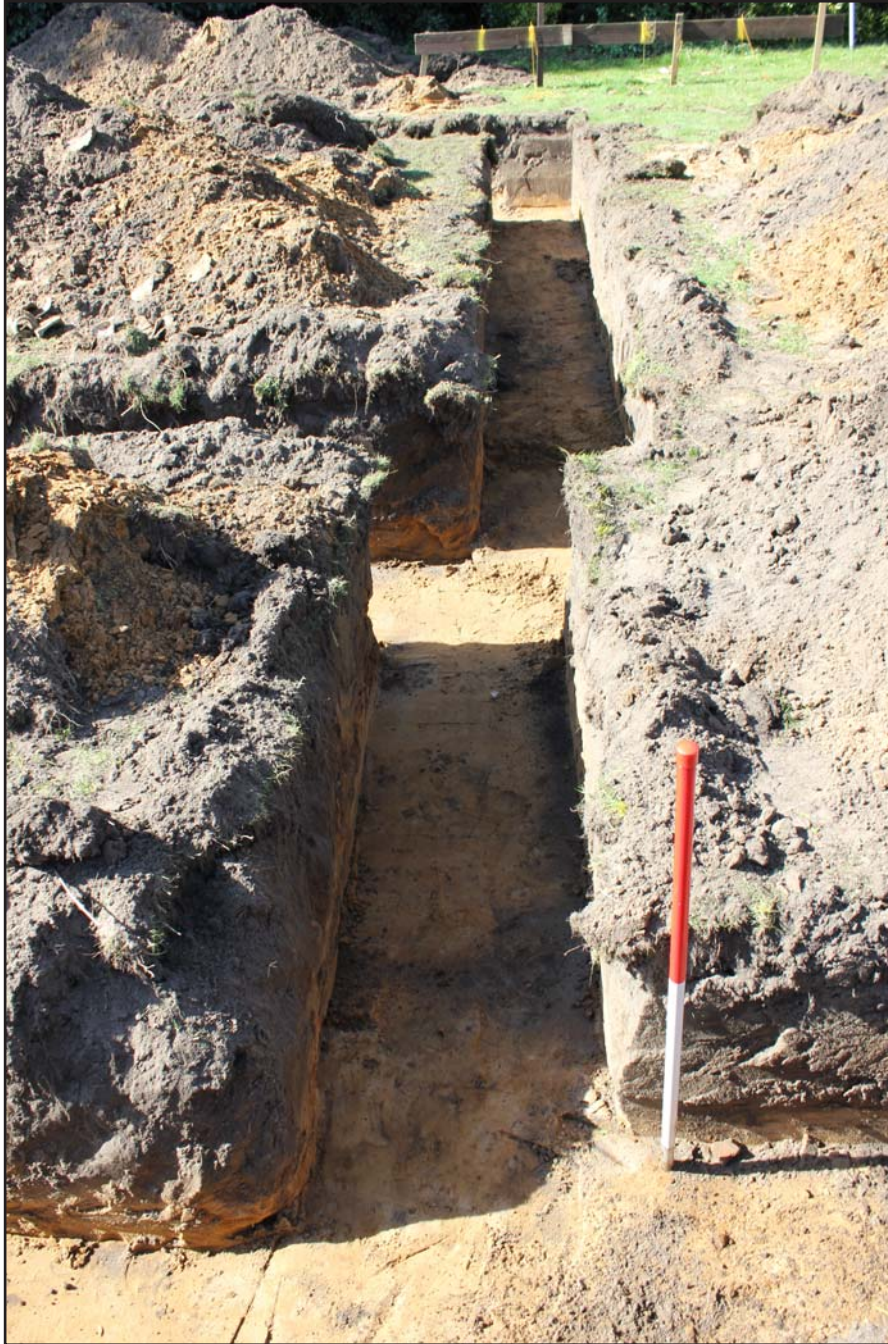
Plate 12: Trench Shot - to east of footings; east of pit feature - from East - Scale 1m
