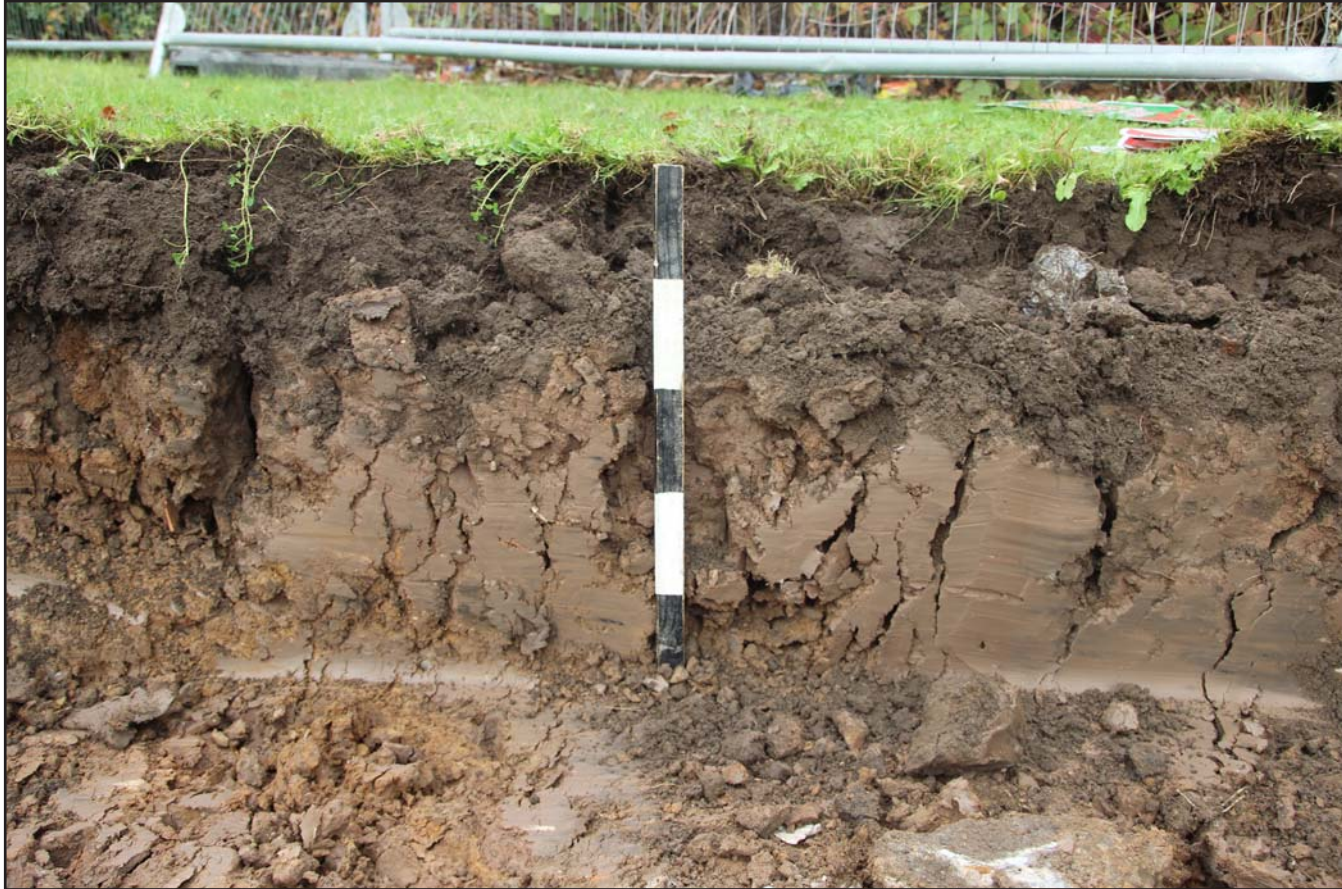
Plate 03: Generic section following excavation to full depth in south of site - from west -scale 0.5m
