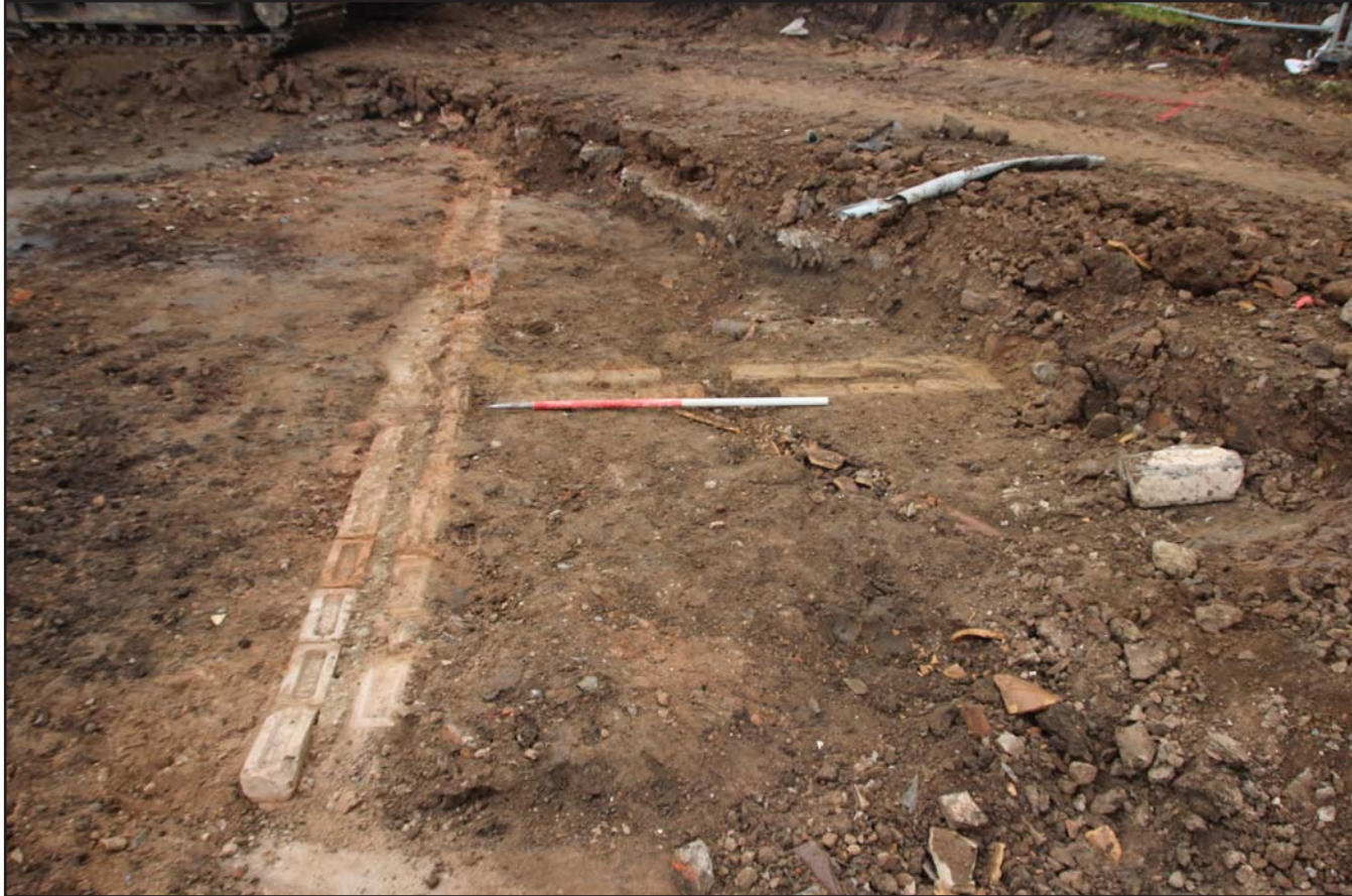
Plate 04: Brick wall and salt glaze pipes near eastern boundary - from southwest - scale 1m
