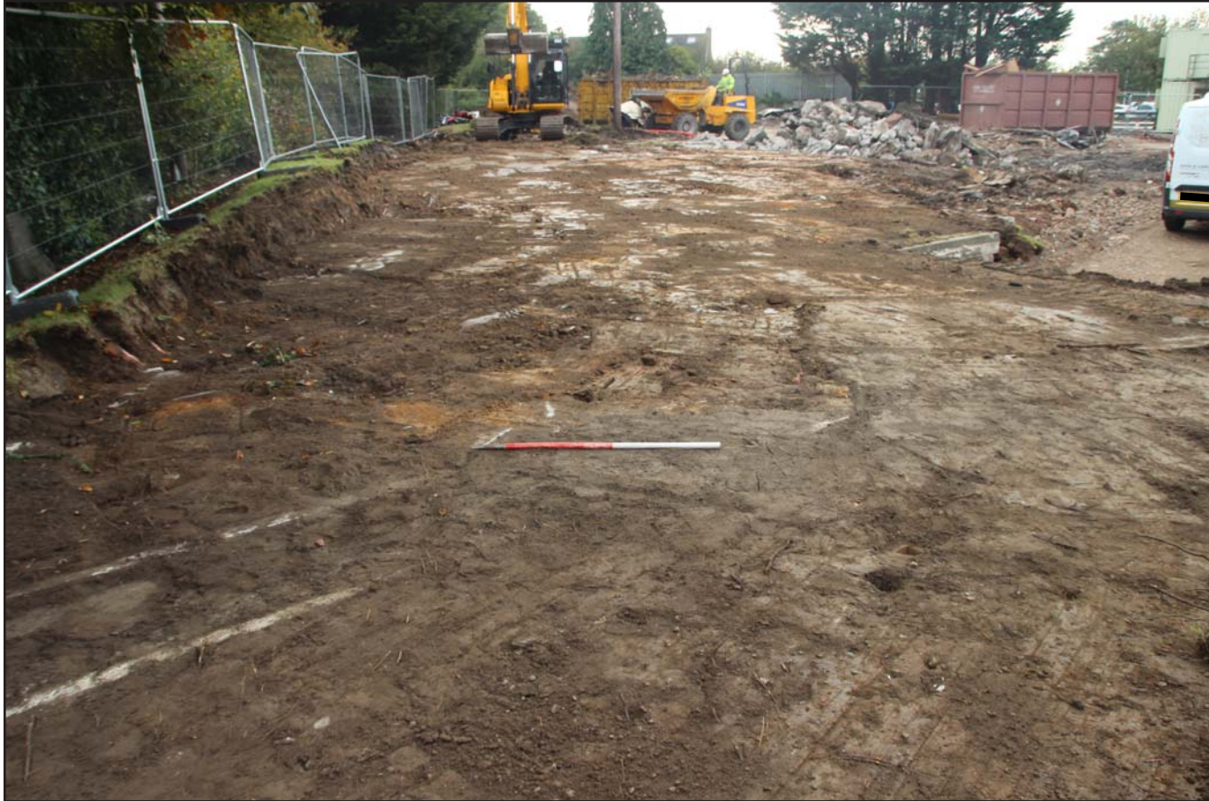
Plate 02: Post excavation shot of northern portion of site after topsoil strip - from north - scale 1m
