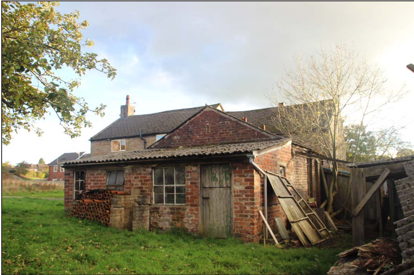
Plate 09: North and west facing outbuilding external elevations, from the northwest. Scale 1.0m.
