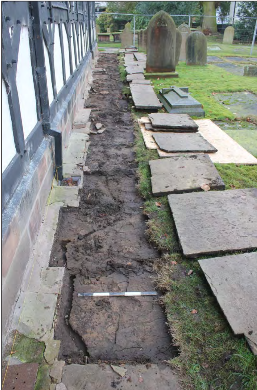
Plate 24: Pathway along northern elevation of St. Oswald's Church following removal of grave markers - from east - 0.5m scale
