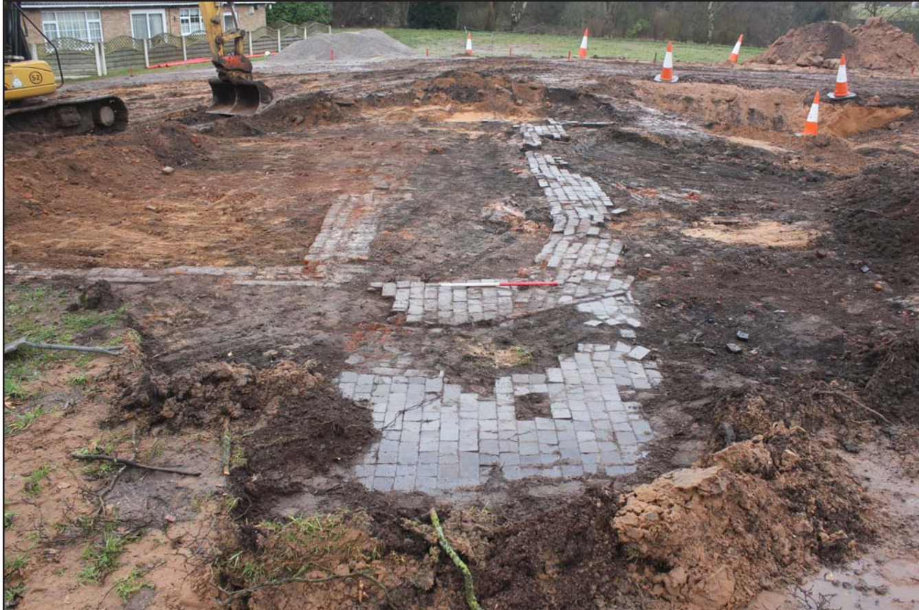
Plate 04: Plan shot showing brick floor surface (1007) in foreground, brick foundation wall (1004) to left and pathway (1005) to right - scale 1m
