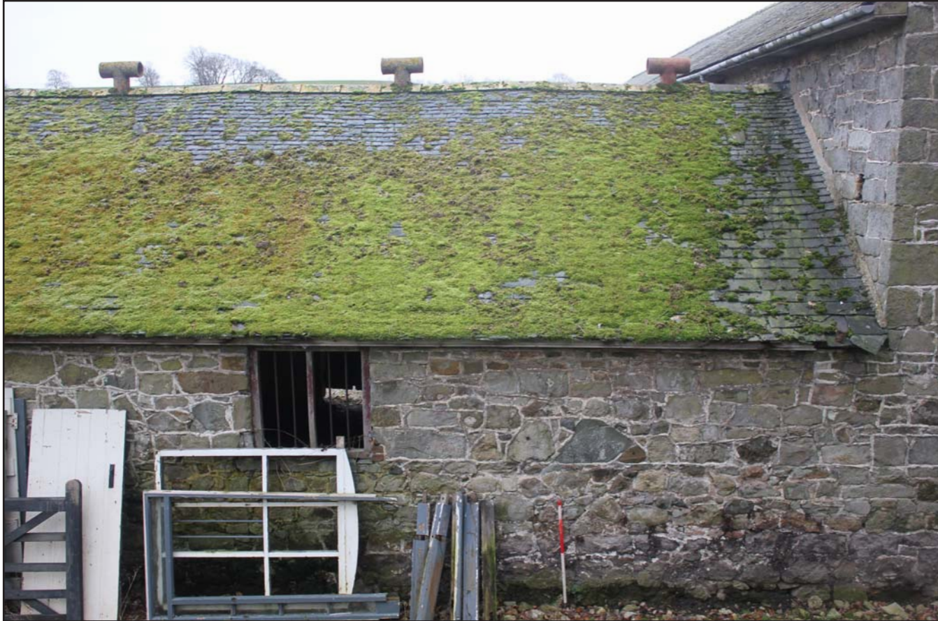
Plate 16: Llwyn y Maen, Oswestry, Shropshire. North-western range, northwest elevation right hand end - From the north-west - scale at 1m
