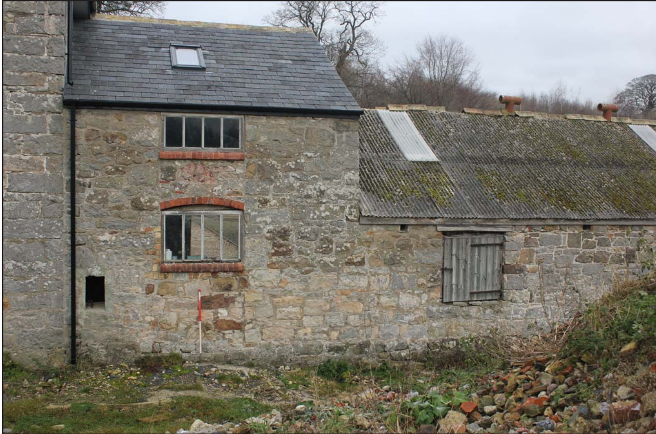
Plate 05: Llwyn y Maen, Oswestry, Shropshire. South-eastern range, south-east elevation (Room 4 - Mill Room) - From the south-east - scale at 1m
