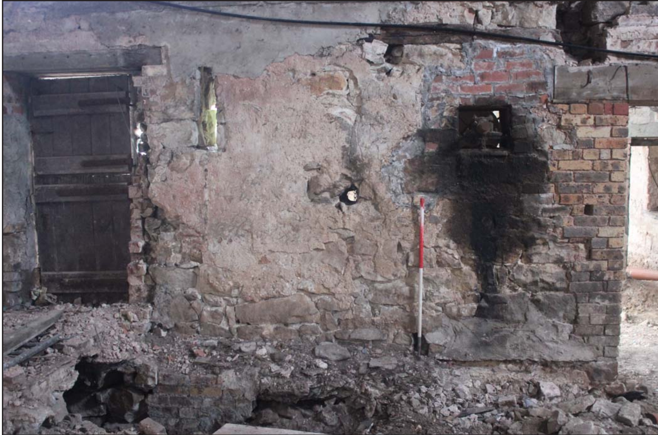
Plate 68: Room 5 - south eastern elevation showing linkage mechanism within wall (Room4 to right) - From the north-west - at 1m scale
