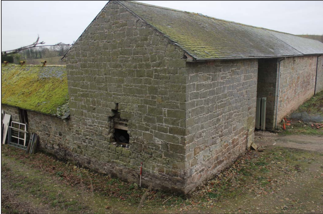
Plate 13: Llwyn y Maen, Oswestry, Shropshire. South-west and north-west elevations - From the west- scale at 1m
