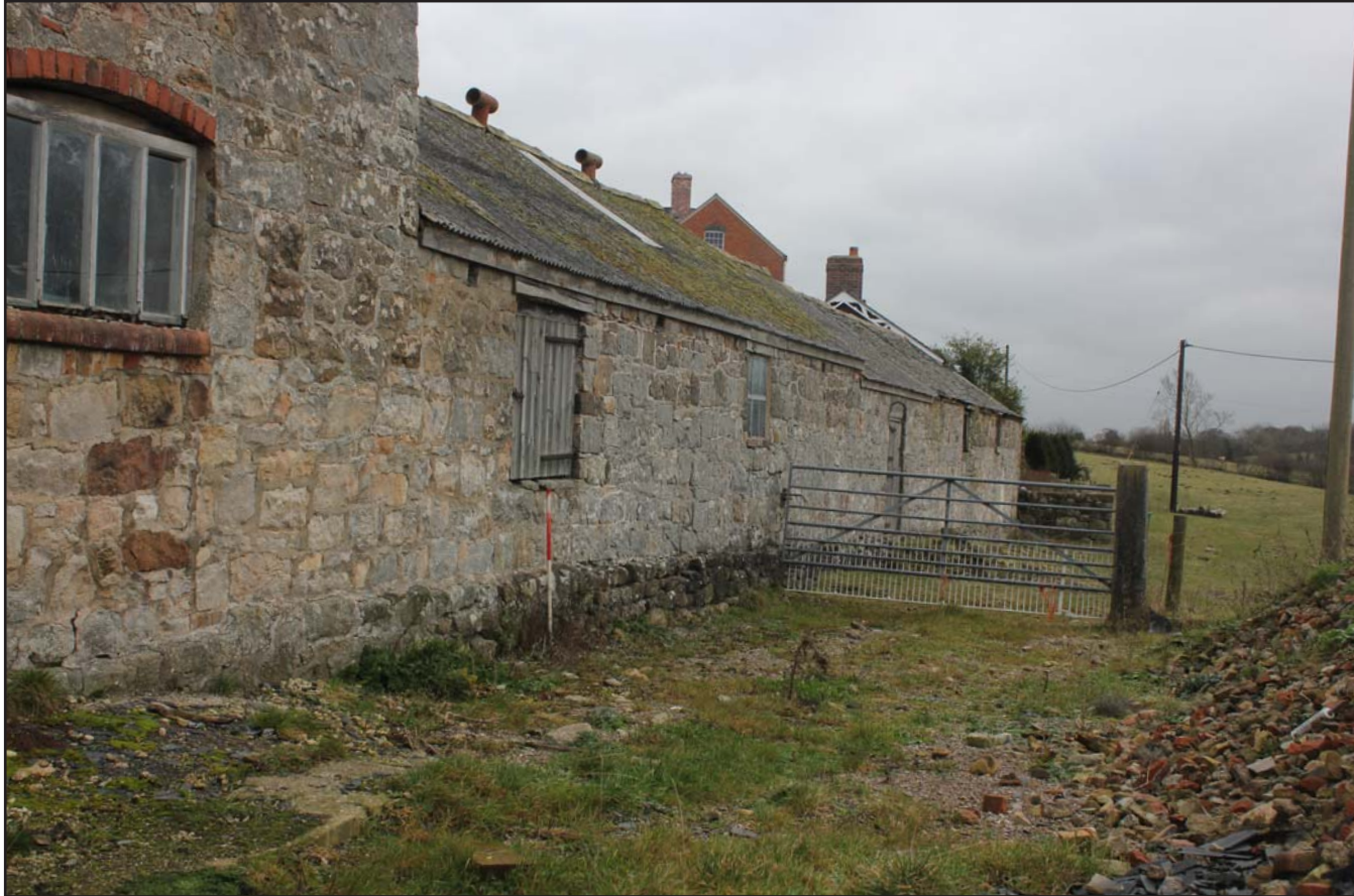
Plate 04: Llwyn y Maen, Oswestry, Shropshire. South-eastern range, south-east elevation central portion - From the south-east - scale at 1m
