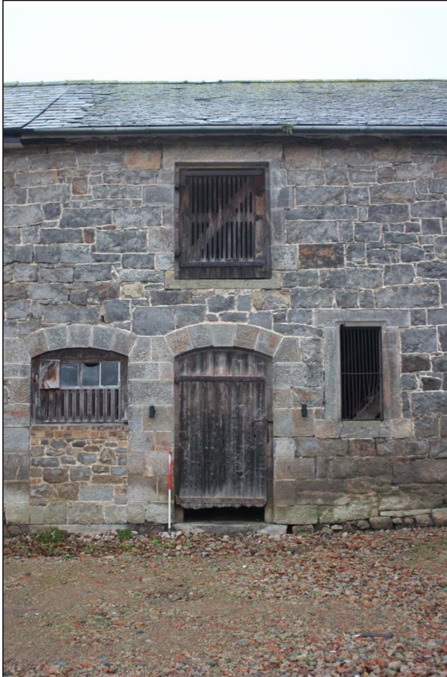
Plate 29: Llwyn y Maen, Oswestry, Shropshire. Courtyard elevations - north-eastern elevation of north-western range (door to Room 7) - From the south-east - scale 1.0m
