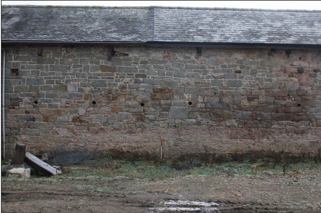
Plate 11: Llwyn y Maen, Oswestry, Shropshire. South-western range, south-west elevation left of centre - From the south-west - scale at 1m
