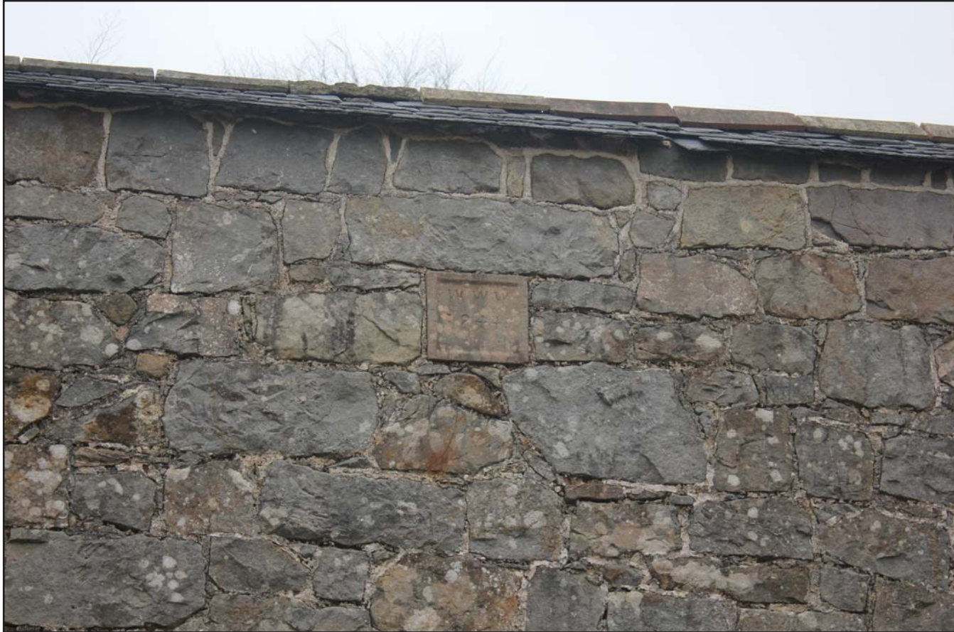
Plate 21B: Llwyn y Maen, Oswestry, Shropshire. Courtyard elevations - south-eastern elevation - Pig sties - Date stone with recoded date - From the east - scale 1.0m
