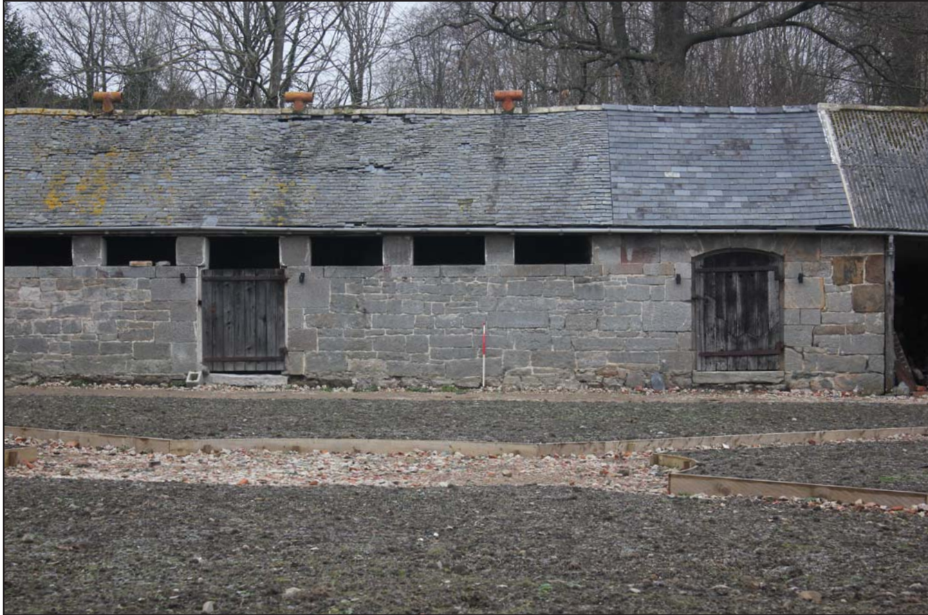
Plate 24: Llwyn y Maen, Oswestry, Shropshire. Courtyard elevations - south-eastern elevation of Room 10 & 9 - From the south-east - scale 1.0m
