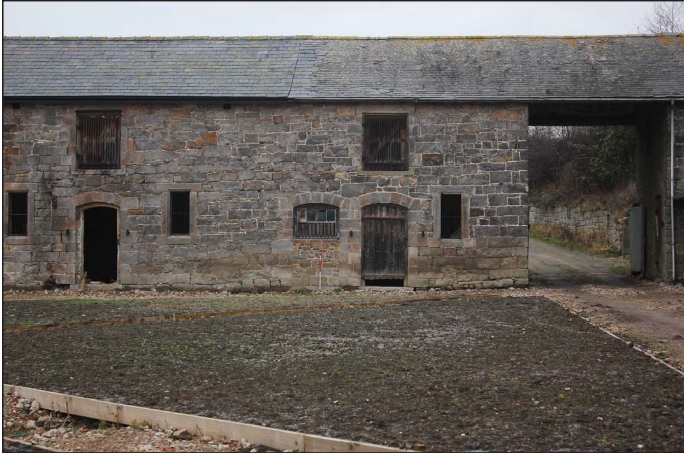
Plate 28: Llwyn y Maen, Oswestry, Shropshire. Courtyard elevations - north-eastern elevation of north-western range (doors Rooms 7 & 8) - From the south-east - scale 1.0m
