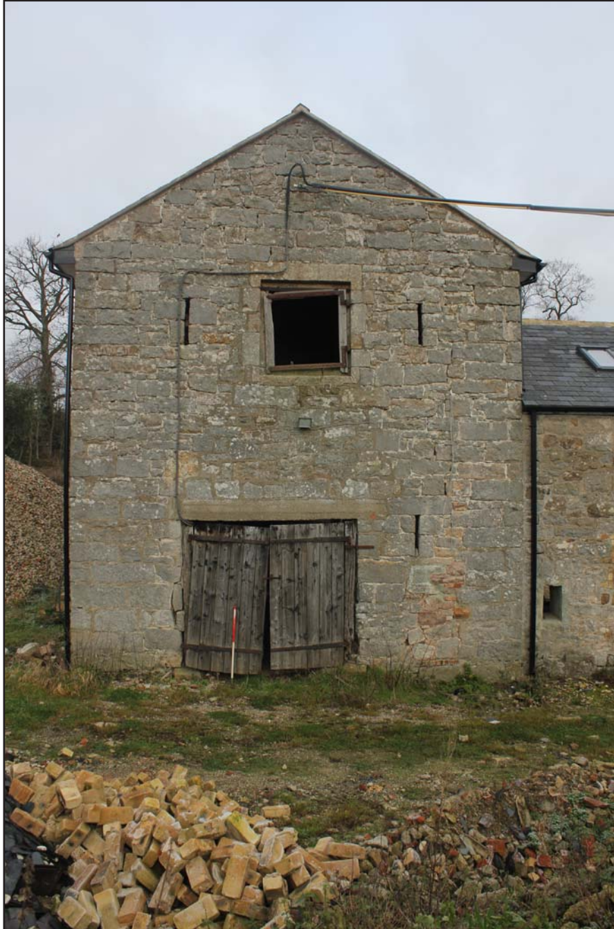
Plate 06: Llwyn y Maen, Oswestry, Shropshire. South-eastern range, south-east elevation (south-west range gable end) - From the south-east - scale at 1m
