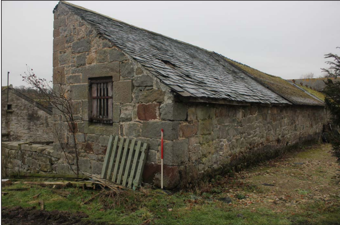
Plate 19: Llwyn y Maen, Oswestry, Shropshire. North-west and north-east elevations - From the north - scale at 1m
