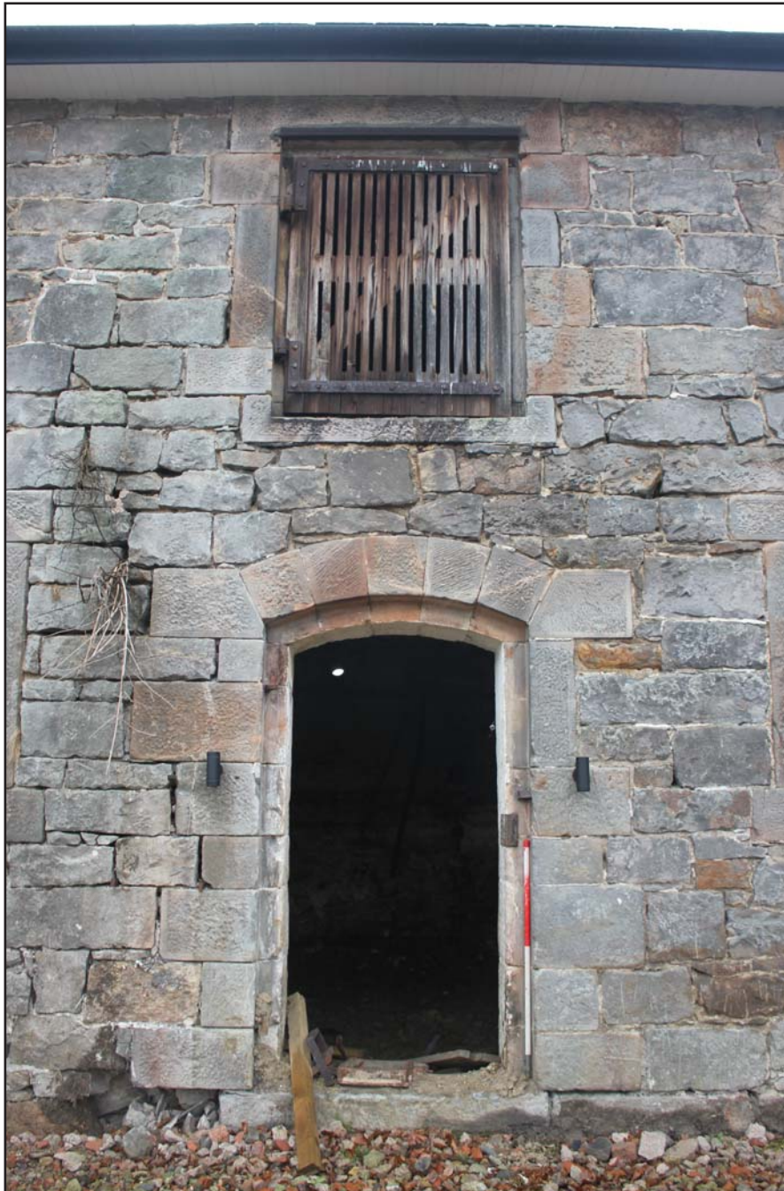
Plate 30: Llwyn y Maen, Oswestry, Shropshire. Courtyard elevations - north-eastern elevation of north-western range (door to Room 6) - From the south-east - scale 1.0m
