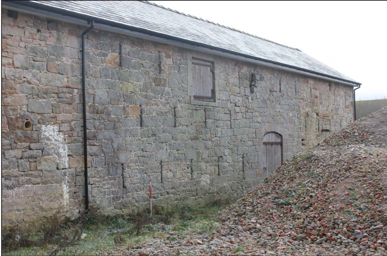
Plate 09: Llwyn y Maen, Oswestry, Shropshire. South-western range, south-west elevation right hand end - From the west - scale at 1m
