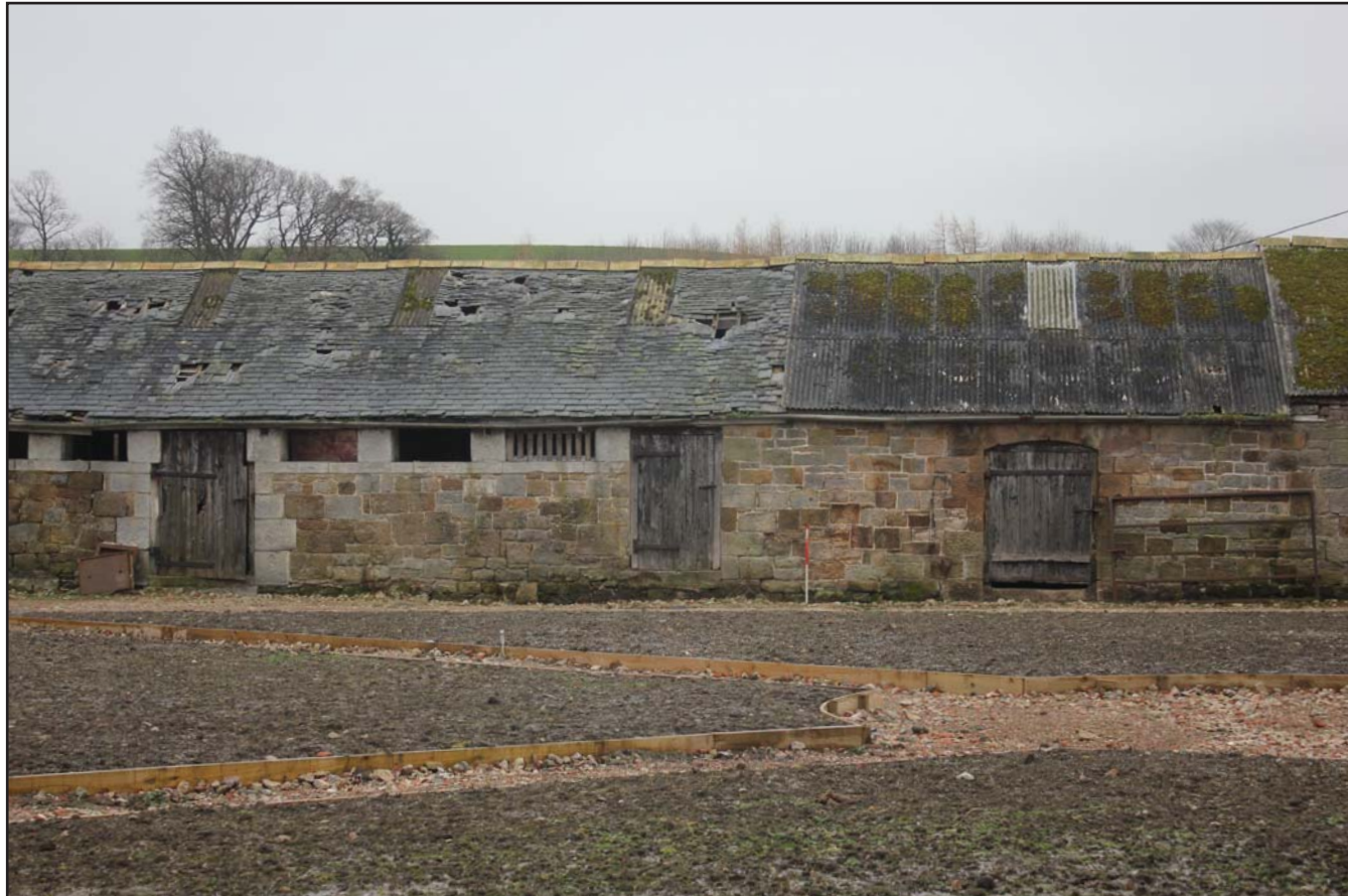
Plate 35: Llwyn y Maen, Oswestry, Shropshire. Courtyard elevations - north-western elevation of south-eastern range (doors to Room 10 & 11) - From the south-east - scale 1.0m
