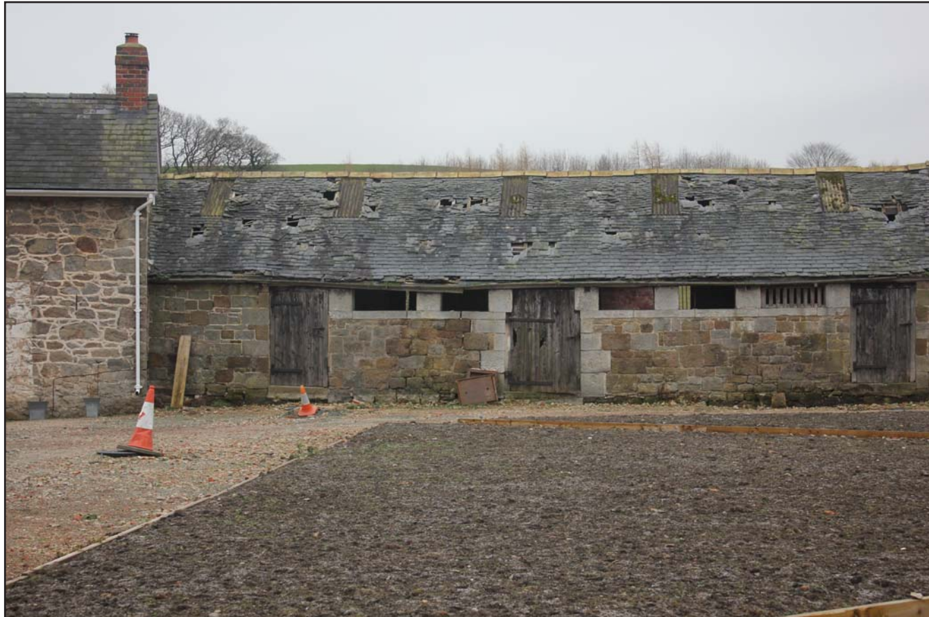
Plate 36: Llwyn y Maen, Oswestry, Shropshire. Courtyard elevations - north-western elevation of south-eastern range (door to Room 11) - From the south-east - scale 1.0m
