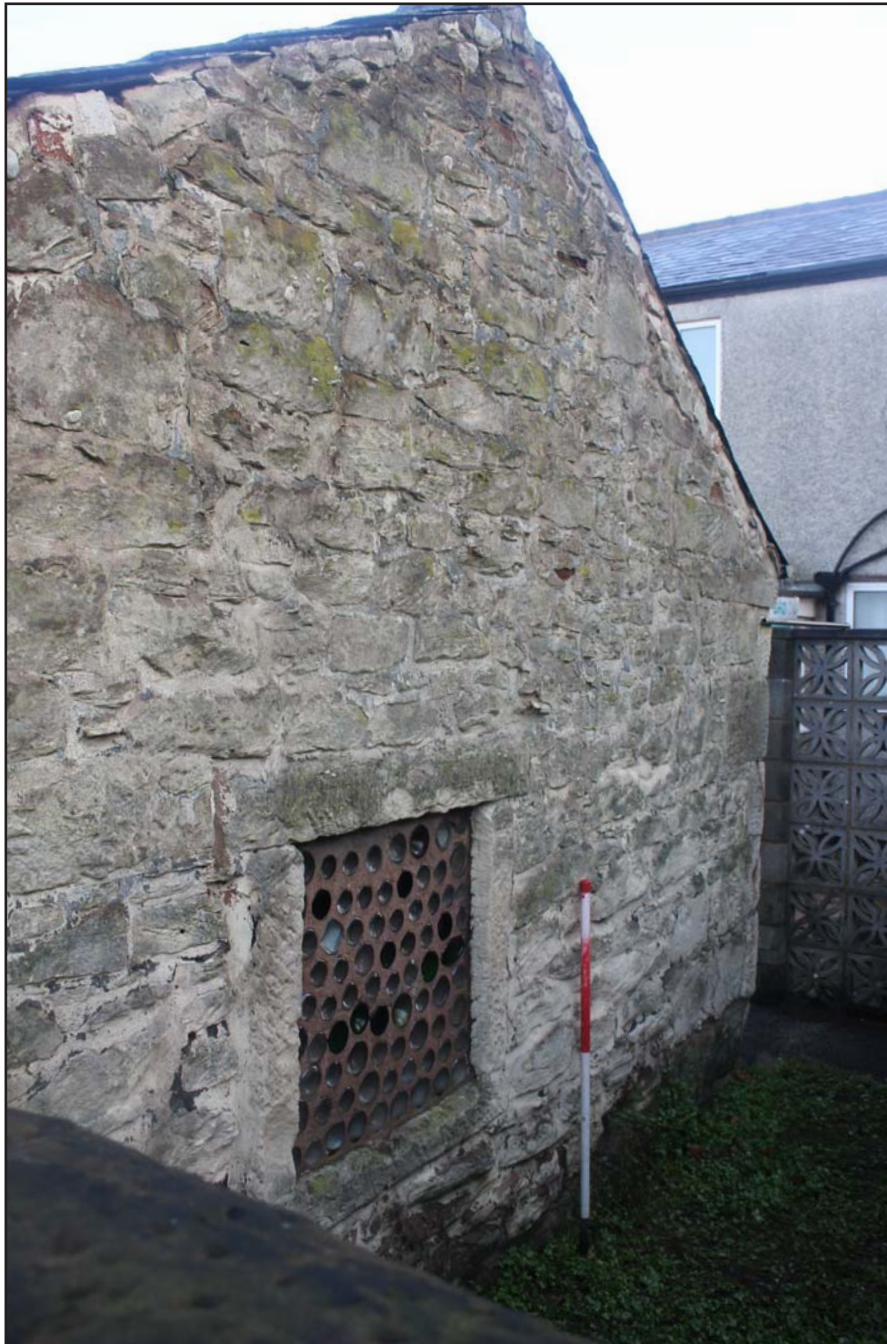
Plate 28: 317, Upton Lane, Widnes - Externals; north-western and south-western elevations of Outbuilding - From the west - scale 1.0m
