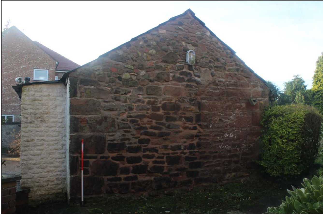
Plate 24: 317, Upton Lane, Widnes - Externals; north-eastern-eastern elevation of Outbuilding - From the northeast - scale 1.0m
