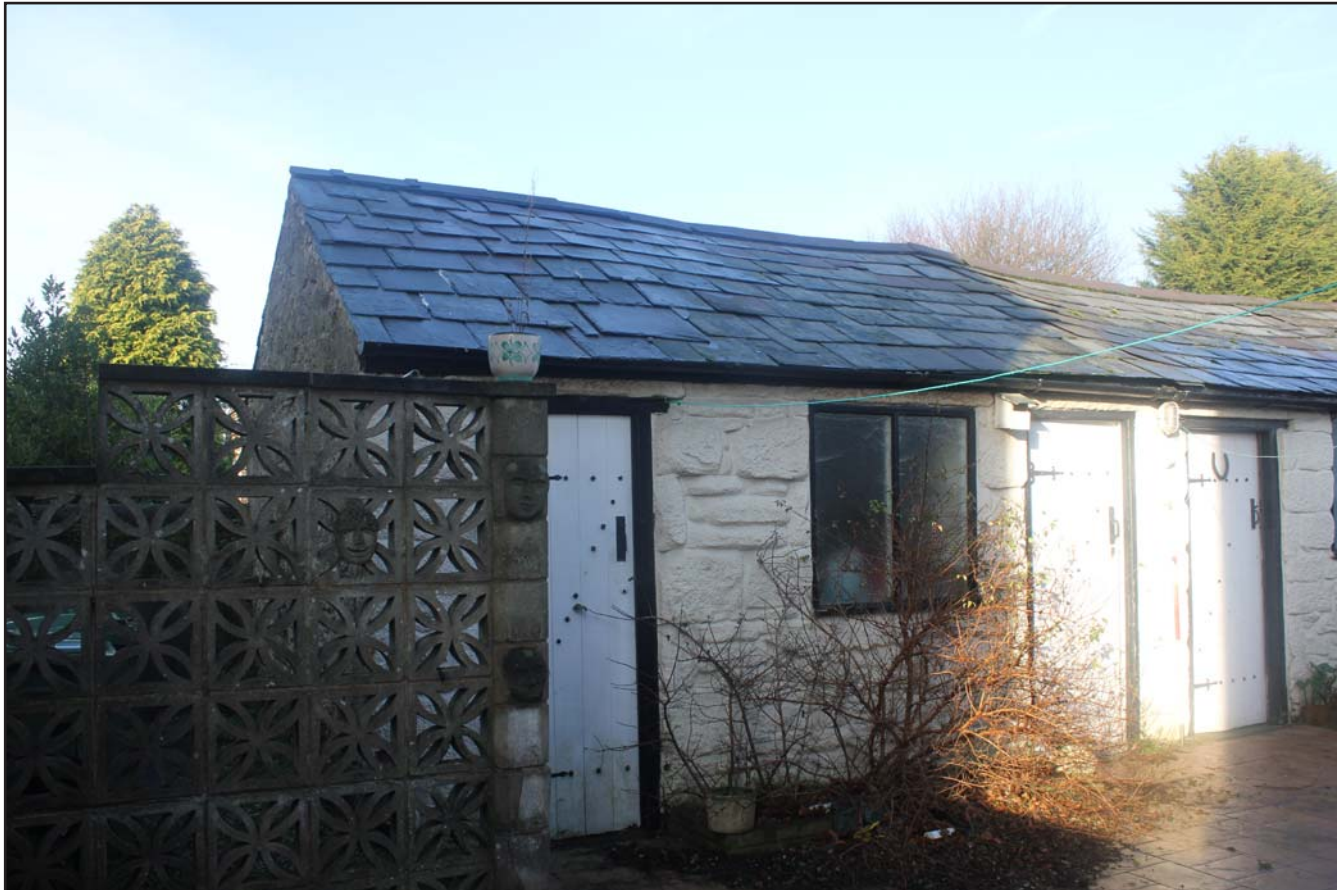
Plate 21: 317, Upton Lane, Widnes - Externals; south-western and south-eastern elevations of Outhouse - From the east - scale 1.0m
