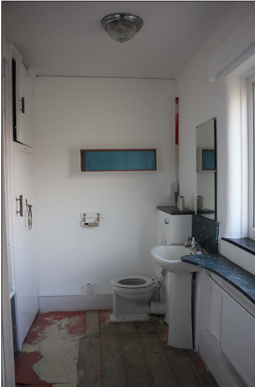
Plate 20: 317, Upton Lane, Widnes - Internal 1F: Bathroom - From the north east - scale 1.0m
