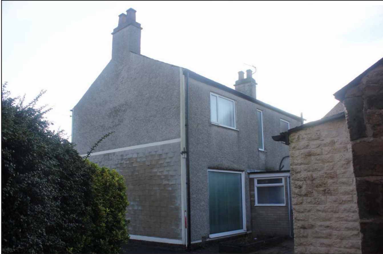
Plate 05: 317, Upton Lane, Widnes external north-eastern and north-western elevations - From the north - scale 1.0m
