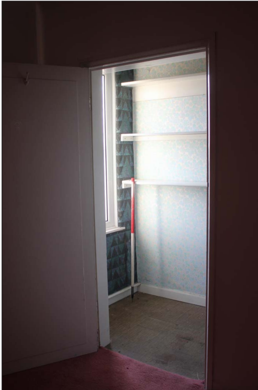
Plate 18: 317, Upton Lane, Widnes - Internal 1F: Walk in wardrobe (Bedroom 1) - From the north - scale 1.0m
