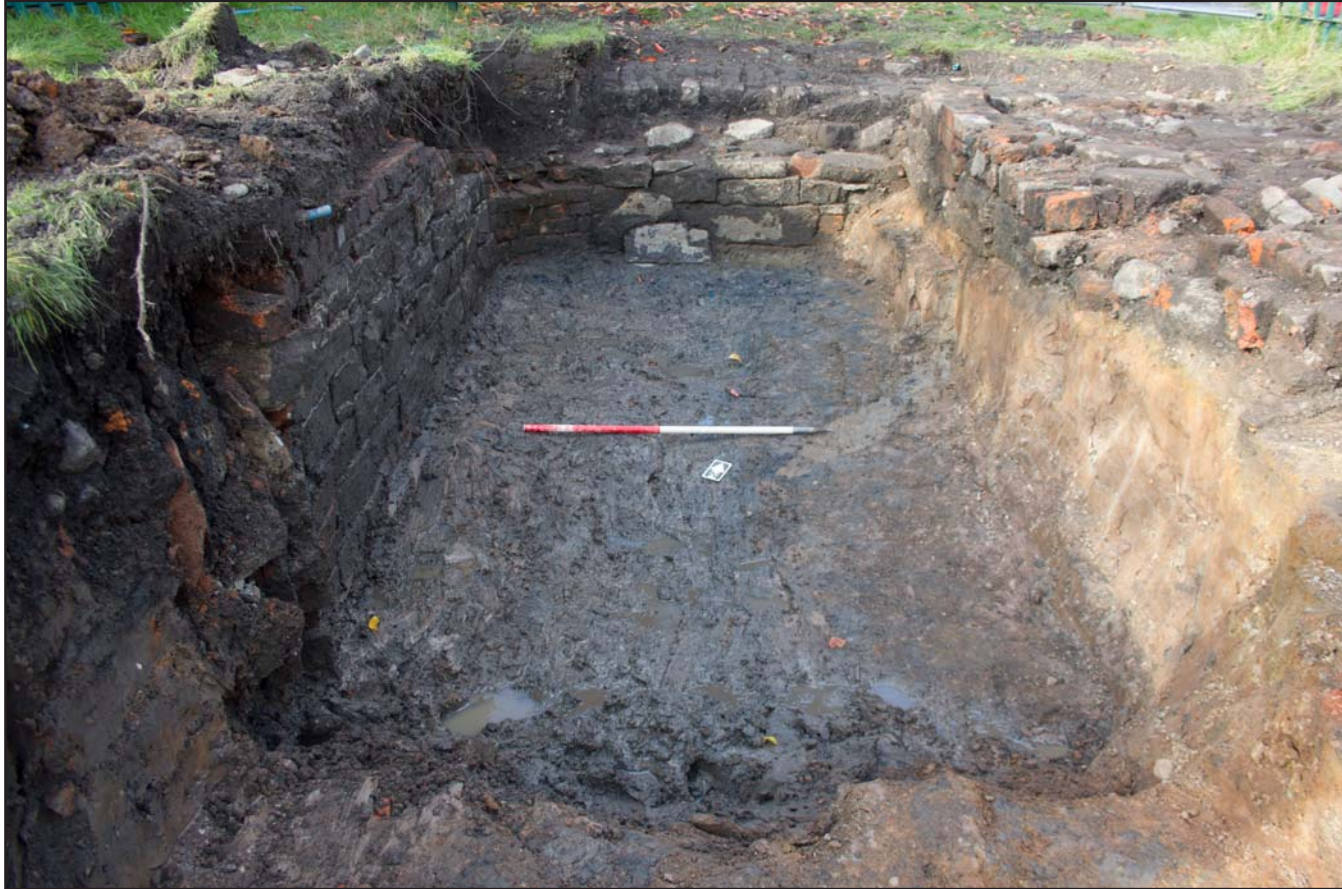
Plate 18: Wall (103) forming tank/cess pit at Mill Wood Avenue, Eccleston, St. Helens, Merseyside - from the southeast - scale 1m
