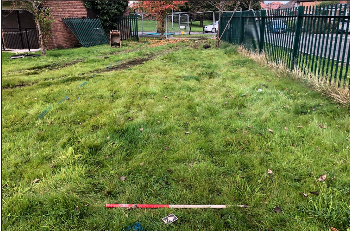
Plate 02: Pre excavation shot of trench at Mill Wood Avenue, Eccleston, St. Helens, Merseyside - from the southeast - scale 1m
