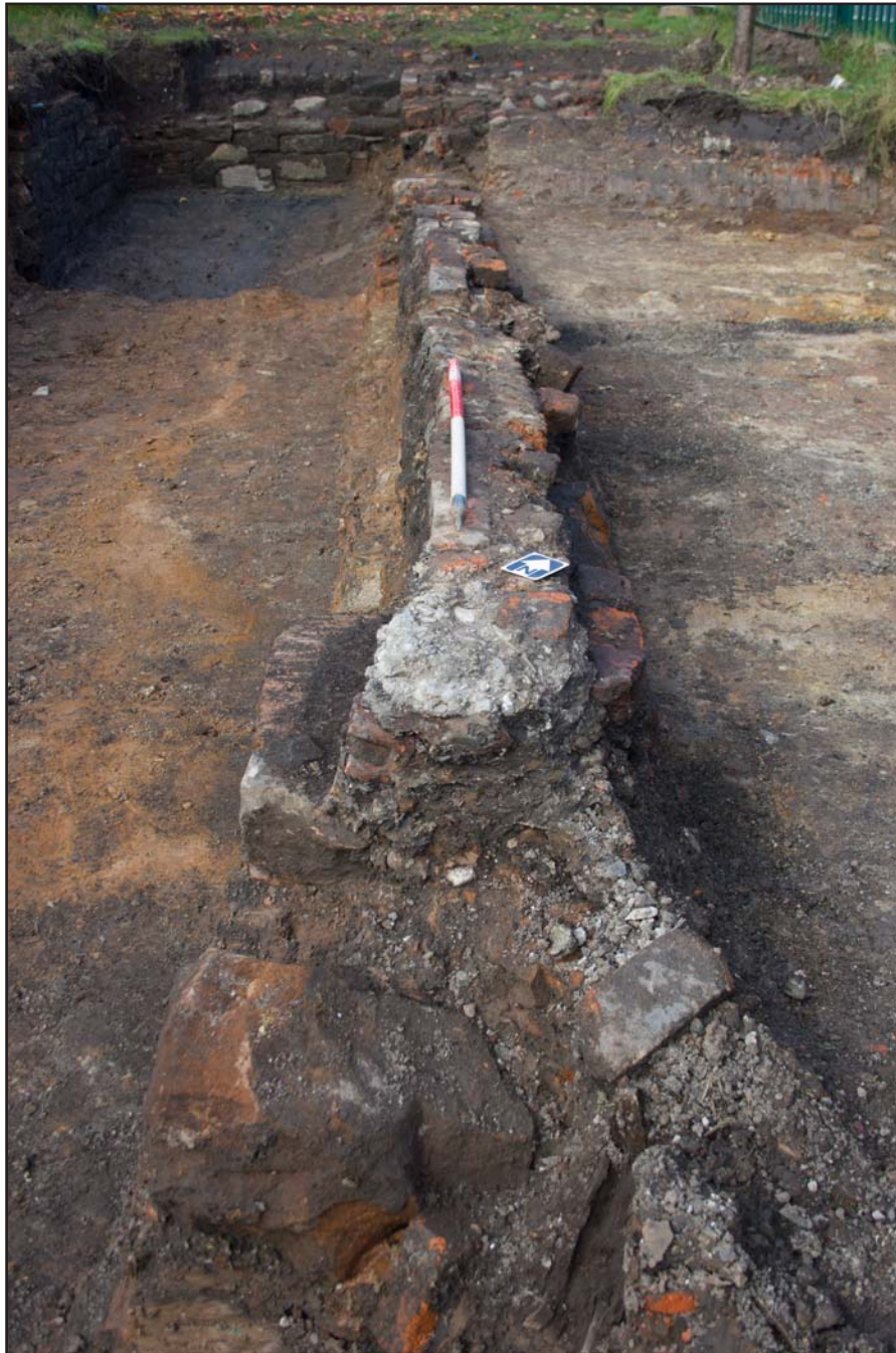
Plate 07: Long northwest to southeast wall (102) at Mill Wood Avenue, Eccleston, St. Helens, Merseyside - from the southeast - scale 1m
