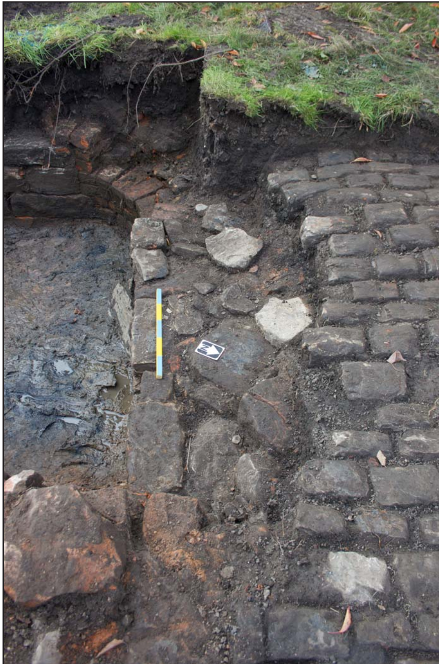
Plate 14: North western return of wall (103) at Mill Wood Avenue, Eccleston, St. Helens, Merseyside - from the south - scale 0.50m
