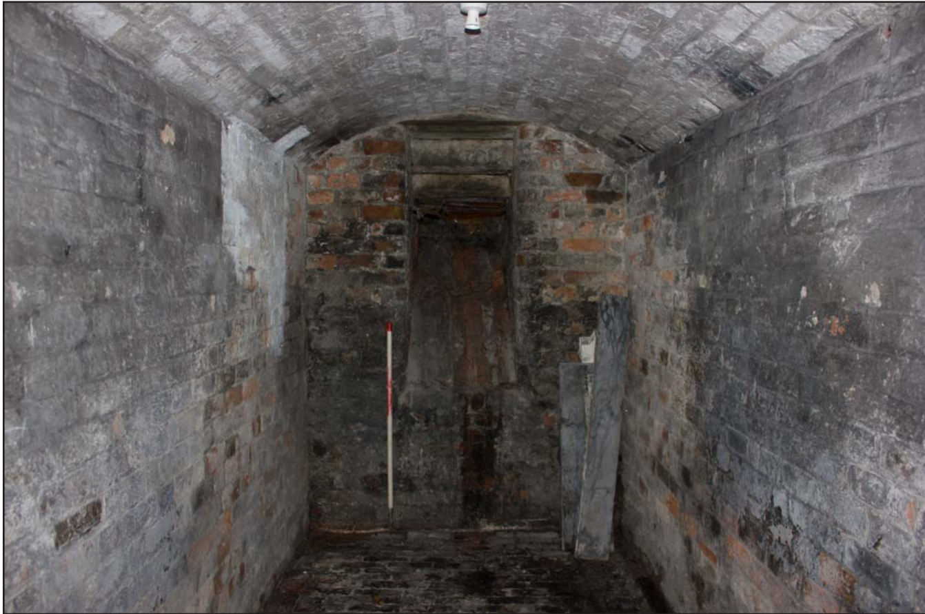
Plate 20: Cellar B4 showing coal chute and barrel vaulted roof, from the north. Scale 1.0m.
