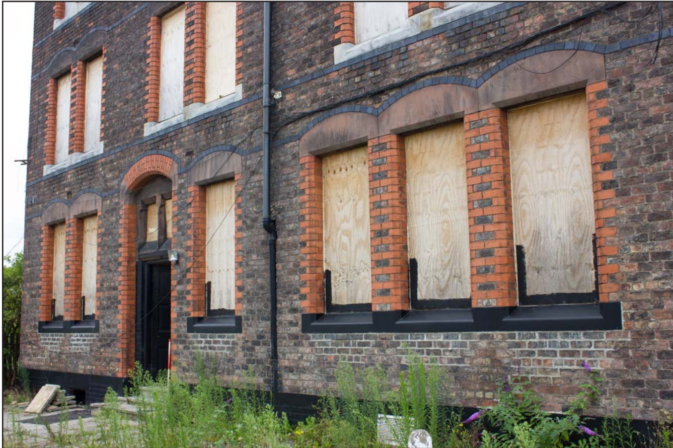
Plate 03: Southern principle external elevation showing ground floor detail, from the southeast. Scale 1.0m.
