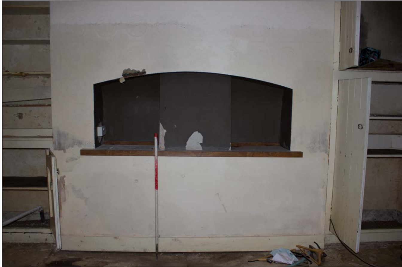
Plate 40: Ground floor Store 2 showing blocked up fireplace, from the east. Scale 1.0m.
