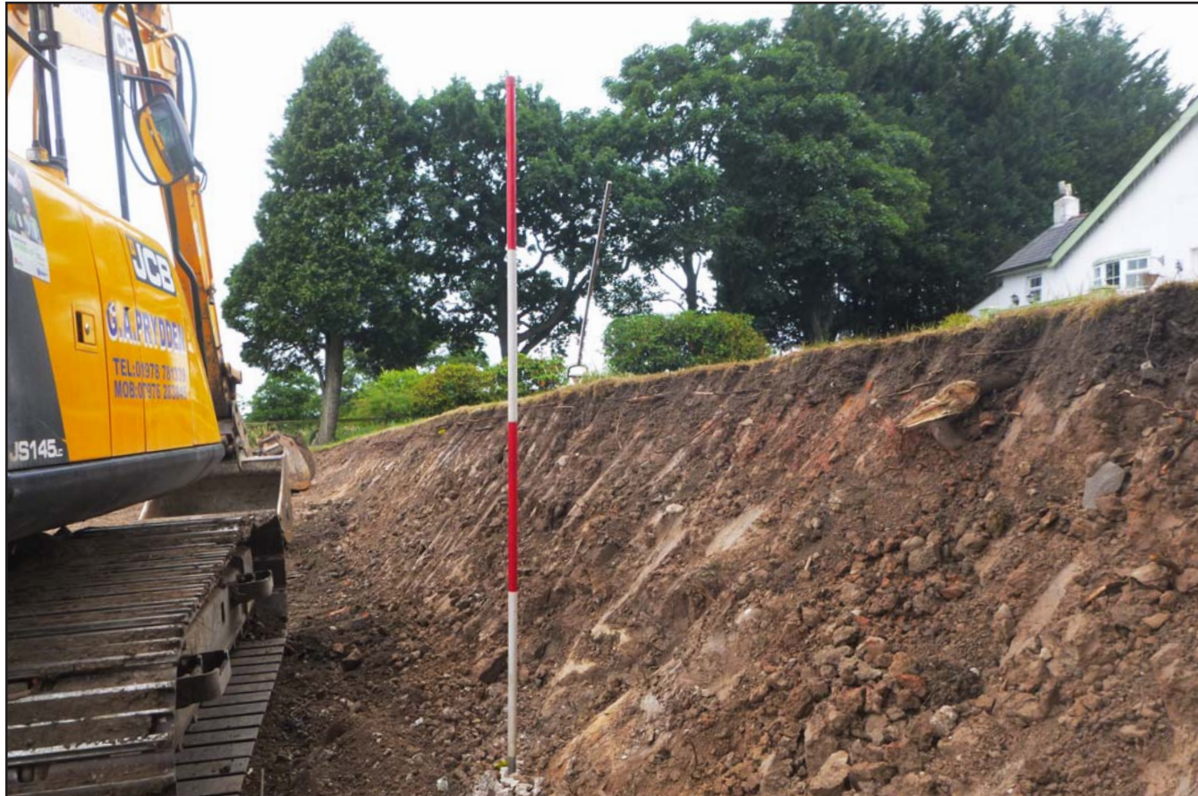
Plate 04: Section of bank on the western boundary (along section) - from the southwest - scale 2m
