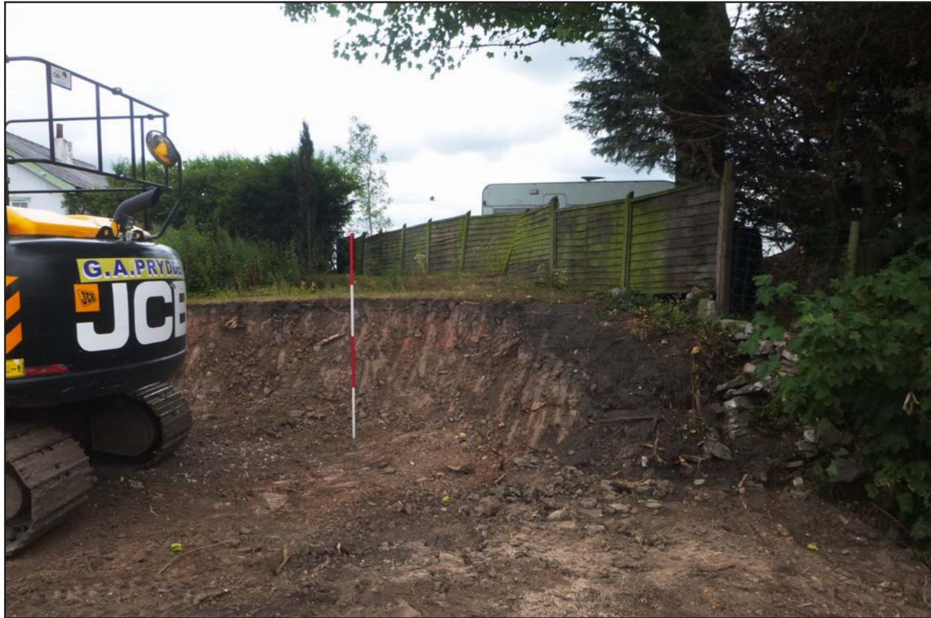
Plate 03: Section of bank on the western boundary - from the west - scale 2m
