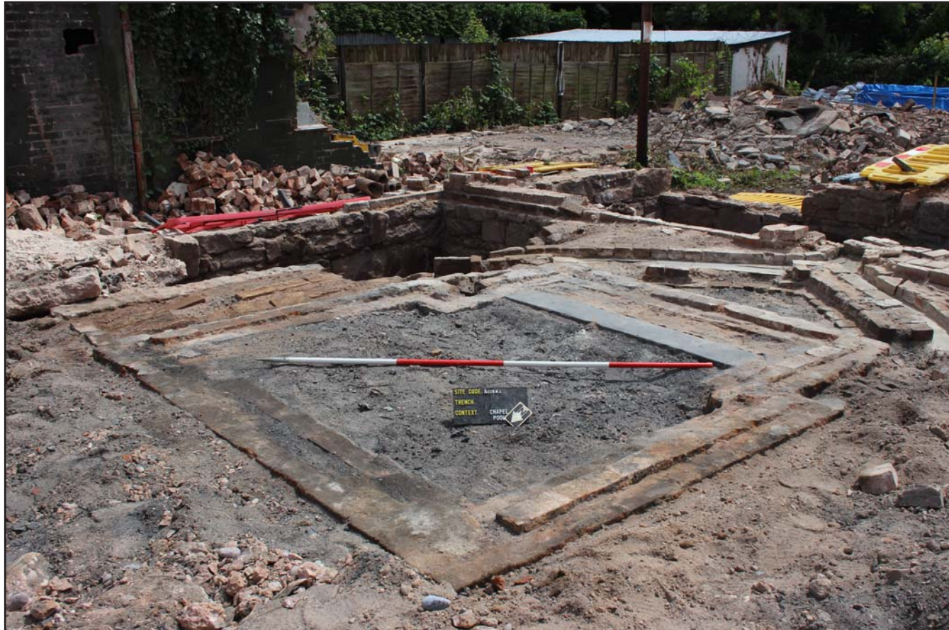
Plate 40: Grey brown ash (104) backfill found covering the whole site beneath the concrete floor slab (101) - from the west - scale 1m
