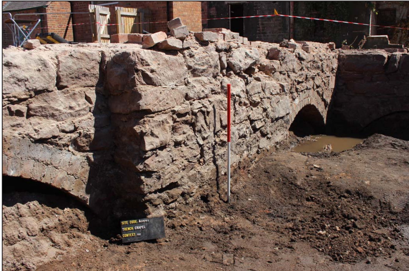
Plate 22: Butress (112) situated to south of interior wall (110) - from the southwest - scale 1m
