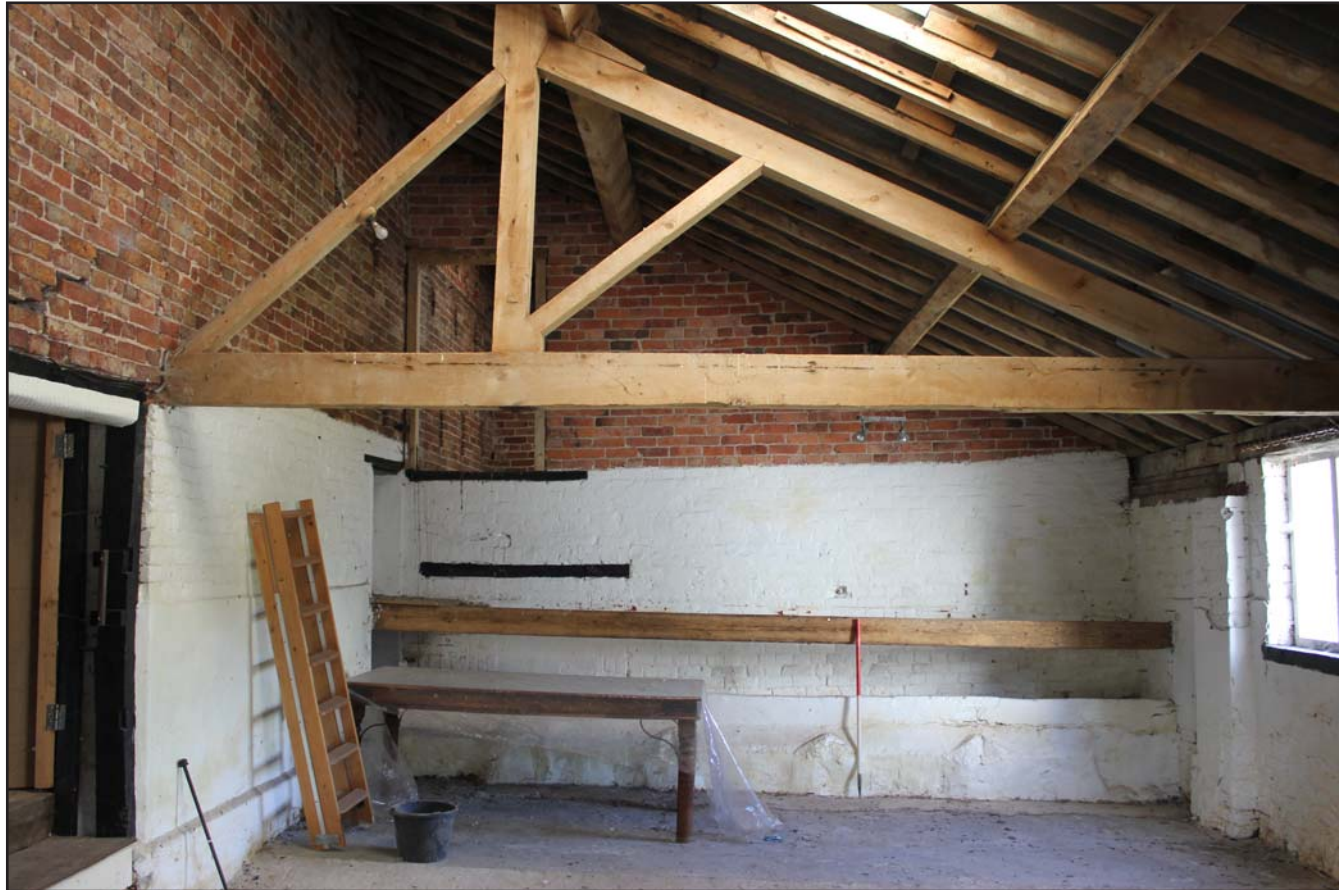
Plate 30: Grimsditch Farm - Northeast Extension Stable interior showing Dualpitch truss, from the southeast. Scale 1.0m.
