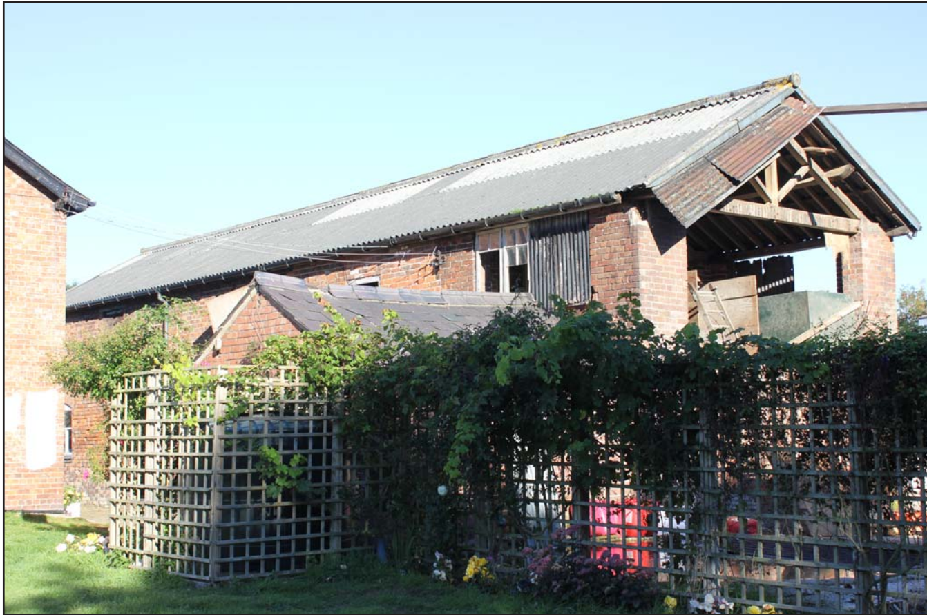
Plate 05: Grimsditch Farm - Barn southwest external elevation and Hay Barn southwest and southeast elevations, from the south.
