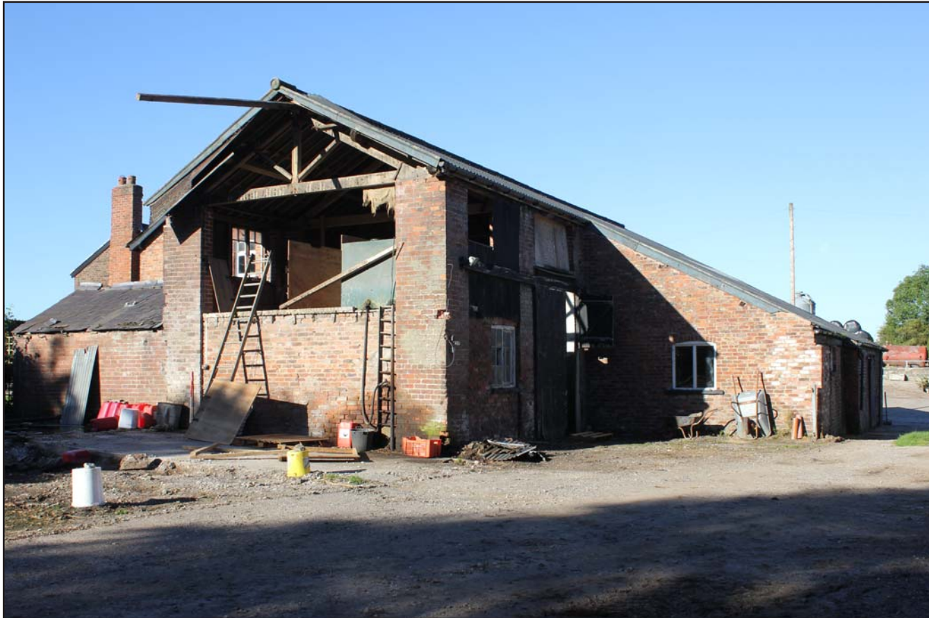
Plate 07: Grimsditch Farm - Hay Barn southeast and northeast external elevations, from the east. Scale 1.0m.
