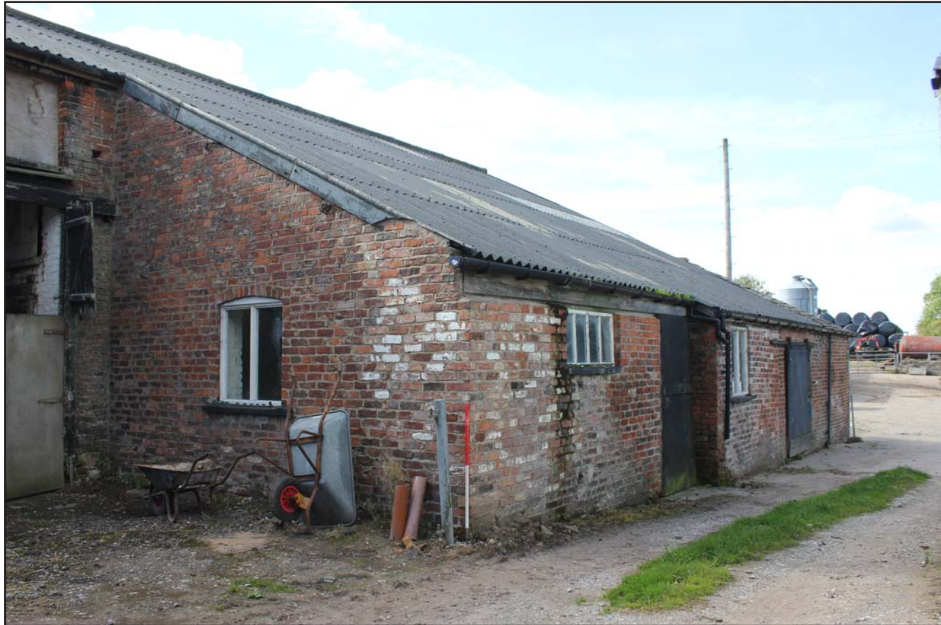
Plate 13: Grimsditch Farm - Northeast Extension southeast and northeast external elevations, from the east. Scale 1.0m.
