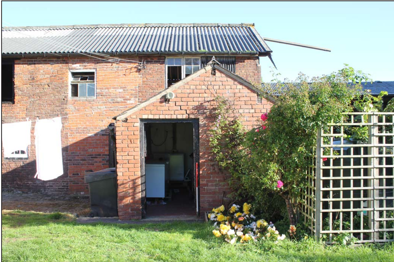
Plate 16: Grimsditch Farm - Southwest Extension southwest external elevation, from the southwest. Scale 1.0m.
