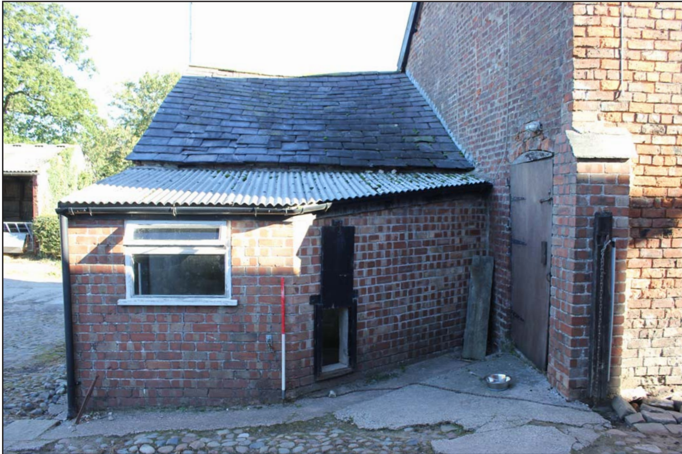
Plate 20: Grimsditch Farm - Kennel Extension southwest external elevation, from the southwest. Scale 1.0m.
