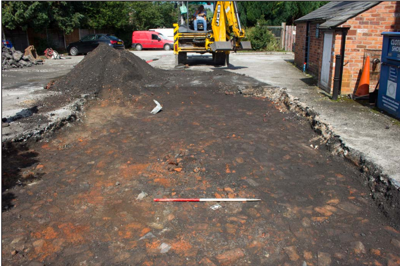
Plate 02: Brick demolition layer (104) revealed beneath dark ash layer (103) - from the southeast - scale 1m
