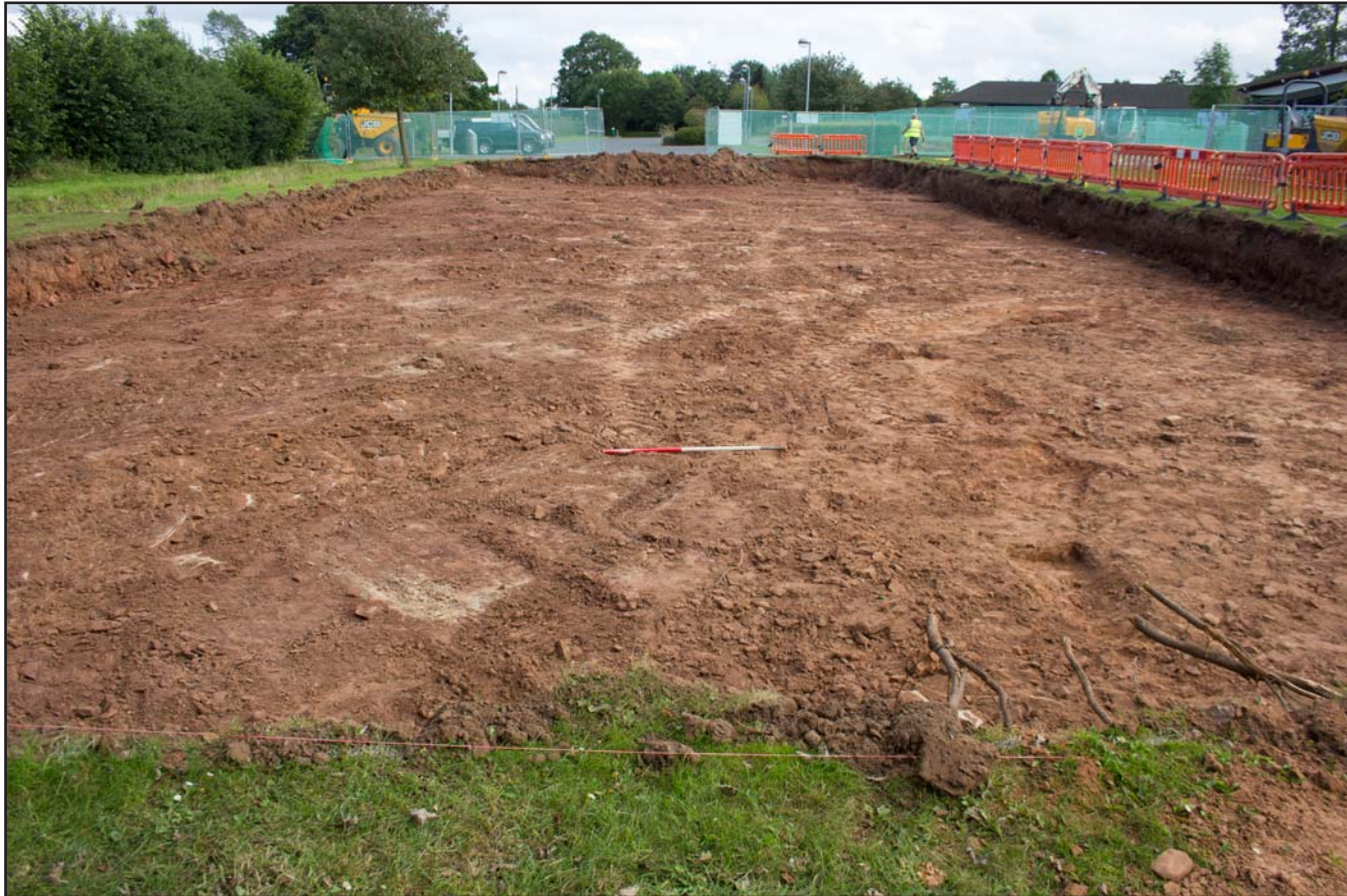
Plate 06: Post excavation shot of area; Car Park A at Telford Crematorium, Woodhouse Lane, Redhill, Shropshire, TF2 9NJ - from the northwest - scale 1m.
