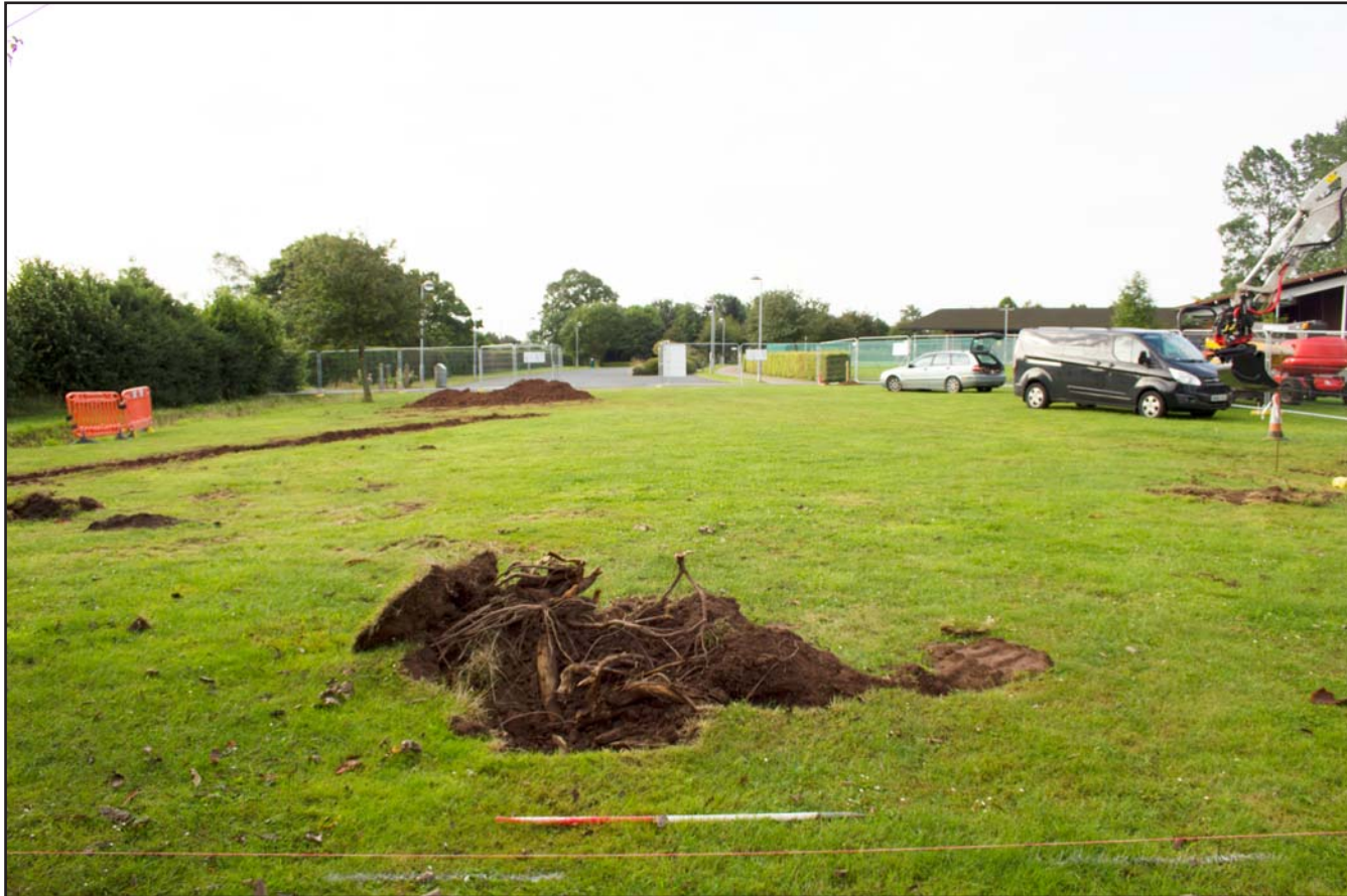
Plate 02: Pre excavation shot of area; Car Park A at Telford Crematorium, Woodhouse Lane, Redhill, Shropshire, TF2 9NJ - from the northwest - scale 1m.
