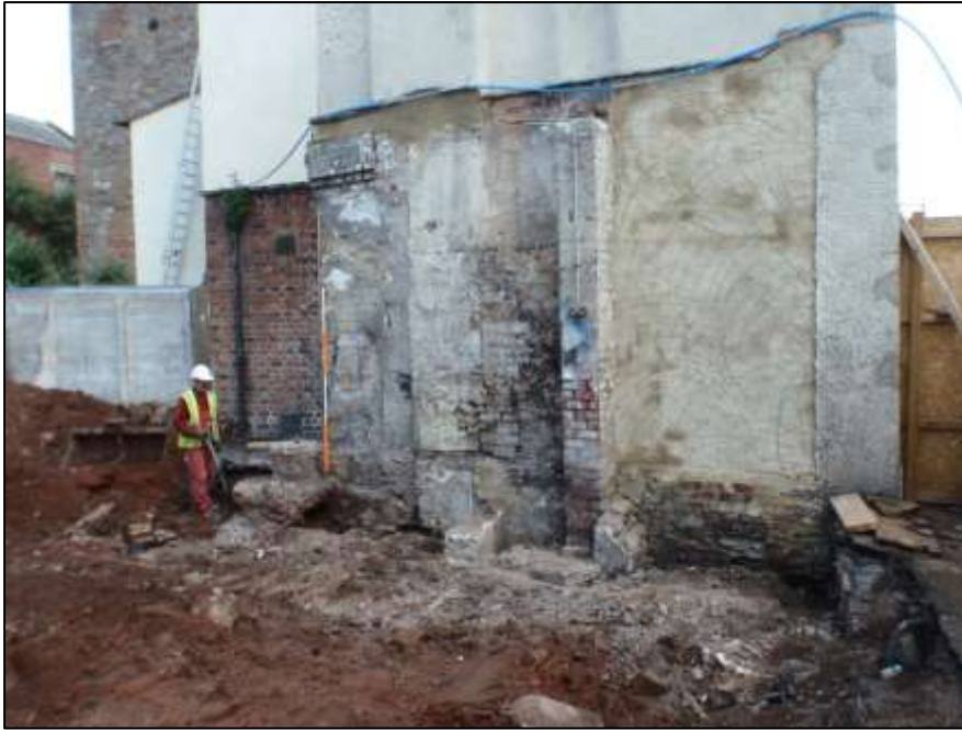
Plate 3. General view of the N side of site during hand excavation of foundations showing suggested remains of cellar walls, looking N, scale 2m.
