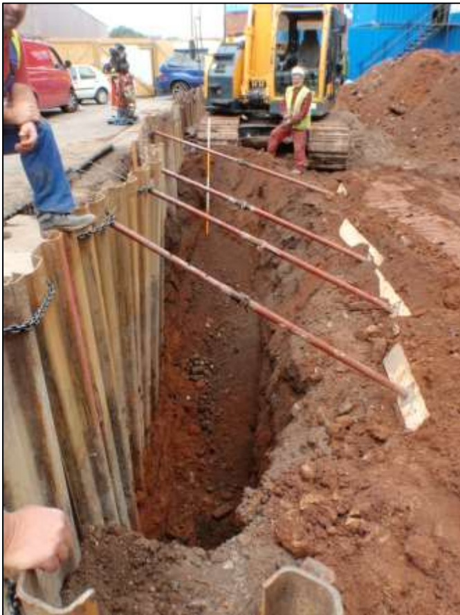
Plate 4. Strip foundations along the Eugene Street frontage during excavation, looking W, scale 2m.
