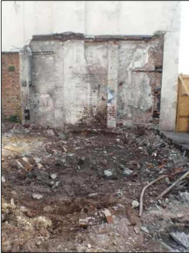
Plate 1. Pennywell Road site frontage after demolition and removal of floors and surfaces showing base for fireplace, looking N. Scale 0.5m.
