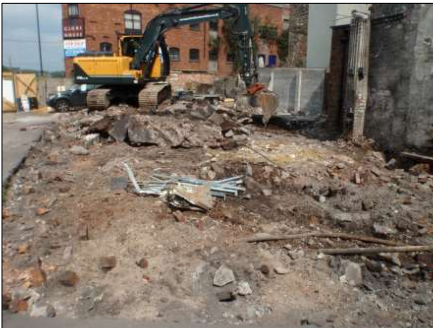
Plate 2. General view of the site during removal of modern surfaces, looking W
