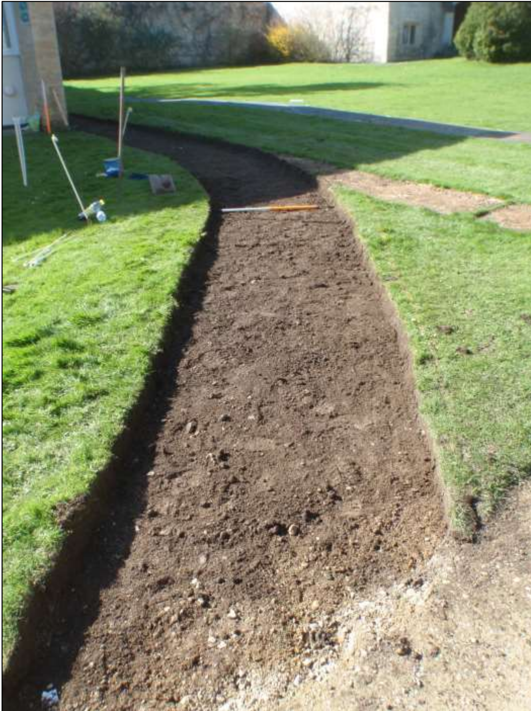
Plate 1. East half of the new footpath as excavated, looking W. Scale 1m.
