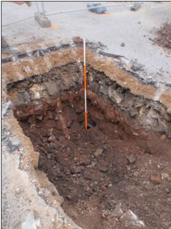
Plate 2. STP03 as excavated, with culvert in SW corner, looking SW, scale 2m
