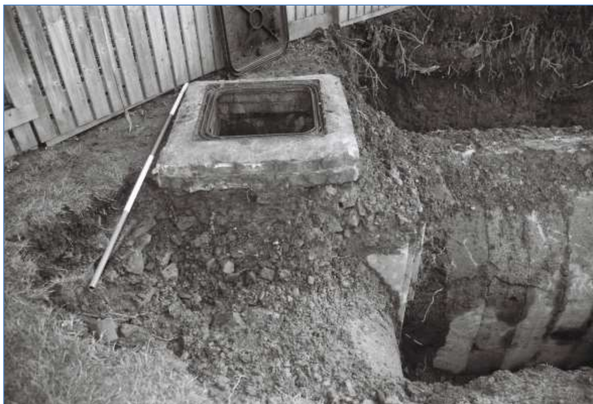
Plate 2: Detail of the manhole escape point at the junction of Tunnels A & B (1.26)
