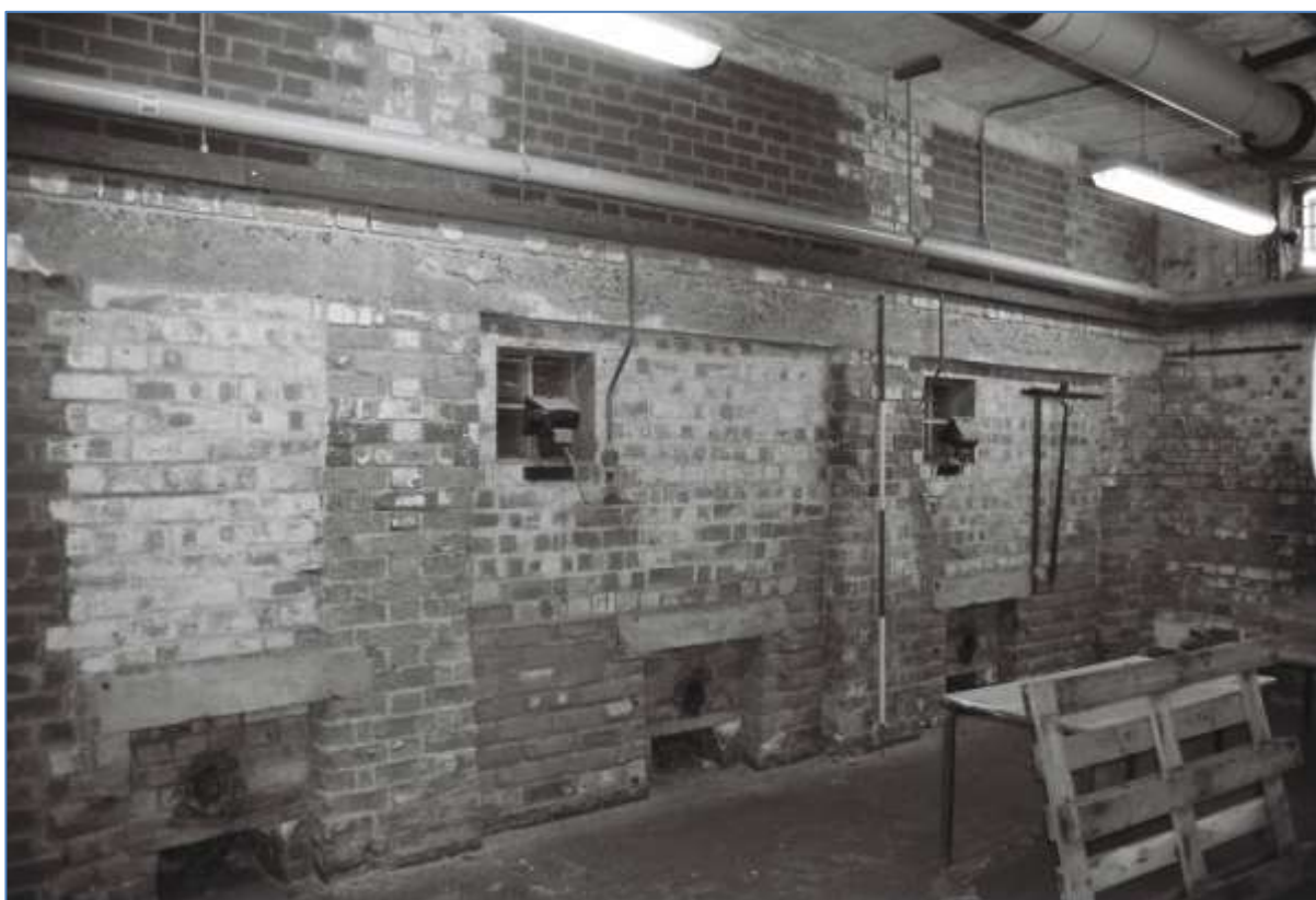
Plate 24: General view of boiler room, evidence of rebuilding and slots for the former coal worm drives (Film 1.12)
