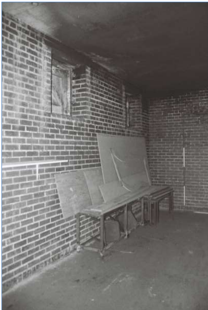
Plate 25: General view of coal store. The three wooden hatch doors are situated above a change in the brick work which possibly indicates later rebuilding (Film 1.13)
