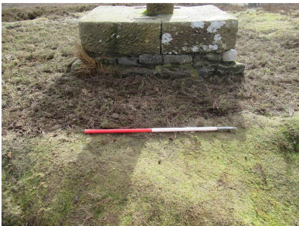
Plate 14 : A view of the repaired hollow surrounding the monument after remedial work (February 2018)
