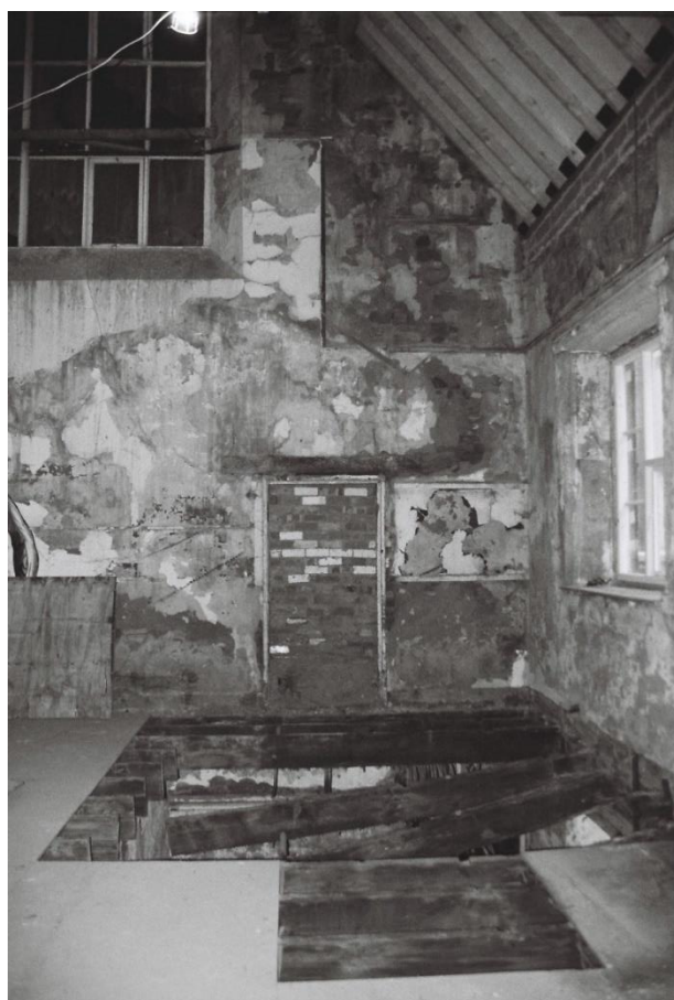
Plate 38: Detail of blocked door to former entrance porch and stair tower, Room F1 (Film/Frame 2.6).
