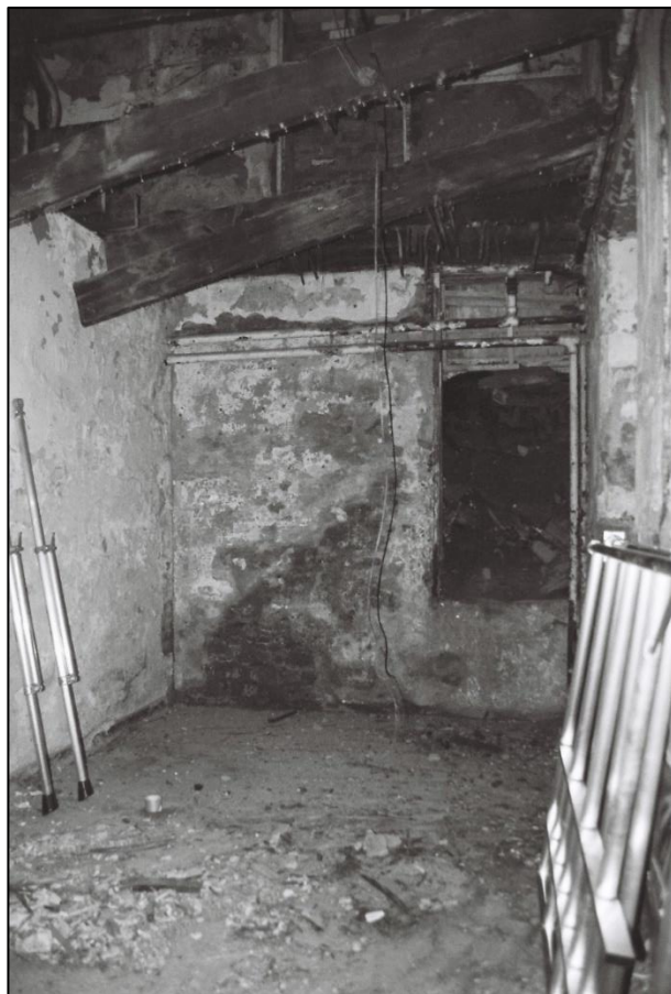
Plate 29: General view of Room G4, note blocked door leading to the former stair tower (Film/Frame 3.28)
