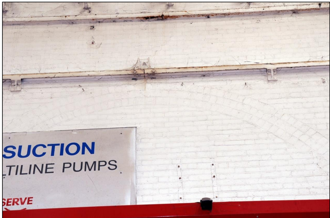
Plate 24: Detail of arch above northern doorway in western range of Building 4 (image 0003).
