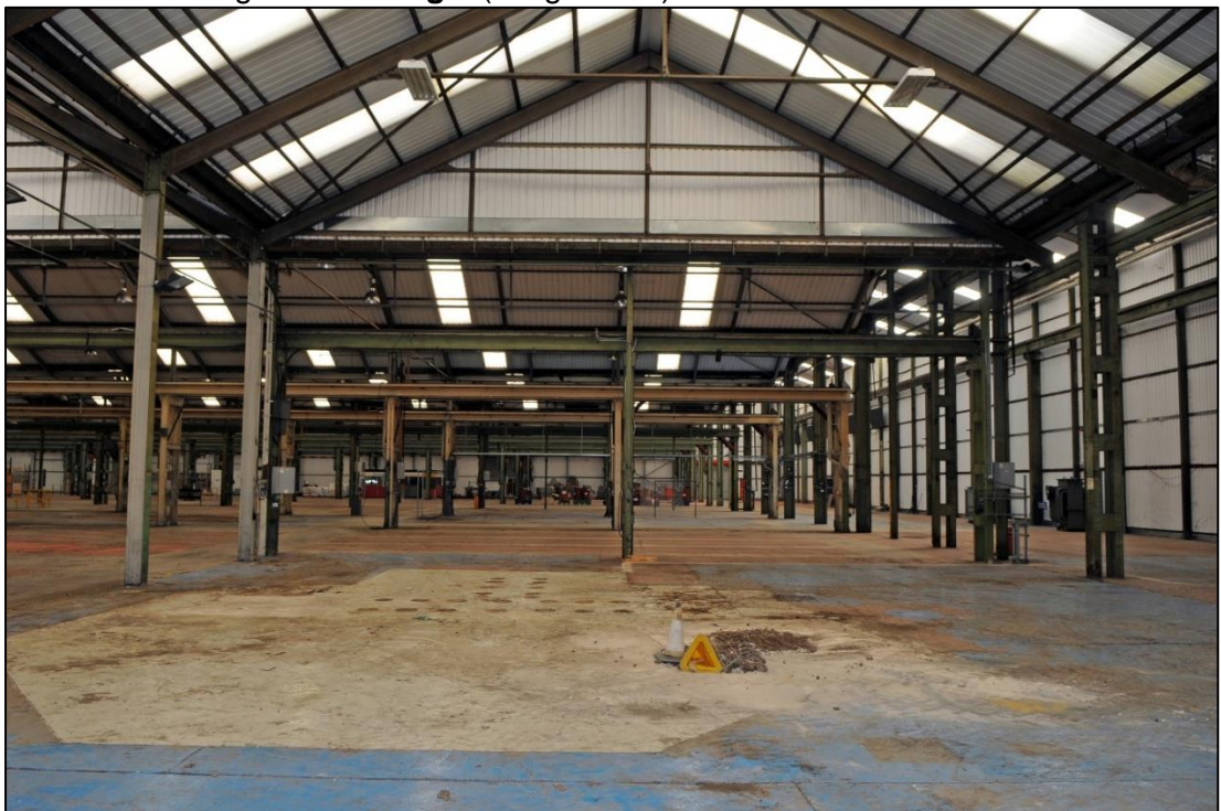
Plate 34: General view of one range of double pitched roof leading into the eastern range of Building 4 (image 16).
