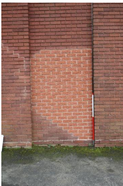
Plate 3: Detailed view of the brick repair work in the south western most recess
