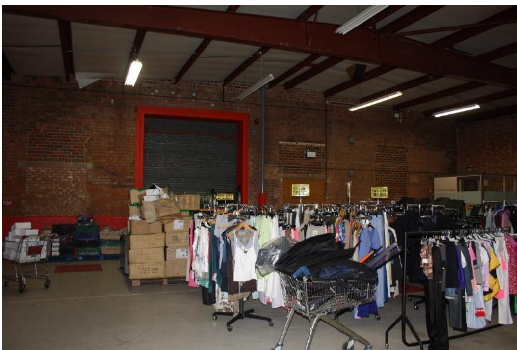
Plate 41: General view of Room 5 including the roof structure and blocked in openings along the north west wall
