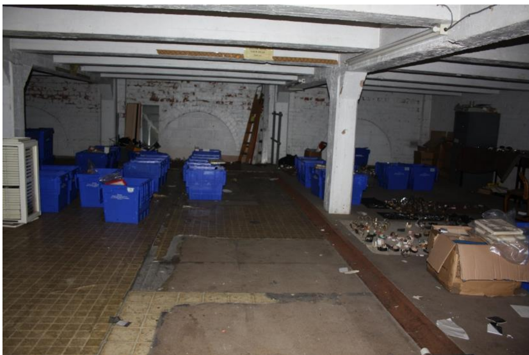
Plate 44: General view of Room 7 including the arch headers in the south east wall
