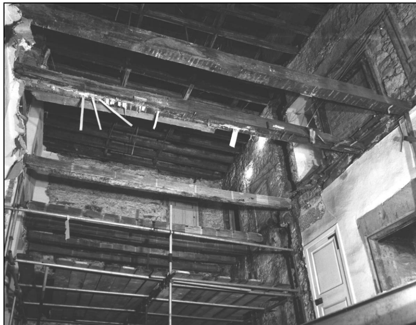
Figure 2-2: The Midhope Room during work in 1966-7, showing timber dated to the late 1560s
