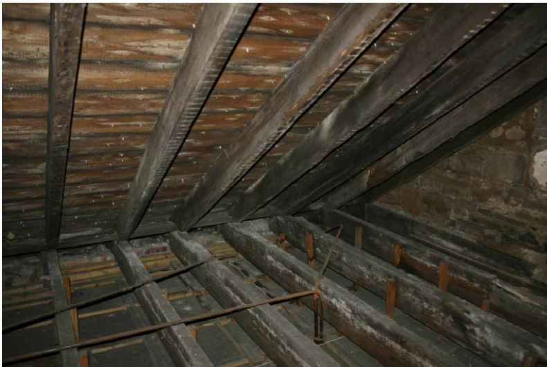
Fig. 128-7 View from south showing collar-beam (020) and northern rafter (018) of truss 6 (sixth couple from right).
