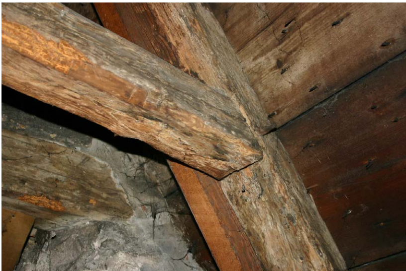
Fig. 130-22 View from northeast showing western rafter (211), western auxiliary rafter (212) and upper collar-beam (213) of truss 22.
