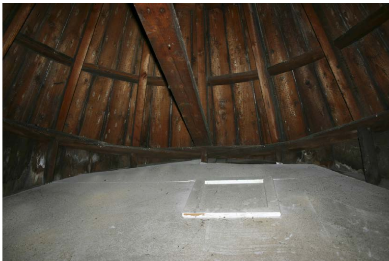
Fig. 136-1 View from north showing collar-beam and northern rafter of truss 1 (third rafter from right).
