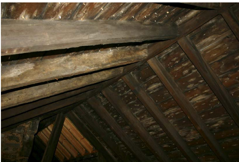
Fig. 128-28 View from south showing northern and southern rafters (064 and 085) of truss 18 (seventh couple from right).
