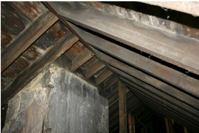
Fig. 128-56 View from northwest showing board 161 and auxiliary rafters 162-165 at head of chimney.
