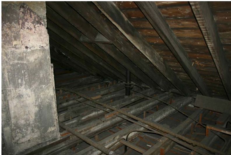
Fig. 128-45 View from south showing northern rafter (139) and northern collar-beam (140) of truss 34 (third couple from right).
