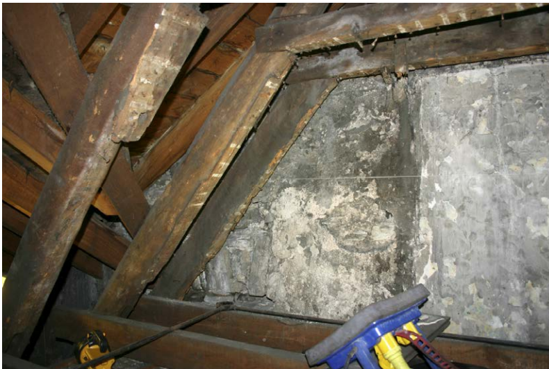
Fig. 131-1 View from east showing upper and lower collar-beams (056 and 057) and southern rafter (054) of truss 1.
