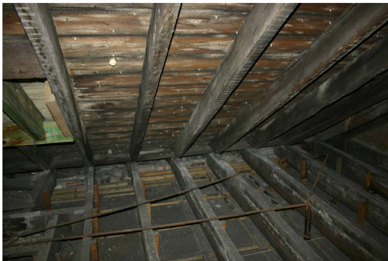
Fig. 128-9 View from south showing collar-beam (027) and northern rafter (025) of truss 8 (eighth couple from right).
