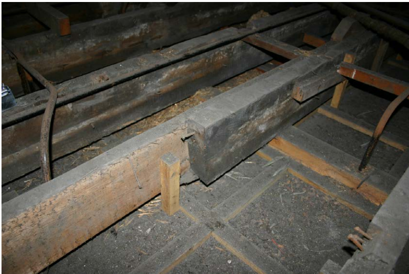
Fig. 128-8 View from northeast showing joint of collar-beams (023 and 024) of truss 7 (second couple from right).
