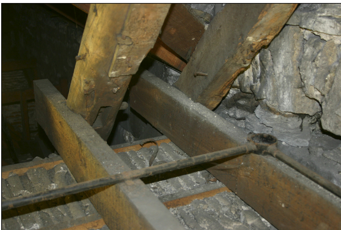
Figure A1-5: Rafter and collarbeam belonging to the roof over the kitchen. The first rafter from the left shows an empty mortise which belongs to a formerly existing collarbeam. The latter was removed when new machine-cut beams were introduced together with the extant lath-and-plaster ceiling.
