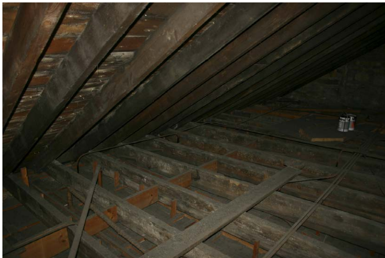
Fig. 128-55 View from north showing southern rafter and collar-beam of truss 38S (eighth couple from left).
