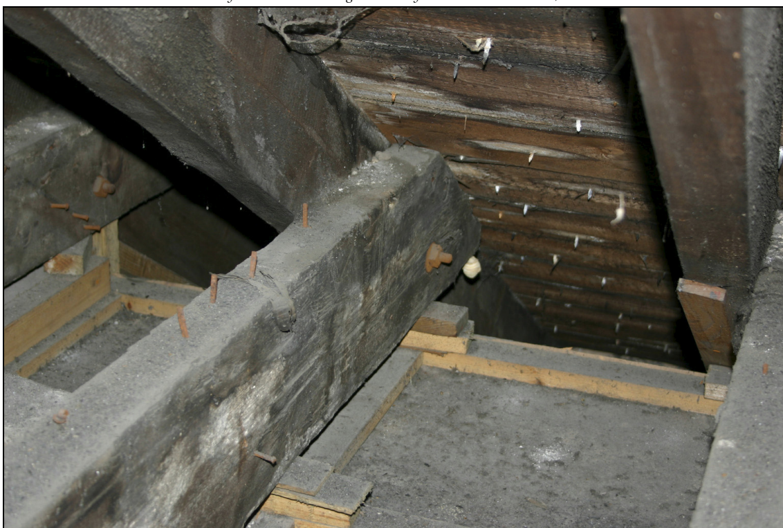
Figure A1-2: Joint between collarbeam and southern rafter over the main block. The collarbeam is attached to the lateral face of the rafter using bolts that can be found in all the other roofs at Abbey Strand.
