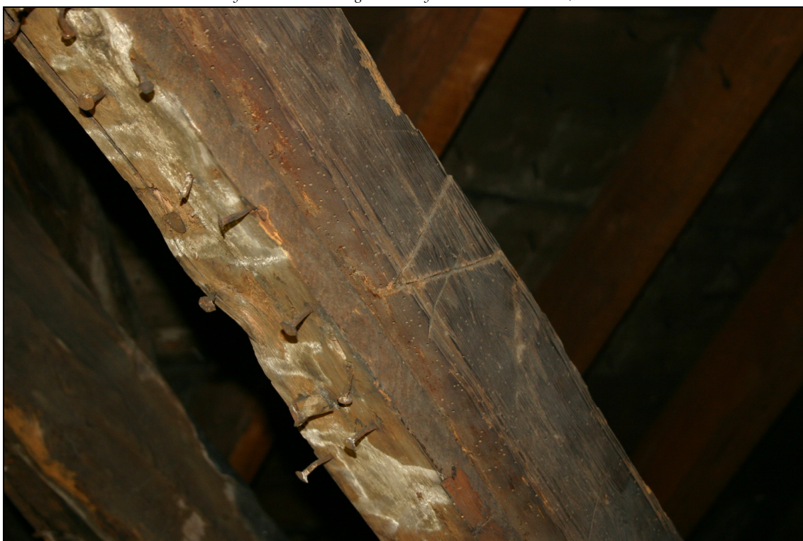
Figure A1-4: Rafter belonging to the roof over the kitchen. Being marked with Roman numerals, the beam shows at its underside handmade nails as well as residuals of a lath-and-plaster ceiling, proving that the space had some sort of residential function.
