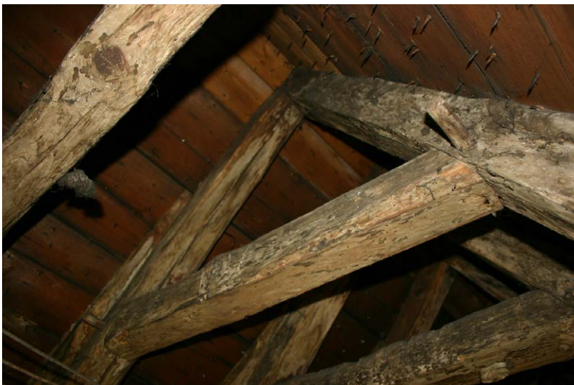
Fig. 130-7 View from southeast showing eastern and western rafters (101 and 102) and upper collar-beam (103) of truss 7.
