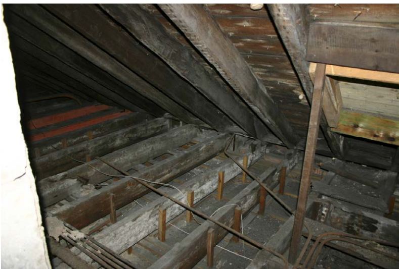
Fig. 128-22 View from southeast showing collar-beam (072) and northern rafter (071) of truss 12 (third couple from right).
