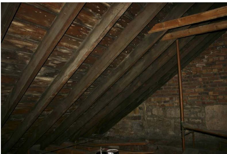
Fig. 128-59 View from northwest showing southern rafter of truss 42 (second rafter from left).
