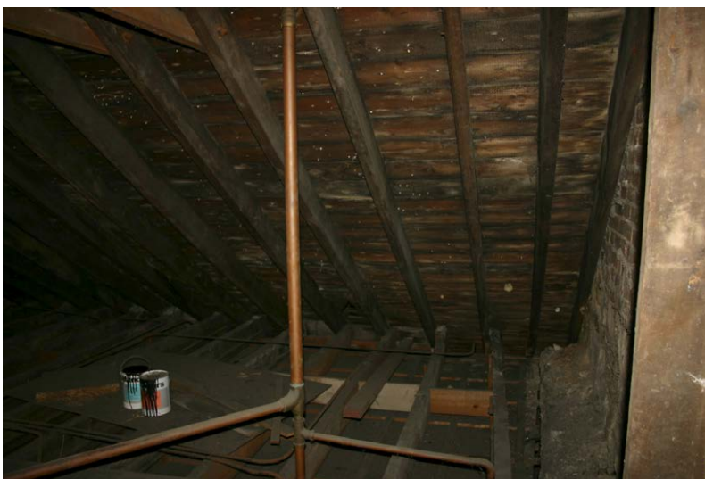
Fig. 128-58 View from north showing southern rafter and collar-beam of truss 41 (seventh rafter from right).
