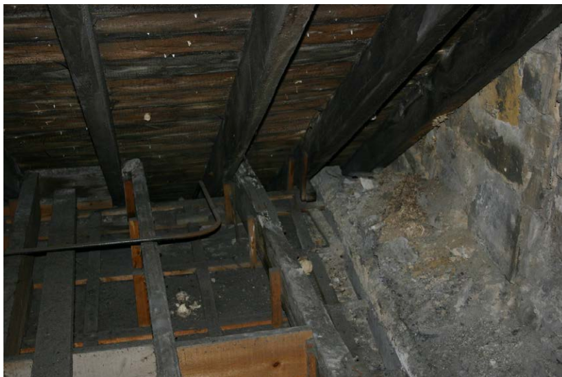
Fig. 128-66 View from north showing southern rafter of truss 49 (first rafter from right).
