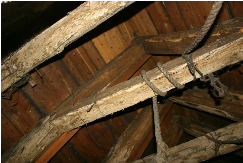
Fig. 130-2 View from north showing rafters 065 and 067, auxiliary rafter 066 and collar-beam 068 of truss 2.
