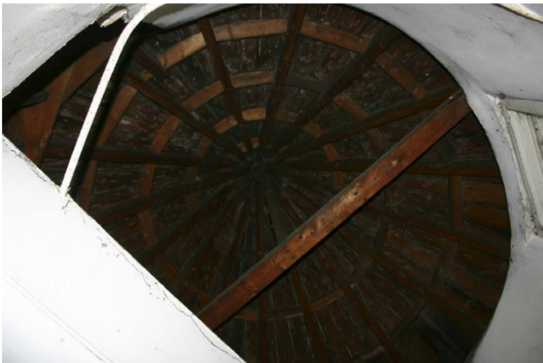
Fig. 136-9 View from north showing rafter 6 (sixth rafter underneath right part of collar-beam).
