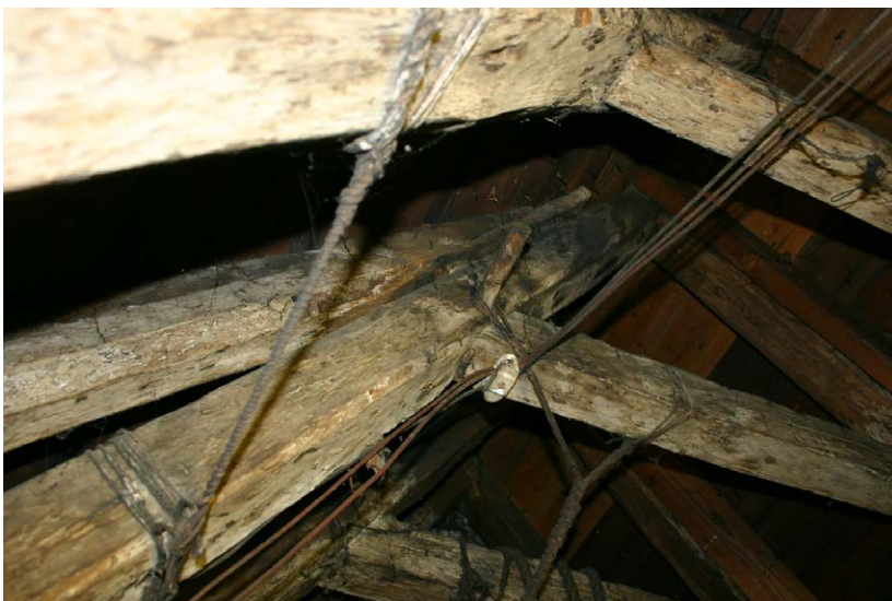
Fig. 130-26 View from east showing lean-to frame of truss 3 (second frame from top).
