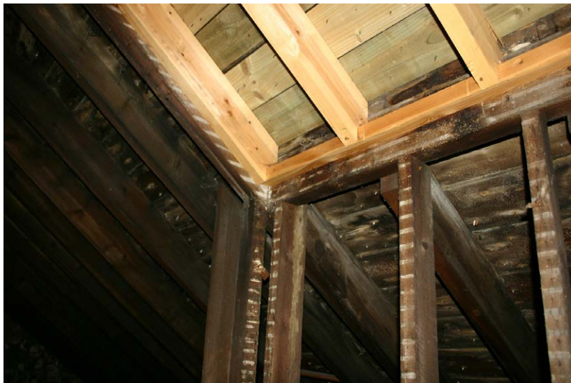
Fig. 128-14 View from northeast showing southern rafter (042) of truss 12 (second couple from west).
