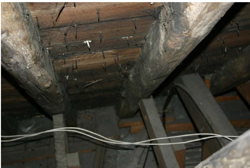
Fig. 130-27 View from east showing lean-to frame of truss 4 (second frame from left).
