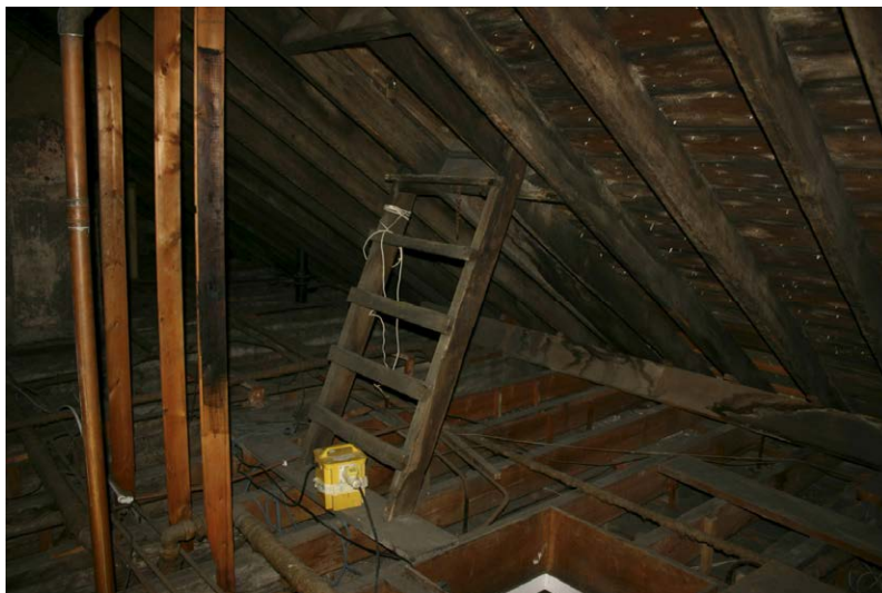
Fig. 128-39 View from east showing northern rafter (118) and collar-beam (120) of truss 28 (fourth couple from right).
