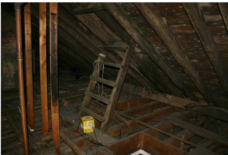
Fig. 128-42 View from south showing northern rafter (100) and northern collar-beam (101) of truss 31 (fifth couple from right).
