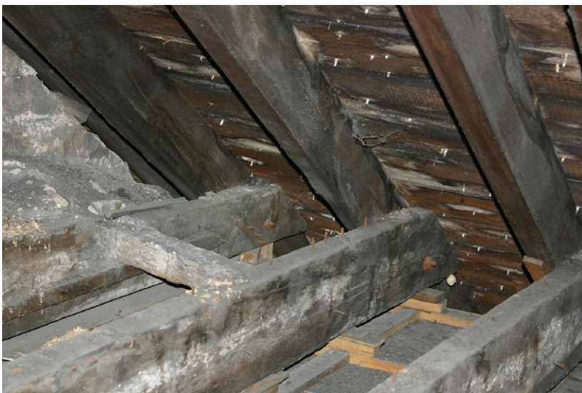
Fig. 128-4 View from northeast showing trimmer (011) between collar-beams (007 and 010) of trusses 2 and 3 (first two couples from left).
