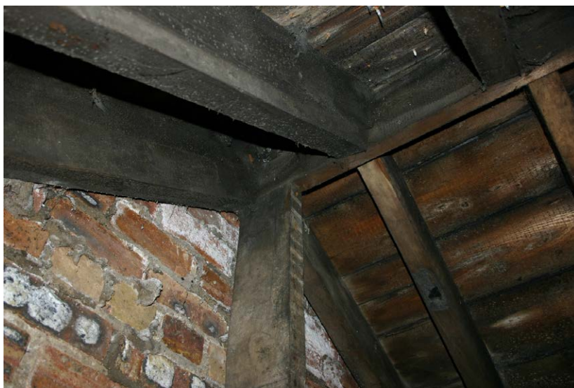
Fig. 128-65 View from southeast showing northern and southern rafters of truss 48 (first couple in front of wall).
