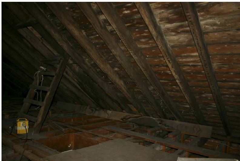
Fig. 128-40 View from south showing northern rafter (122) and collar-beam (123) of truss 29 (sixth couple from right).
