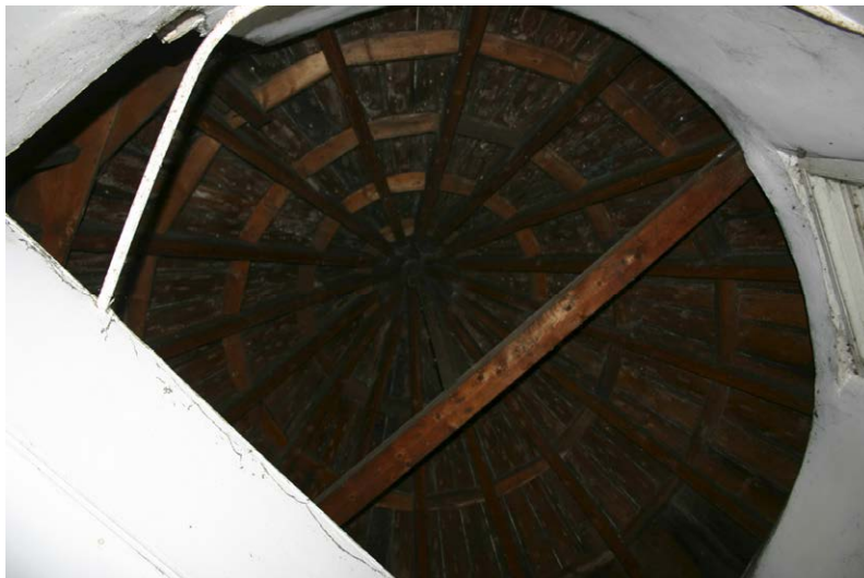
Fig. 136-8 View from north showing rafter 5 (fifth rafter underneath right part of collar-beam).
