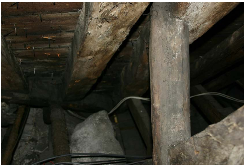
Fig. 130-29 View from east showing lean-to frame of truss 6 (second frame from left).
