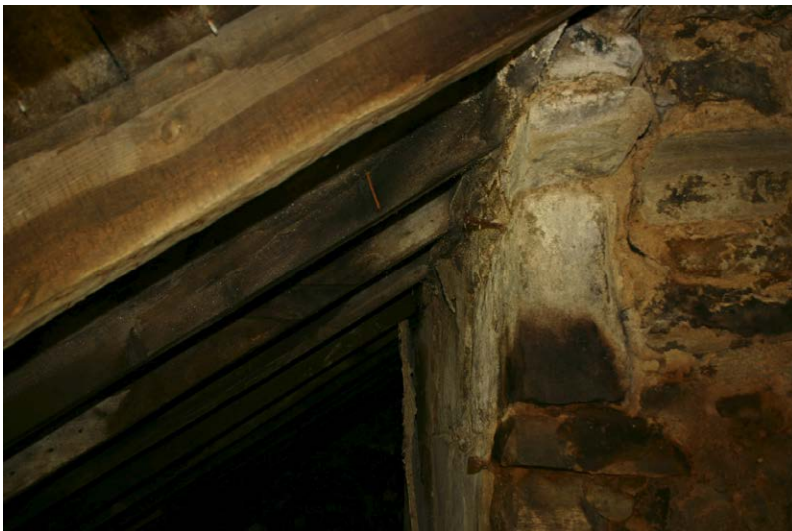
Fig. 128-25 View from west showing northern rafter of truss 15 (first rafter from top).
