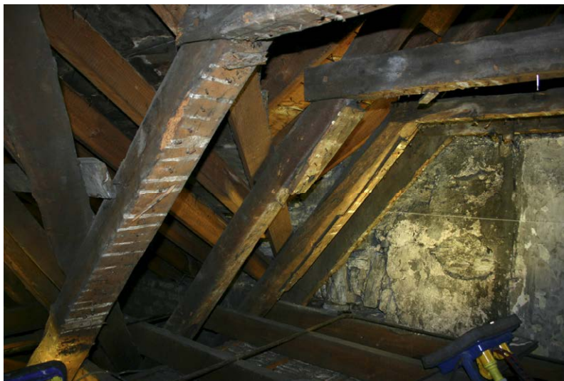
Fig. 131-4 View from west showing upper and middle collar-beams (070 and 071) and southern rafter (067) of truss 3.
