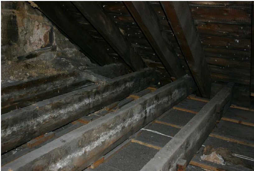
Fig. 128-5 View from northeast showing collar-beam (014) and southern rafter (013) of truss 4 (second couple from right).
