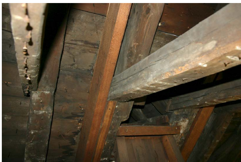
Fig. 131-14 View from north showing southern rafter (115), southern auxiliary rafters (118 and 119) and upper collar-beam (117) of truss 10.
