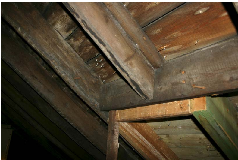
Fig. 128-10 View from southeast showing northern rafter (029) of truss 9 (first rafter from right).
