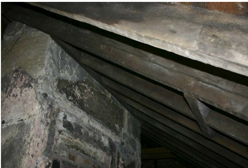
Fig. 128-50 View from east showing northern rafter of truss 38N (fifth couple from top).
