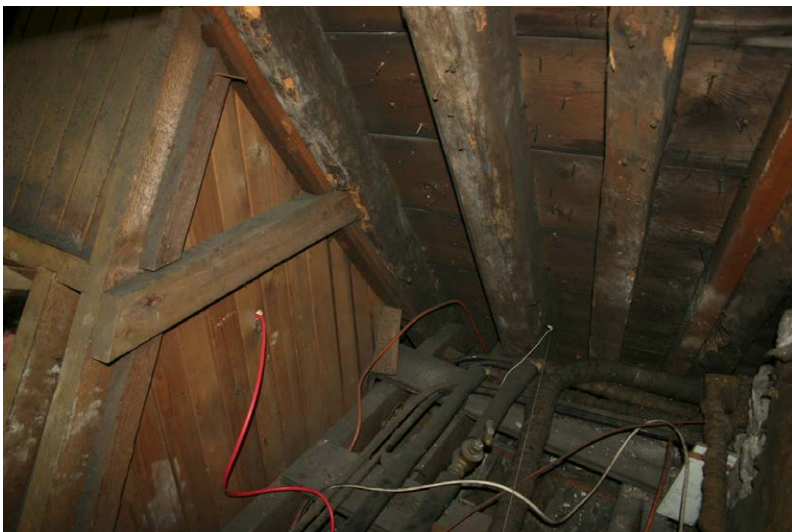
Fig. 131-16 View from northwest showing the eastern wall of n-dormer with sloping posts (125 and 126) and ledger (127).
