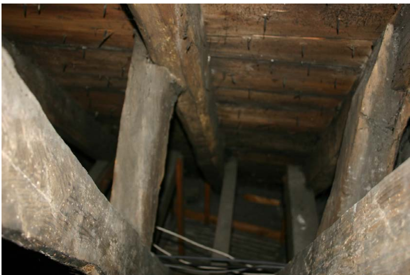
Fig. 130-25 View from east showing lean-to frame of truss 2 (first frame from right).
