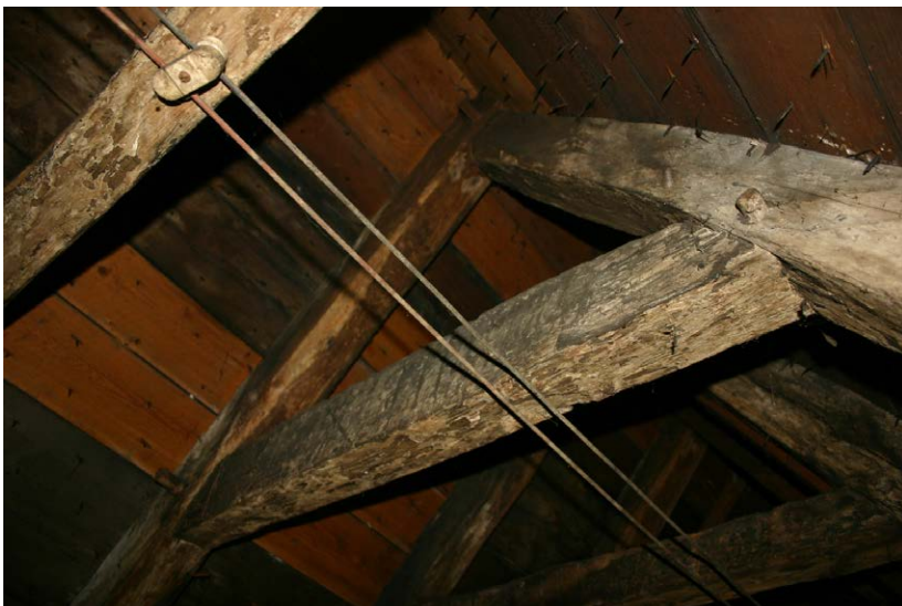
Fig. 130-14 View from southeast showing upper collar-beam (154) and eastern and western rafters (152 and 153) of truss 14.
