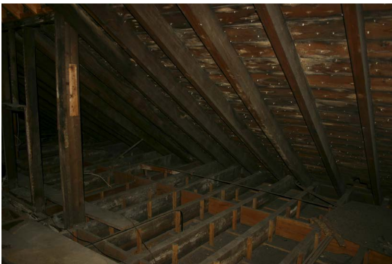
Fig. 128-17 View from north showing collar-beam (049) and southern rafter (048) of truss 15 (sixth couple from right)
