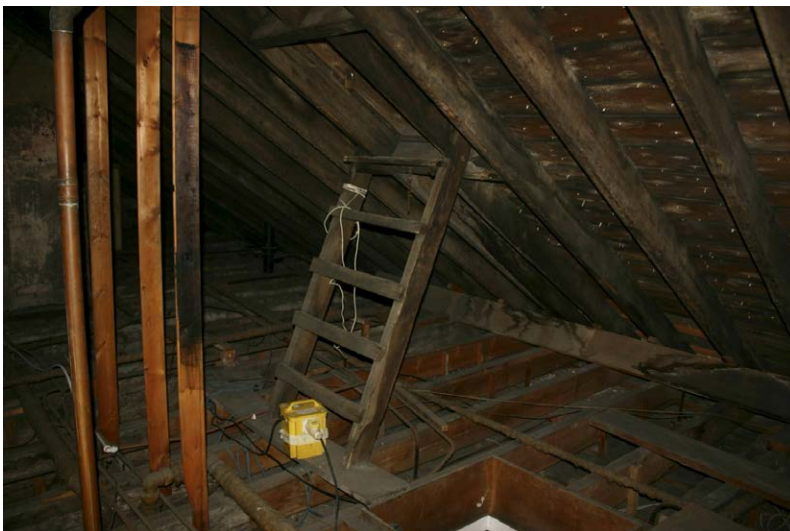
Fig. 128-41 View from south showing northern rafter (126) and northern collar-beam (128) of truss 30 (eight couple from right).
