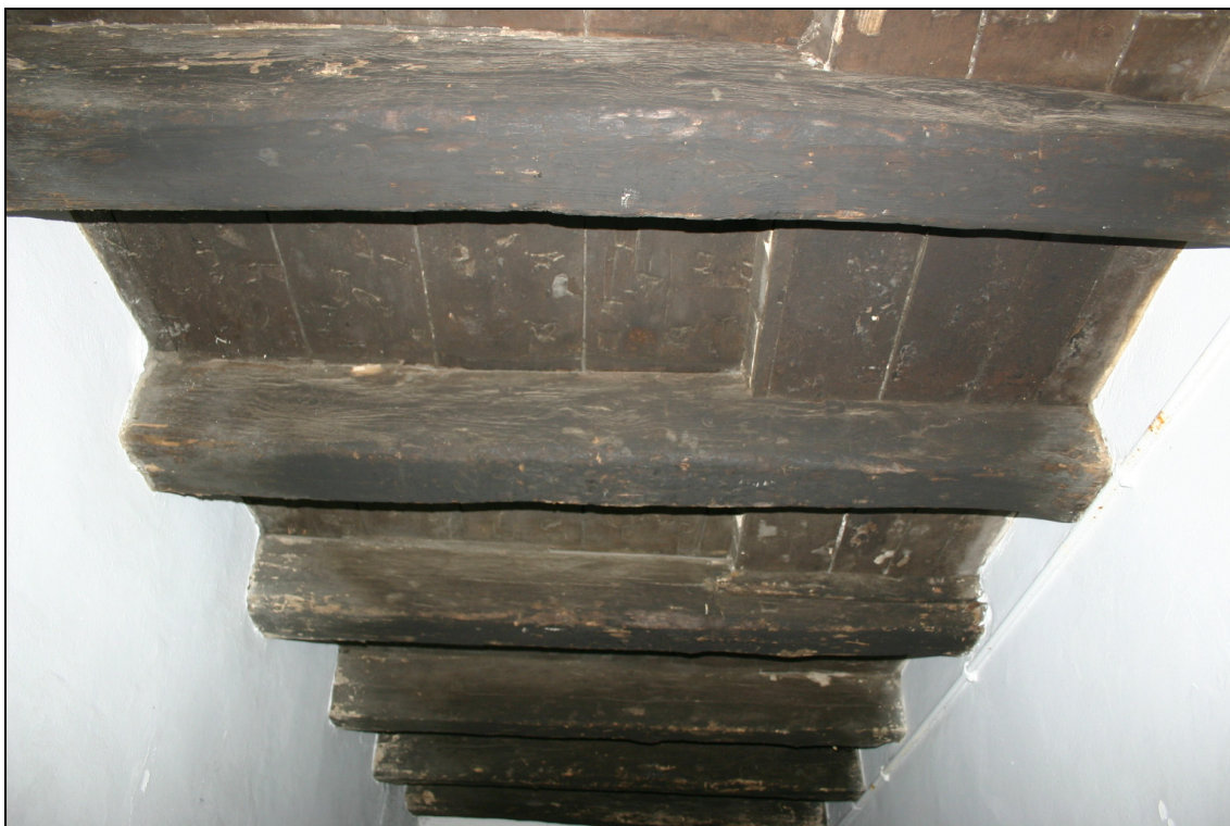
Figure A1-1: Ceiling over the southern part of the Pend. The joists consist of high quality oak and it is very likely that they could be dated dendrochronologically. This would establish a construction-date for the southern part of the main block.
