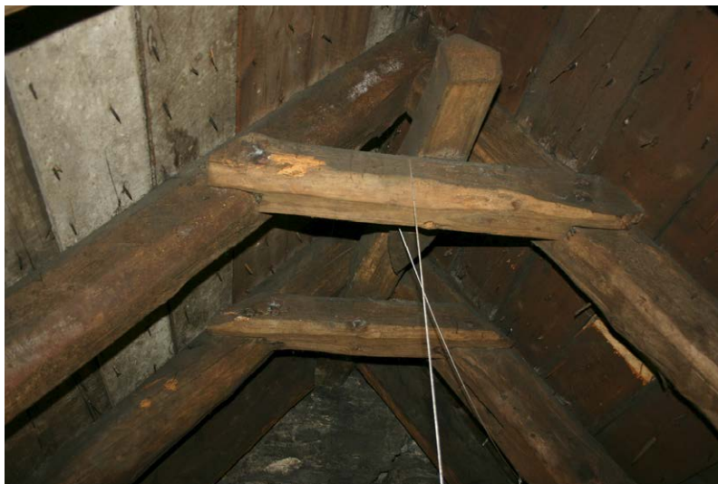
Fig. 131-2 View from east showing upper collar-beam (062) and southern and northern rafters (058 and 059) of truss 2.
