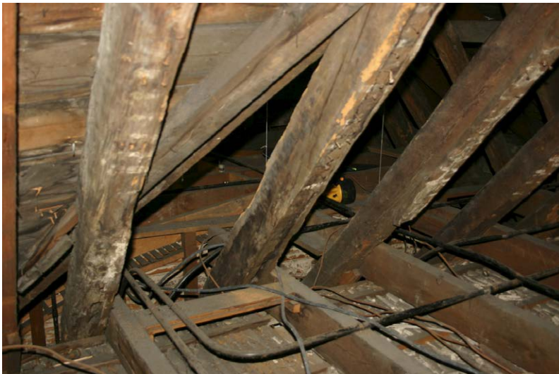
Fig. 131-9 View from east showing board 092 nailed to collar-beams (085 and 091) of trusses 5 and 6.
