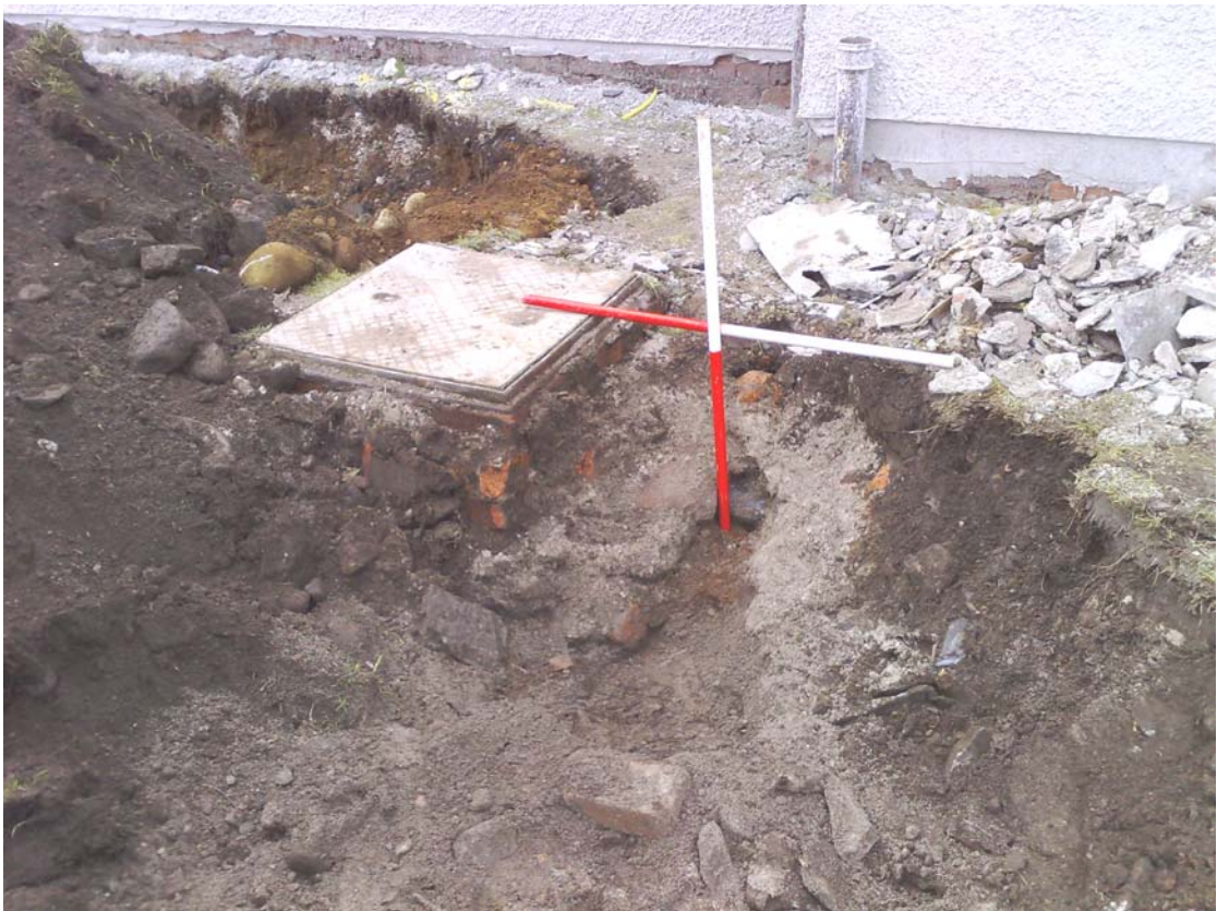
Plate 4: Looking WSW at the manhole with cast iron pipe below and to the right.
