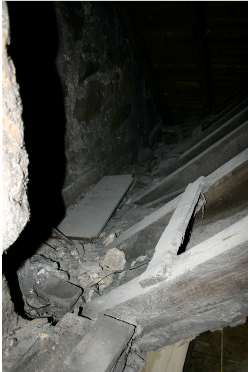
Figure 9: The roof (late C17), chimney (probably c.1538) and N wall (probably c.1538) of U20 at attic level.
