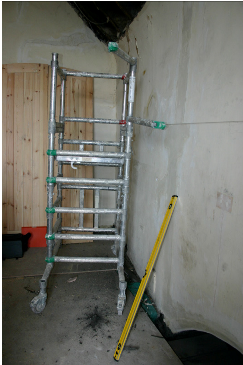
Figure 7: The roof (late C17), ceiling (late C17) and relieving arch (probably c.1538) in U20.
