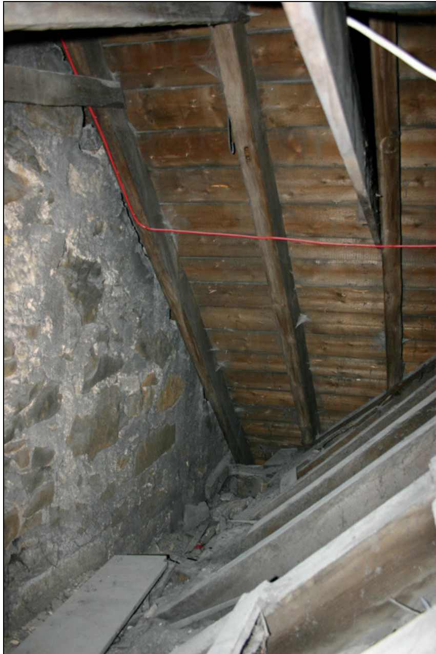
Figure 11: The N wall (probably c.1538), roof R05 (post-C17) and roof R10 (late C17) in U20.
