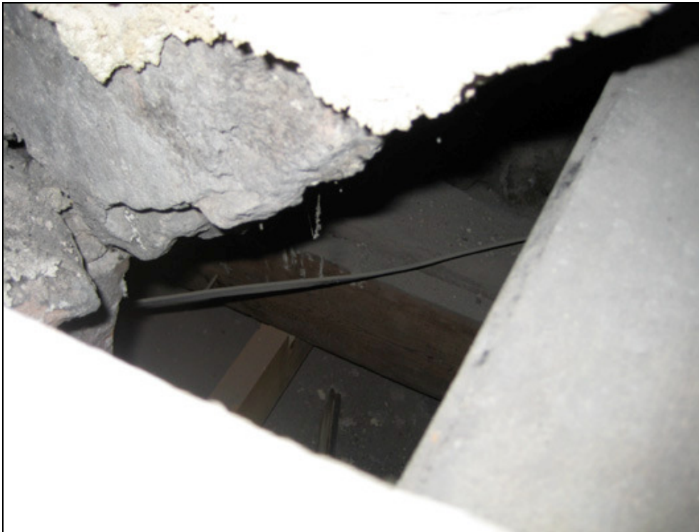
Figure 8: The relieving arch (probably c.1538) and floor joist (1538d) at the N wall of U20. The arch relates to the northernmost floor joist of the Queen's Bedchamber. This suggests that the arch was created in the context of the 1538 building operations.
