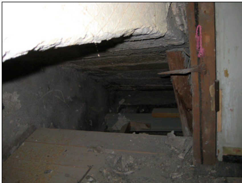
Figure 14: The western part of the relieving arch in U19, U21 and U22 (probably c.1538).
