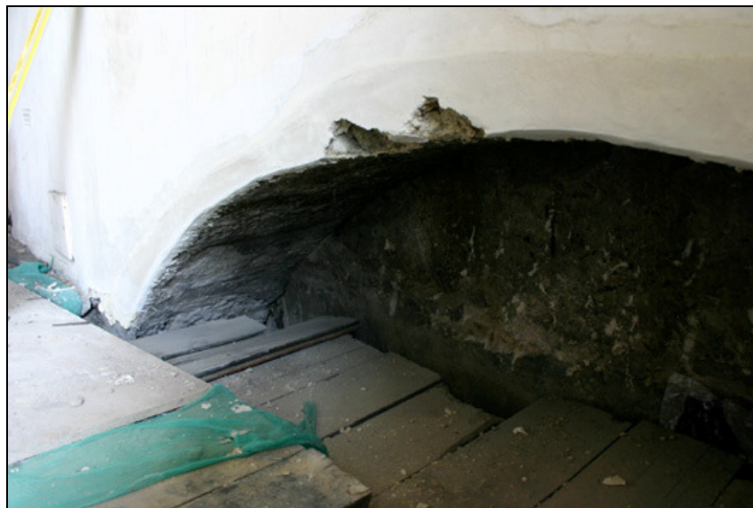
Figure 4: The western part of the relieving arch in U20 (probably c.1538). The arch is butted against rising rubble masonry which apparently belongs to the cross-wall that divides the Queen's Bedchamber and the King's Bedchamber. It is, without embarking on further research, impossible to say whether the rubble wall pre-dates or post-dates the arch.
