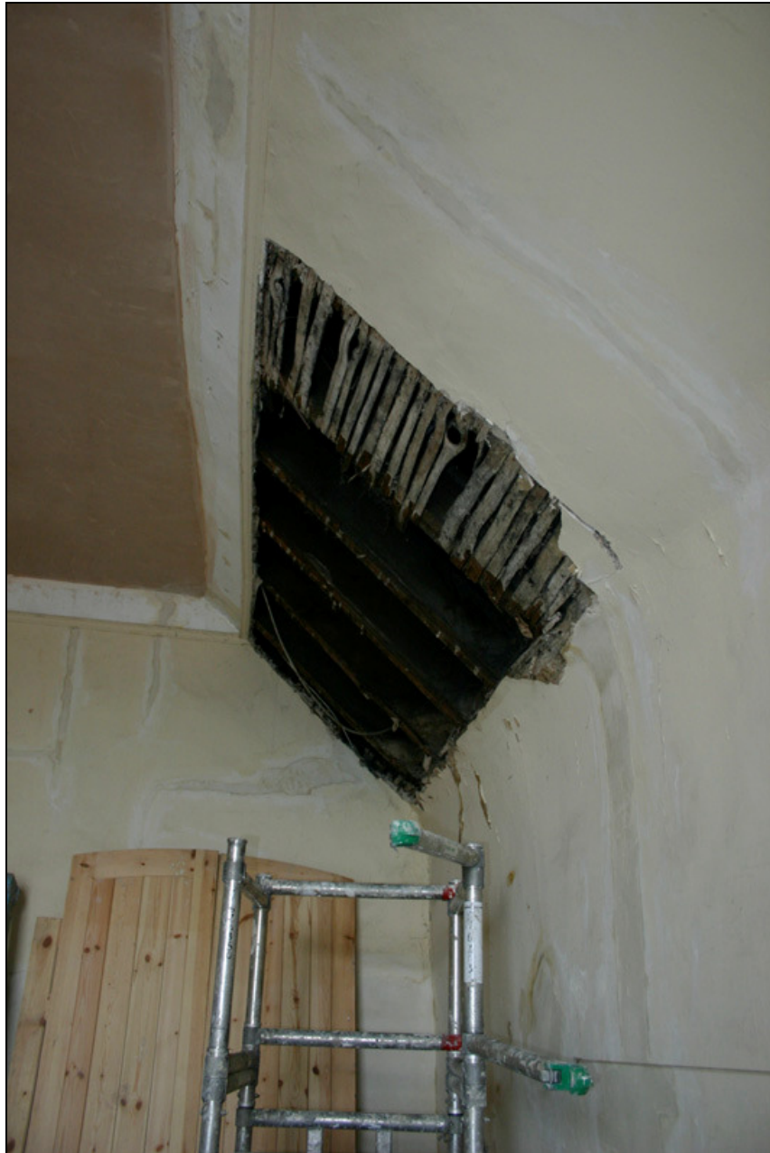
Figure 6: The roof (late C17) and lath and plaster ceiling (late C17) over U20 .
