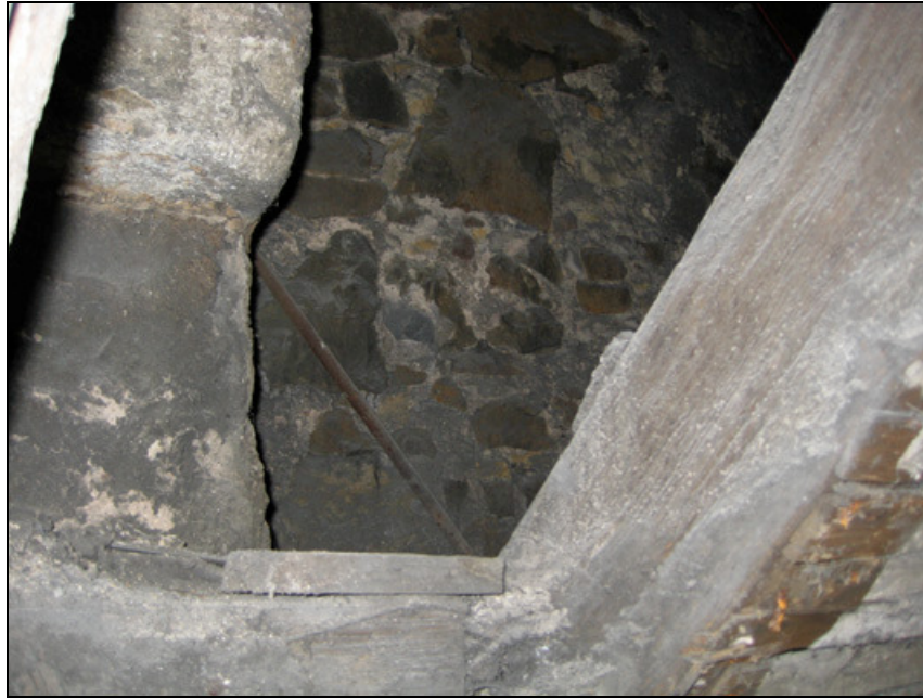
Figure 10: The chimney (probably c.1538), N wall of U20 (probably c.1538) and rafter of R10 (late C17). The chimney, datable in all probability to the years around 1538, possess a notch that appears more or less at current wall-head level. This notch may belong to the original roof over the SE-corner of Stirling Palace. The rubble wall over U20 at attic level may also belong to that period because it is highly unlikely that Stirling Palace originally possessed hip-and valley rafters. Instead it was common practice to butt the roof slabs against extended gable walls. The notch at the chimney may have been used for receiving lead-clad timbers employed for waterproofing the valley between the rafter feet and the rising wall.
